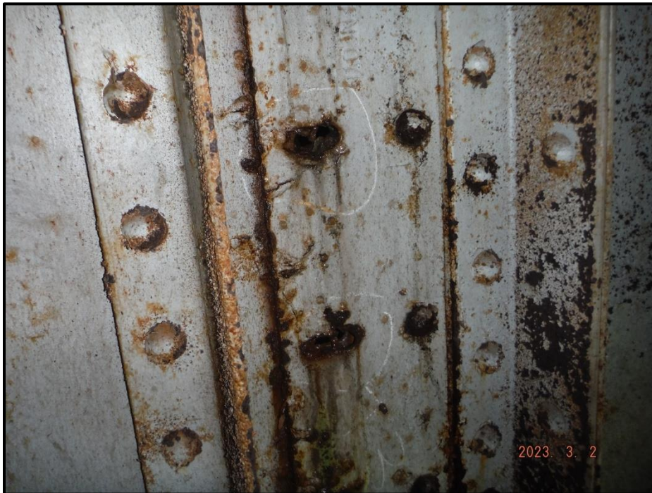
Photograph 34. Bent 3, Bay 1, Girder 2, web sliding plate, looking west. (3) missing bolts with heavy laminar corrosion, CS3.
