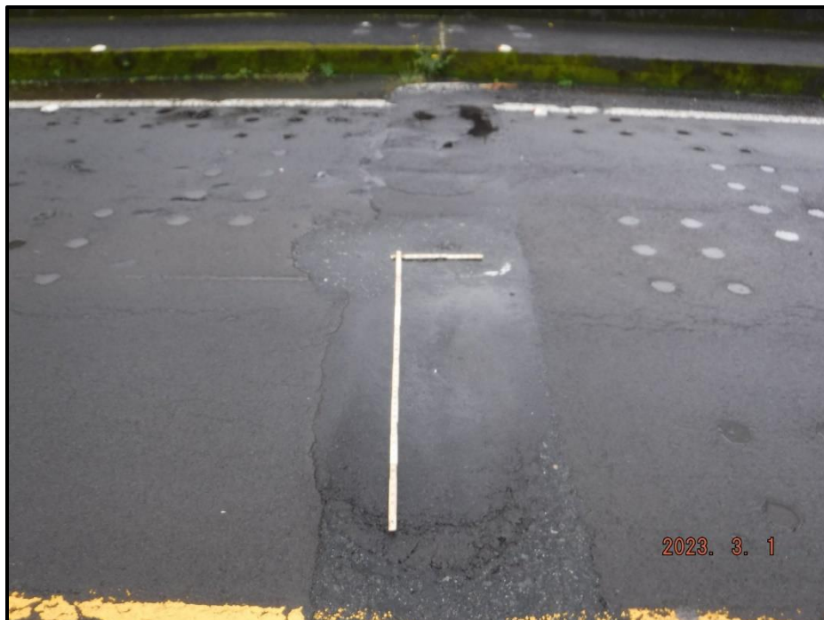
Photograph 16. Bent 3 Joint, both lanes, looking west. 2' 4" L x 4' W area of settled patches with a 6" Dia. x 1" D spall within. The rest of the paved over joint is rutted up to 1" deep, CS3
