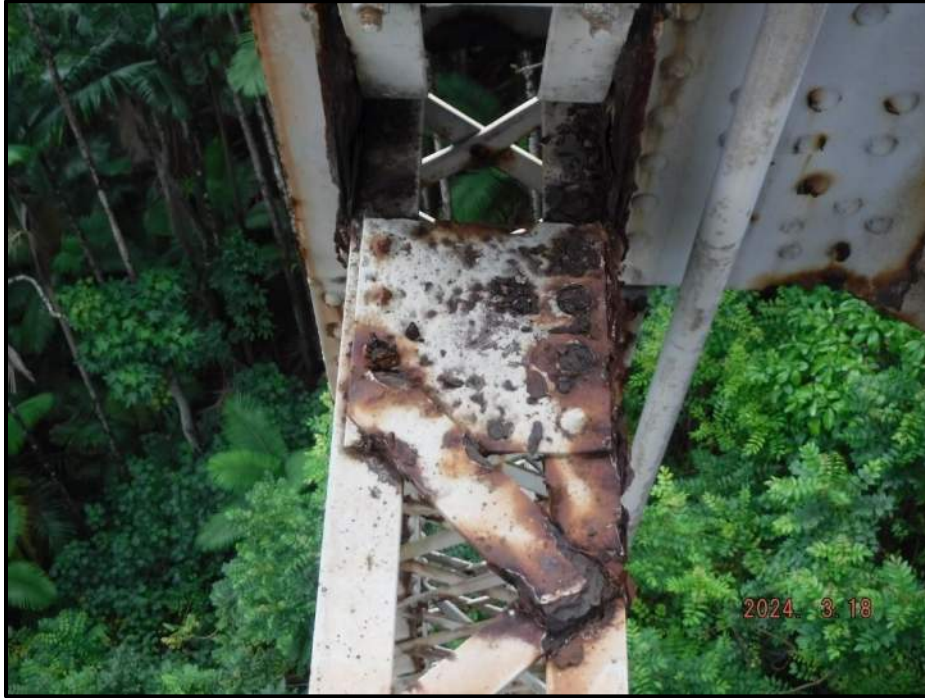
Photograph 39. Bent 3, Level 1, lower section, Columns A and B, horizontal bracing, looking east. Pack rust up to 1-1/2" thick with section loss up to 30% to gusset plates and 100% loss to rivet heads of batten plate, CS3.
