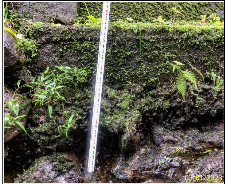
Photo 10. Bent 5, Column B footing, looking south. Exposure with grouted rocks exposed below, up to 1.4' H and a bottom rock layer of 1.6' H
