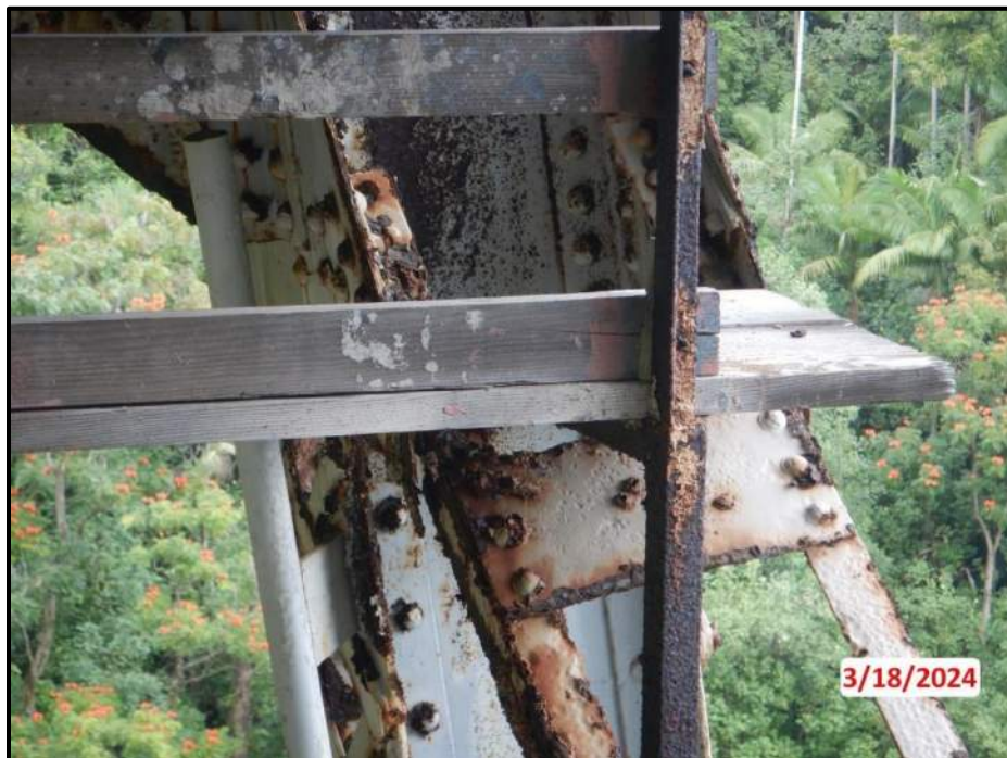
Photograph 22. Tower 2, Level 1, Column A , upper north diagonal bracing, near Bent 3, looking north. Vertical leg of interior angle near Column A connection, 6" L x 2" H corrosion hole. Exterior leg has area of pack rust causing separation of gusset plate up to 1". Rest of this member has multiple areas of knife-edging along interior angle over 8' length with individual areas up to 1" x 6" exhibiting 100% section loss, CS3.
