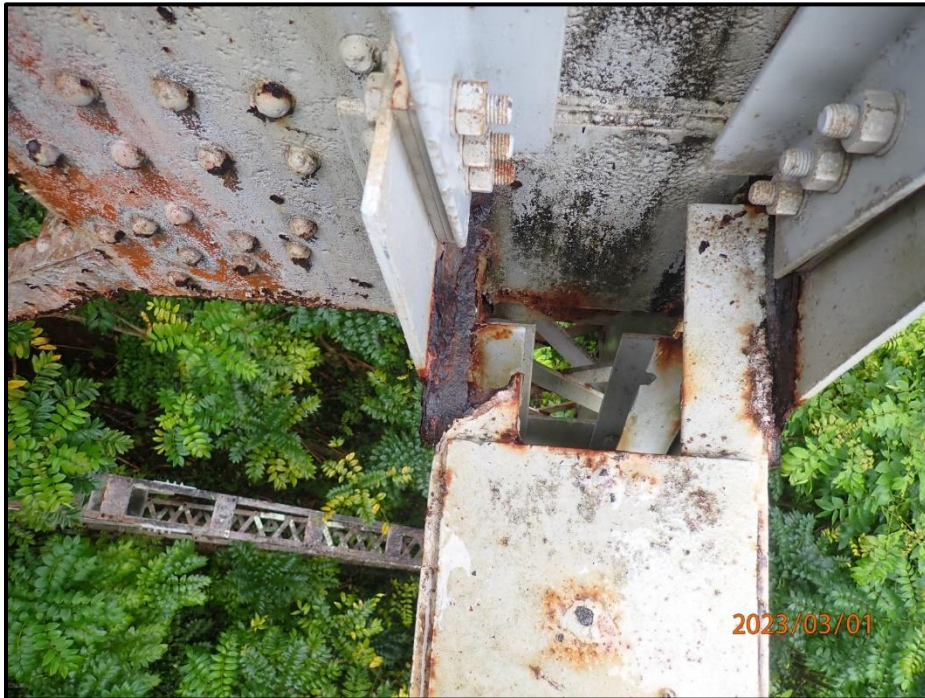
Photograph 79. Bent 3, Level 2, Column B, horizontal bracing, south flange, looking north. 9" L x full width of angle area of 100% section loss, CS3.
