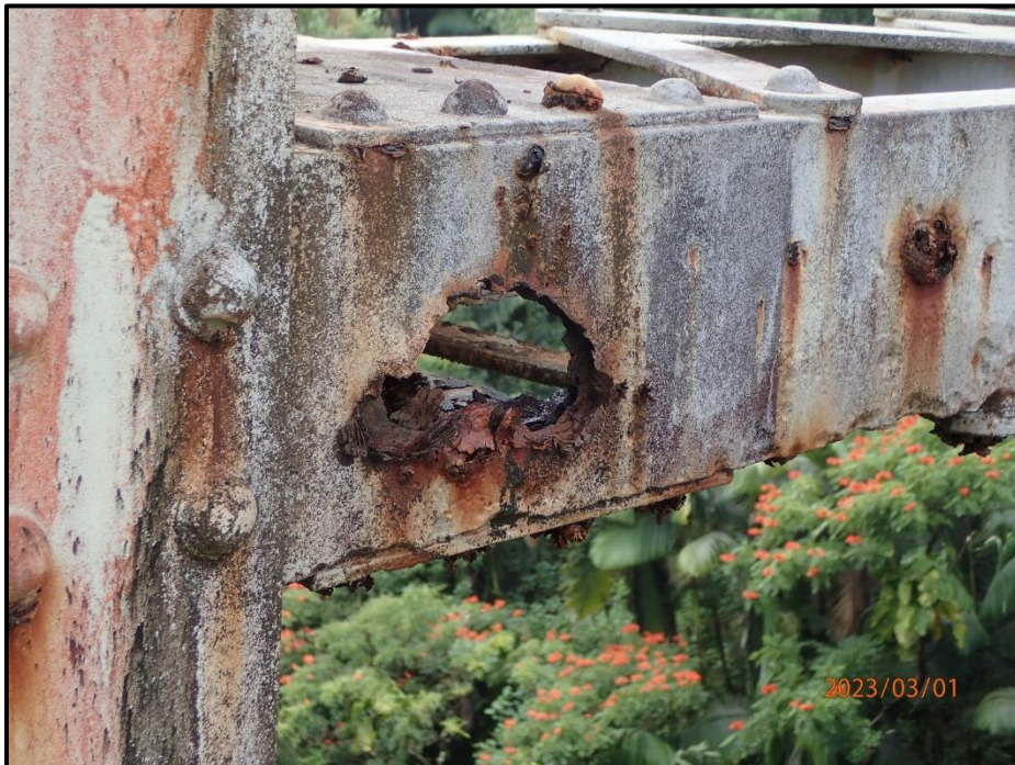
Photograph 102. Tower 3, Level 2, Column C, horizontal bracing, east channel, looking west. 8" L x 2" H corrosion hole, CS3.
