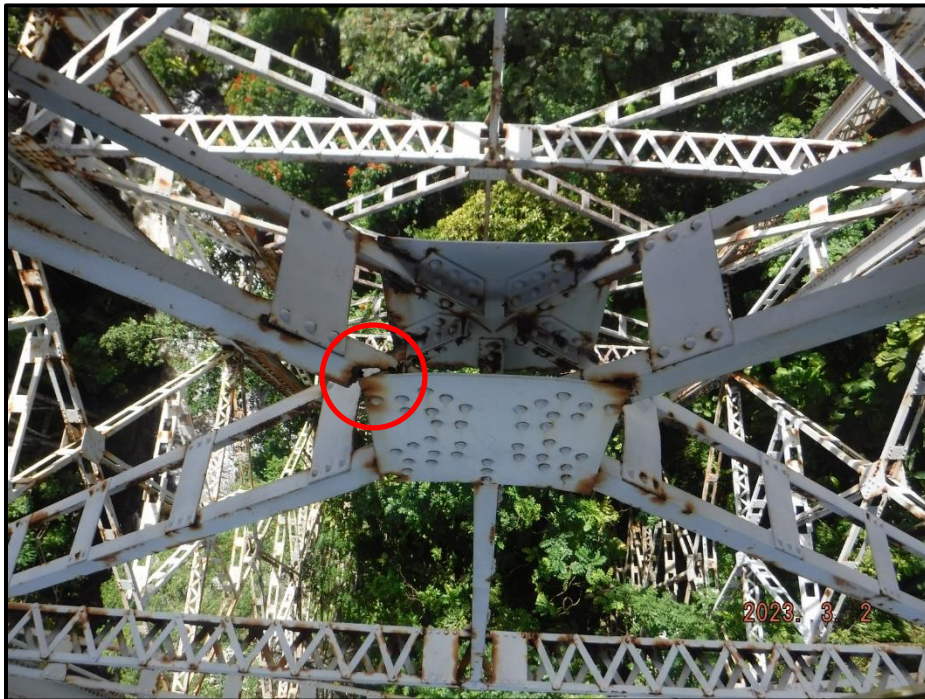
Photograph 133. Tower 4, Level 1, lower south diagonal bracing, looking west. Exterior angle of diagonal has 100% section loss to vertical leg and only 2 1/2" of section remaining on horizontal leg; angle is deformed 1/4" over 10" near section loss, CS4.
