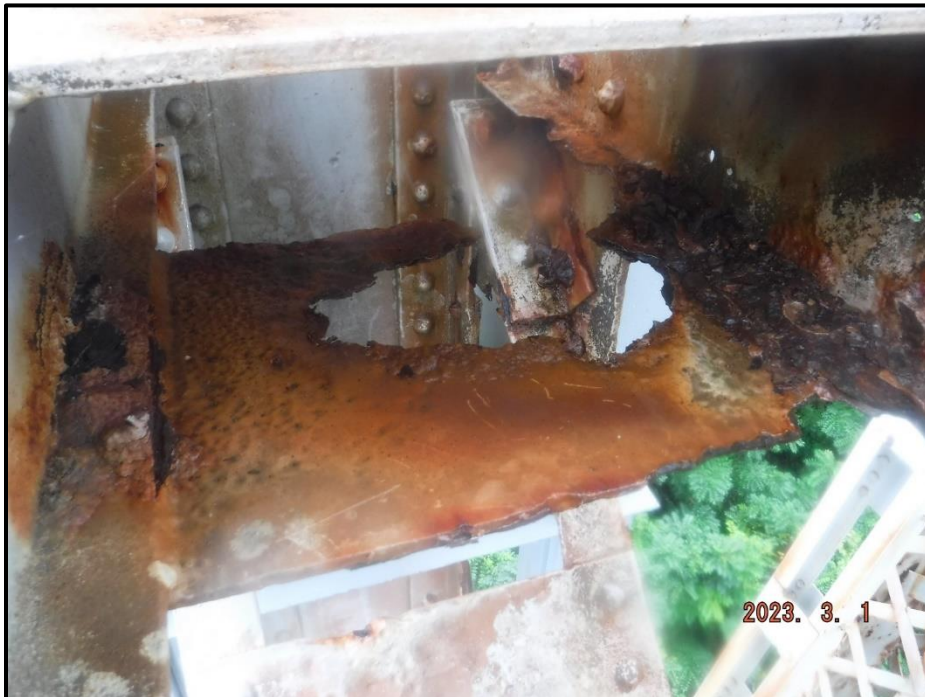
Photograph 94. Tower 3, Level 2, Column A, horizontal bracing, looking south. 9" diameter corrosion hole in lower batten plate with 3" W x 1/8" section remaining, CS3.
