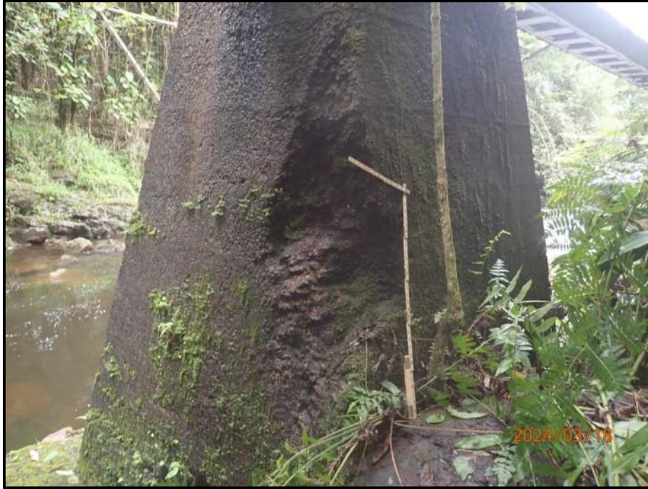
Photograph 83. Bent 5, Level 6, Column C, footing, southwest corner, looking east. Spall, 5' H x 1' 4" W x up to 10" deep, CS3.
