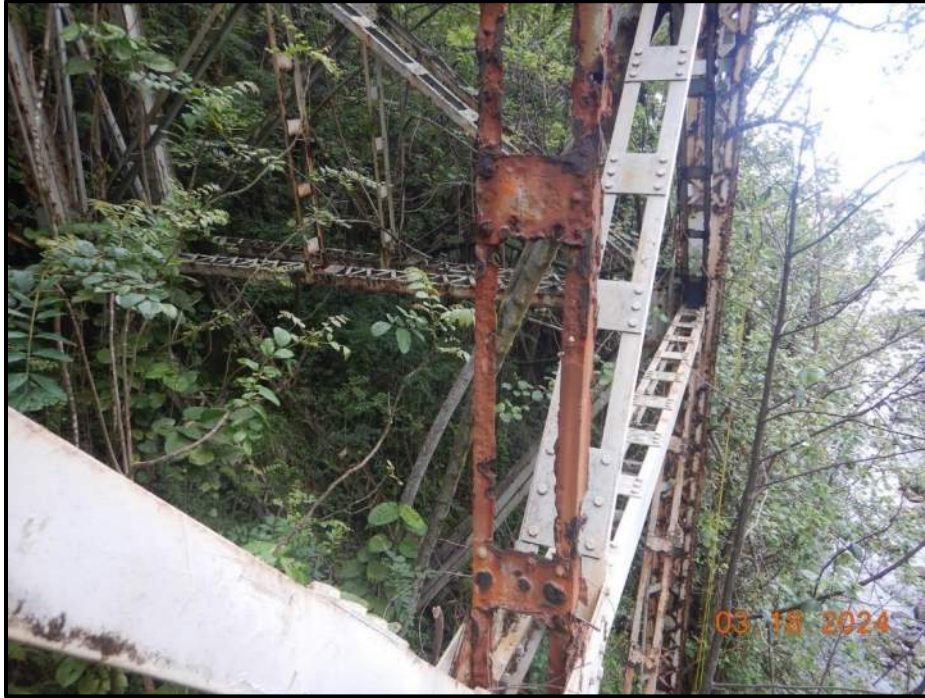
Photograph 91. Bent 6, Level 4, between Columns B and C, vertical bracing, looking east. Severe corrosion throughout this member with up to 60% cross sectional loss, CS4.
