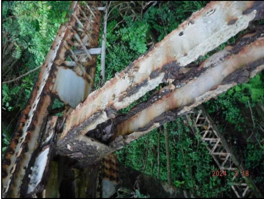
Photograph 95. Bent 6, Level 5, between Columns A and B, horizontal bracing web members, looking southeast. Up to 75% section loss throughout, CS4.
