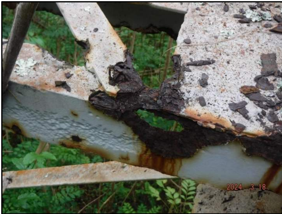
Photograph 18. Bent 2, Level 2, between Columns B and C, horizontal bracing near Column B, along flanges, looking north. Knife-edging with up to 1-1/2" L x 1" W corrosion holes, CS3.
