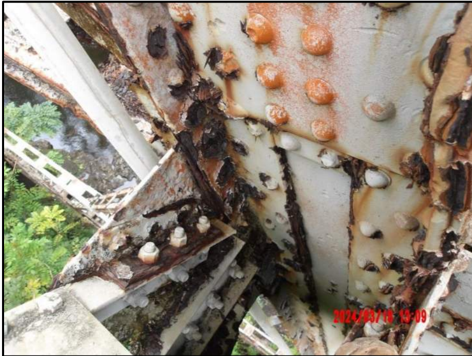
Photograph 80. Bent 5, Level 5, Column B interior splice plate rivets, looking northwest. Up to 100% section loss, corrosion, CS3.
