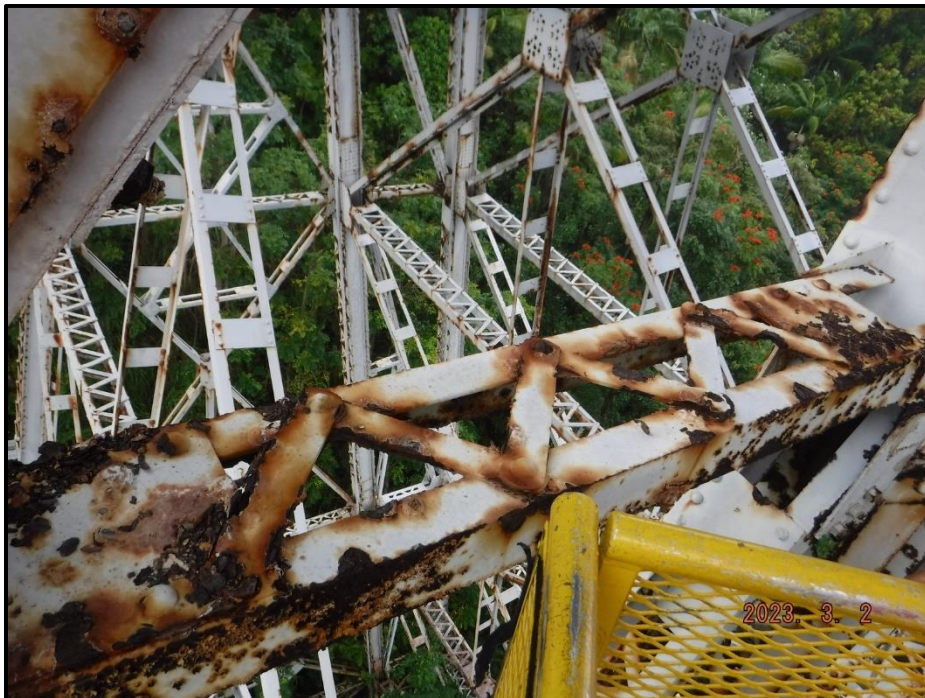
Photograph 119. Bent 6, Level 1, upper section, between Columns C and D, horizontal bracing, looking south. Heavy pitting with 1' 6" L x 2" H area of 100% section loss, CS3.
