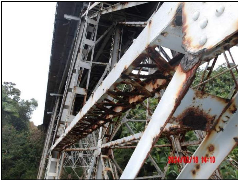
Photograph 58. Tower 3, Level 1, Column A, horizontal bracing, looking south. Heavy pitting and laminar corrosion with up to 80% section loss. Few lacing bars exhibit 100% section loss and knife-edging. Channel legs exhibit scattered knife-edging, CS3.
