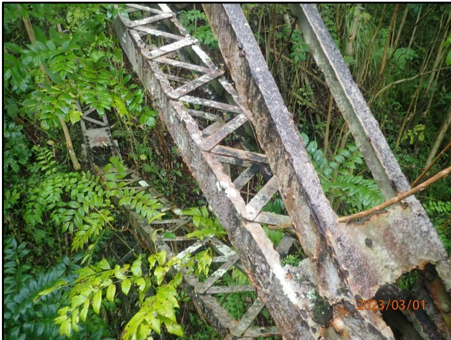
Photograph 70. Tower 2, Level 3, Column B, looking west. Multiple up to 3/4" diameter corrosion holes throughout, and covered in vegetation, CS3.
