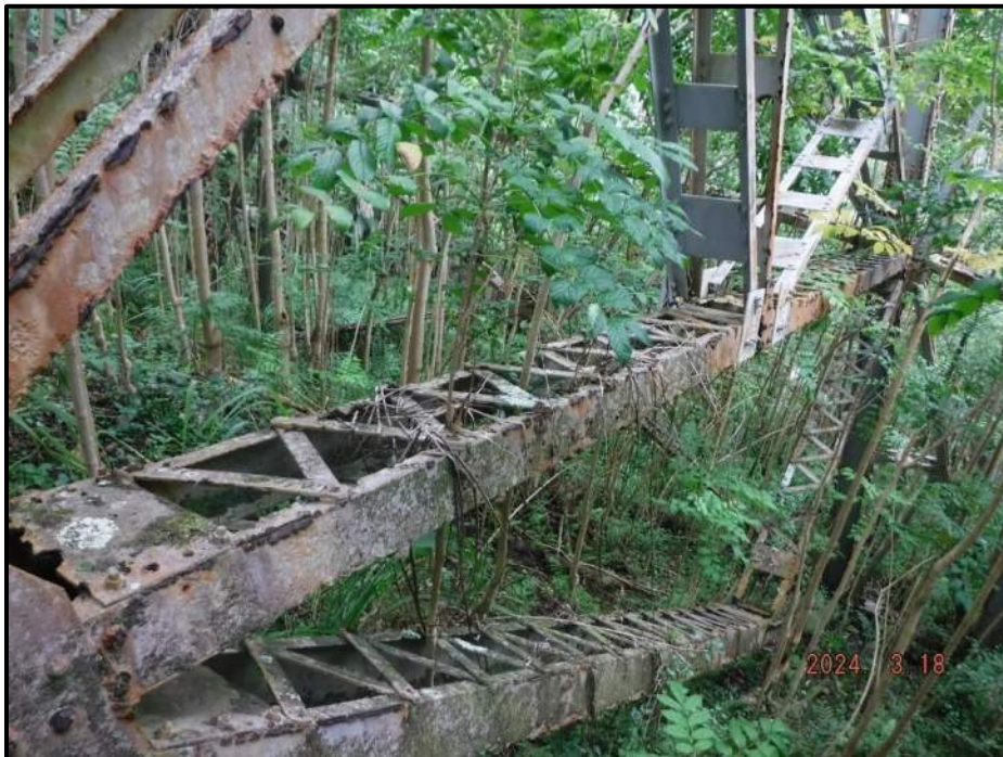
Photograph 26. Tower 2, Level 3, Column B, horizontal bracing, looking northwest. Multiple up to 3/4" diameter corrosion holes throughout, and covered in vegetation, CS3.
