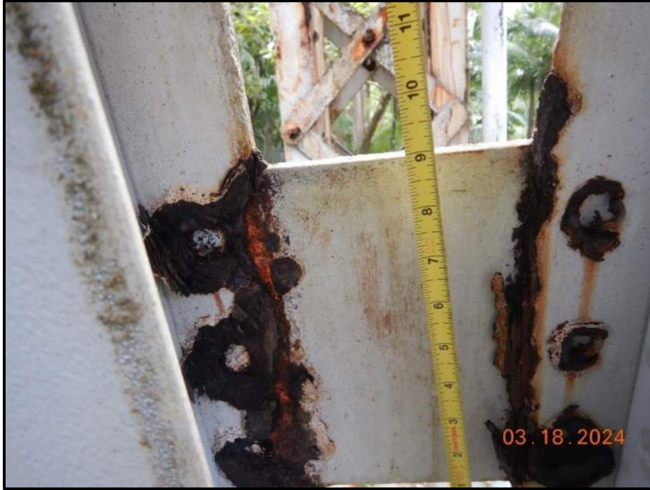
Photograph 17. Bent 2, Level 2, between Columns C and D, diagonal bracing, near short horizontal, batten plate, interior rivet heads, looking west. All have 100% section loss, CS3.
