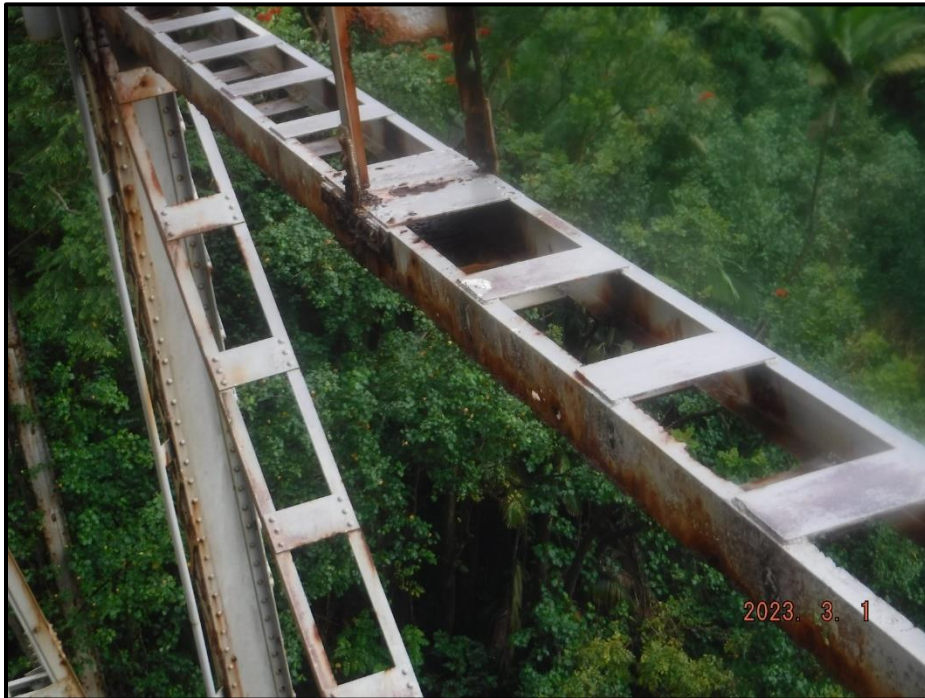
Photograph 95. Tower 3, Level 2, Column A, horizontal bracing, near Bent 4, looking northeast. 50% section loss to entire member with holes throughout, CS4.
