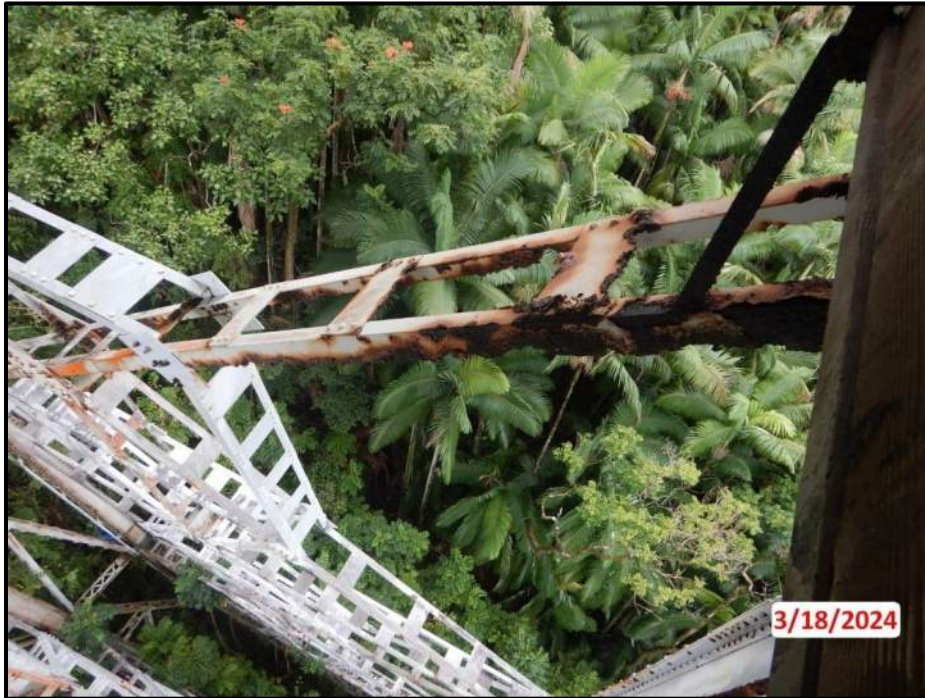
Photograph 30. Tower 2, Level 1, Column D, upper north diagonal bracing, looking west. Heavy knife-edging and up to 6" L x 2" H corrosion holes, CS3.
