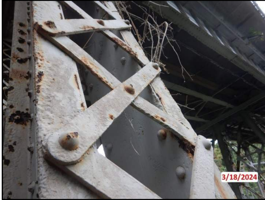
Photograph 9. Bent 1, Level 1, lower section, Column A, looking northwest. Typical pitting, pack rust and laminar corrosion, CS3.
