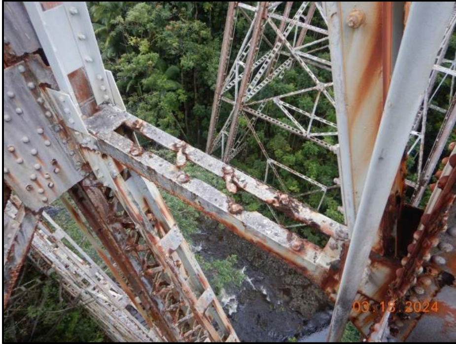
Photograph 87. Bent 6, Level 2, between Columns C and D, horizontal bracing, all (4) lacing bars, looking southeast. 100% section loss, CS3.
