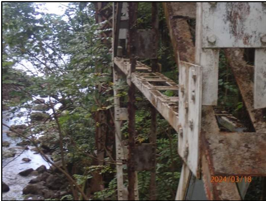
Photograph 82. Bent 5, Level 6, between Columns B and C, vertical bracing, looking east. Up to 25% section loss and pitting up to 1/8" deep, CS3.
