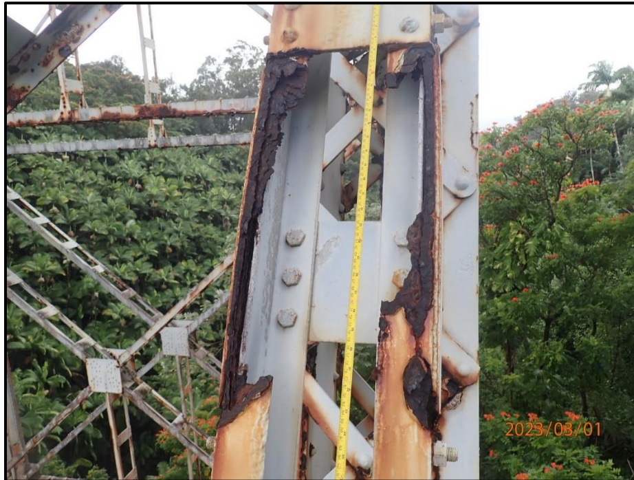
Photograph 146. Bent 7, Level 2, between Columns A and B, diagonal bracing top angle, looking west. Section loss, 100% loss for 2' 4" L, CS3.
