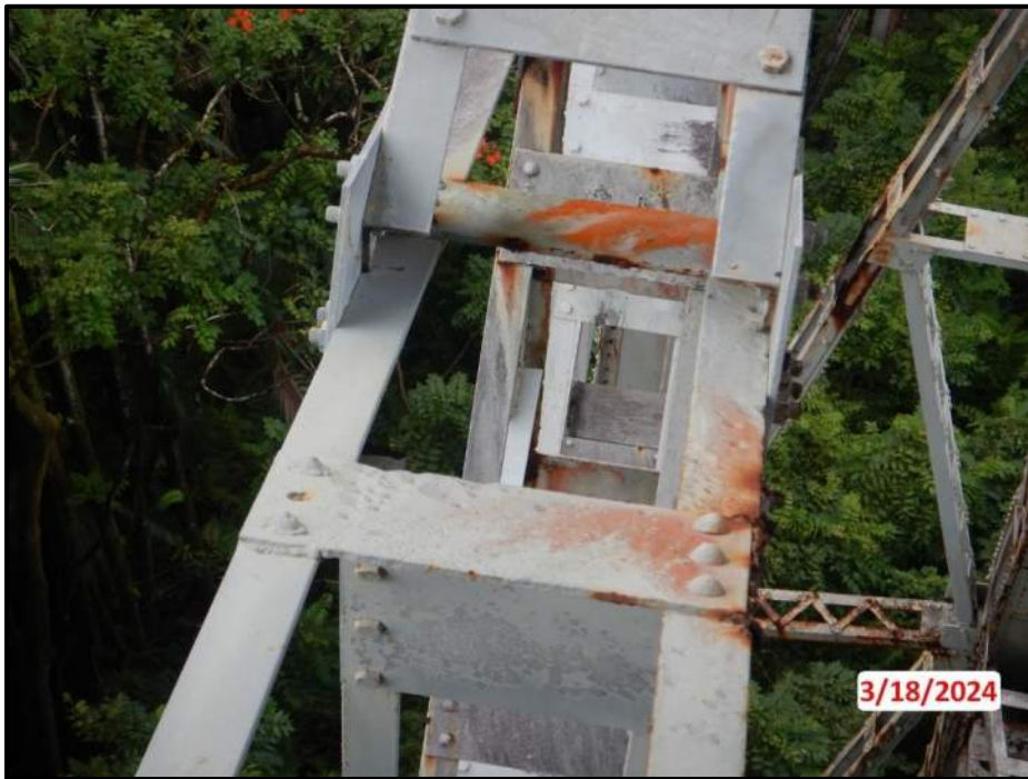
Photograph 28. Tower 2, Level 1, Column D, upper north diagonal bracing, top face of batten plate, west rivet heads, looking north. (1) of (3) missing, CS3.
