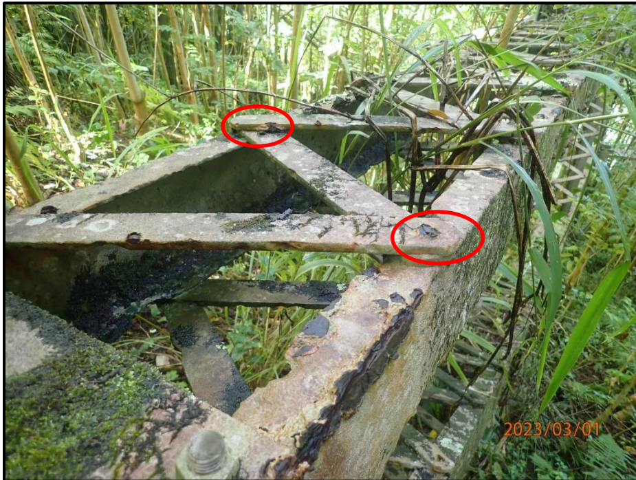
Photograph 69. Tower 2, Level 3, Column B, horizontal bracing, looking north. Numerous rivet heads in horizontal strut with up to 100% section loss, CS3.
