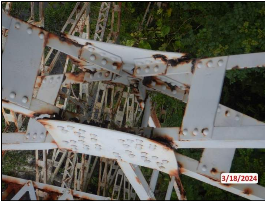
Photograph 102. Tower 4, Level 1, Column B, upper south diagonal bracing, looking west. Exterior angle of diagonal has 100% section loss to vertical leg and only 2" of section remaining on horizontal leg; angle is deformed 1/4" over 10" near section loss, CS4.
