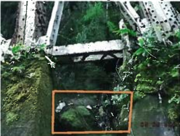
Picture of bent 6 with a bolder wedged between piers.
