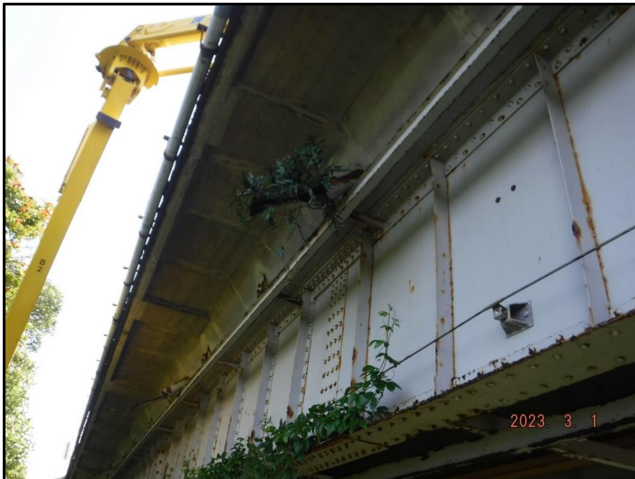
Photograph 14. Span 2, east overhang, 1st scupper south of Bent 2, looking west. Vegetation growth and almost full of debris.
