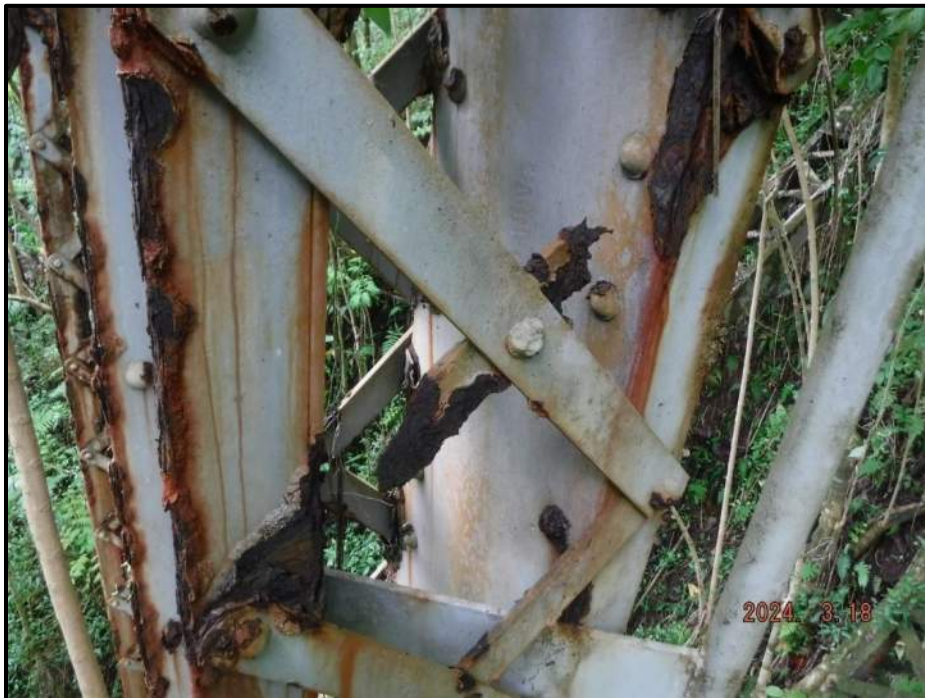
Photograph 44. Bent 3, Level 4, Column B, (1) lacing bar, looking east. 100% section loss on both ends on the west column face, CS3.
