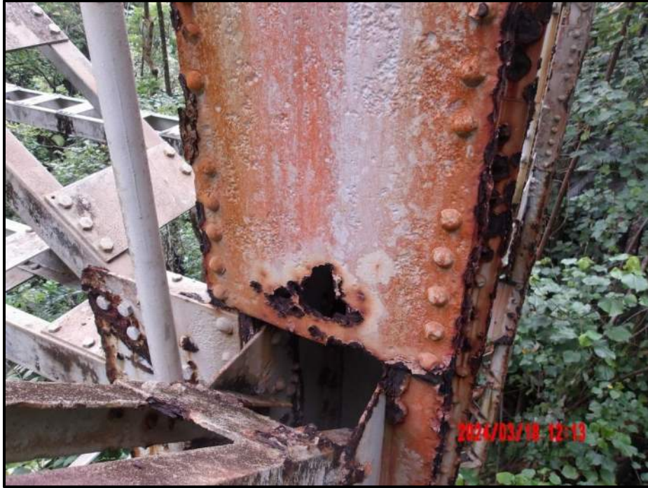
Photograph 53. Bent 4, Level 4, Column B, west face, cover plate, looking east. Corrosion hole, 8" W x 5" H, CS3.
