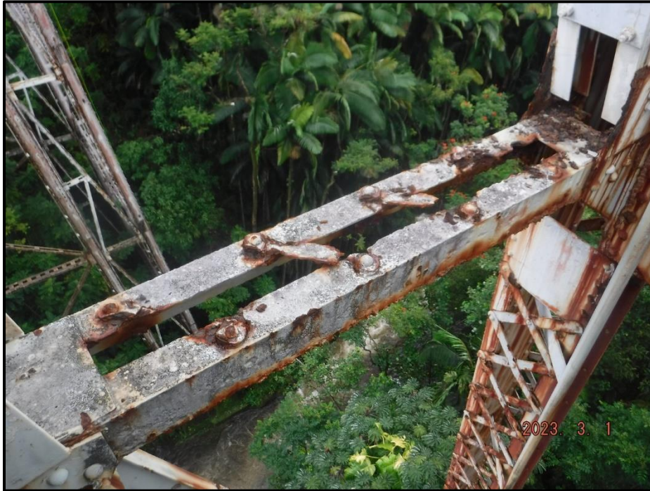
Photograph 124. Bent 6, Level 2, between Columns C and D, horizontal bracing, looking southwest. All (4) lacing bars have 100% section loss, CS3.
