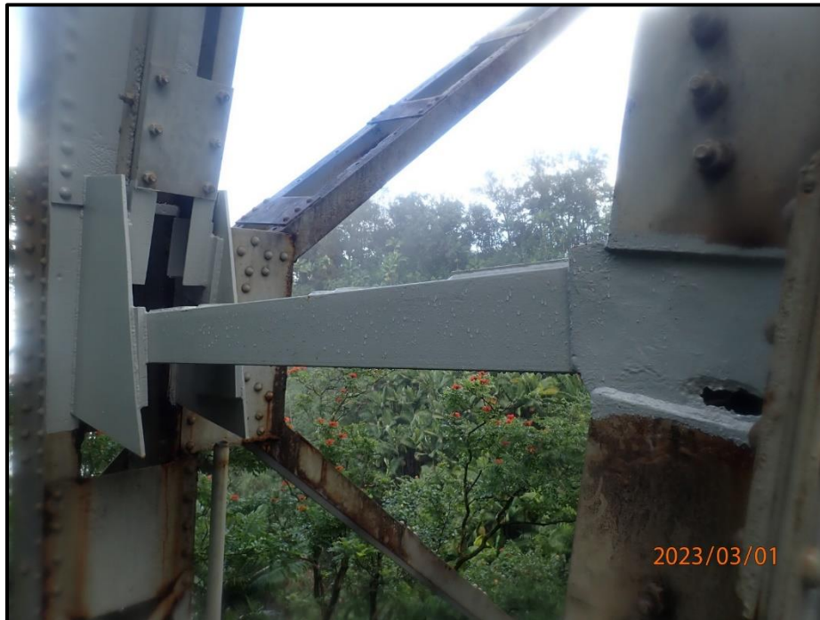
Photograph 147. Bent 7, Level 2, between Columns A and B, horizontal bracing and gusset plate at Column A, looking southeast. Previous detached bracing and gusset plate has been replaced.
