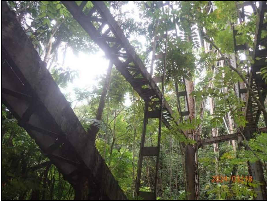
Photograph 69. Tower 3, Level 6, Column D, upper horizontal bracing, looking northwest. Vegetation, tree growing through members.
