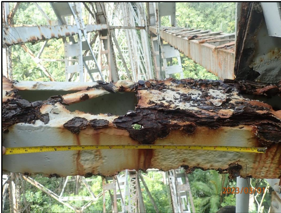
Photograph 60. Bent 2, Level 1, lower section, between Columns A and B, horizontal bracing, looking north. South face of angle has 1' 8" L x 1" H x up to 100% section loss with (3) lacing bars up to 75% section loss. The south angle has approximately 30% section loss
