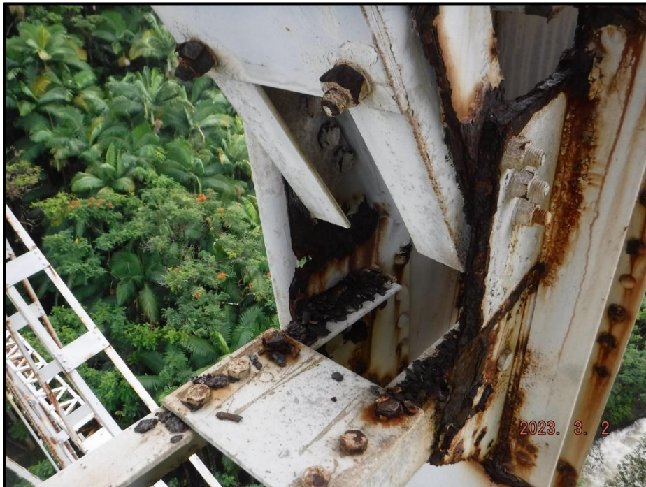
Photograph 106. Bent 5, Level 1, upper section, Column D, lower gusset plates, looking southwest. Heavy laminar corrosion with up to 100% section loss, CS3.
