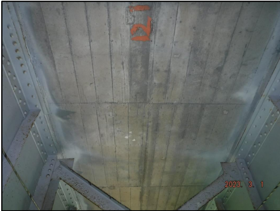
Photograph 25. Span 2, underside of deck, Bay 2, looking north. Map cracking throughout up to 1/16" W, CS3.
