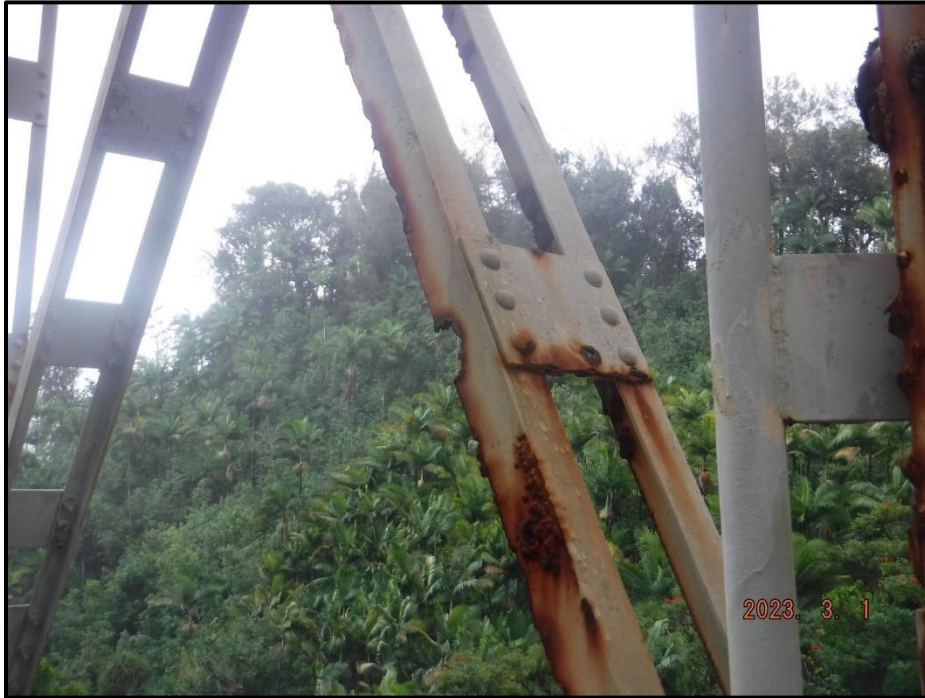
Photograph 122. Bent 6, Level 2, between Columns C and D, lower west diagonal bracing near Column D, looking southeast. 3" L x 2" H corrosion hole on north angle vertical leg, CS3.
