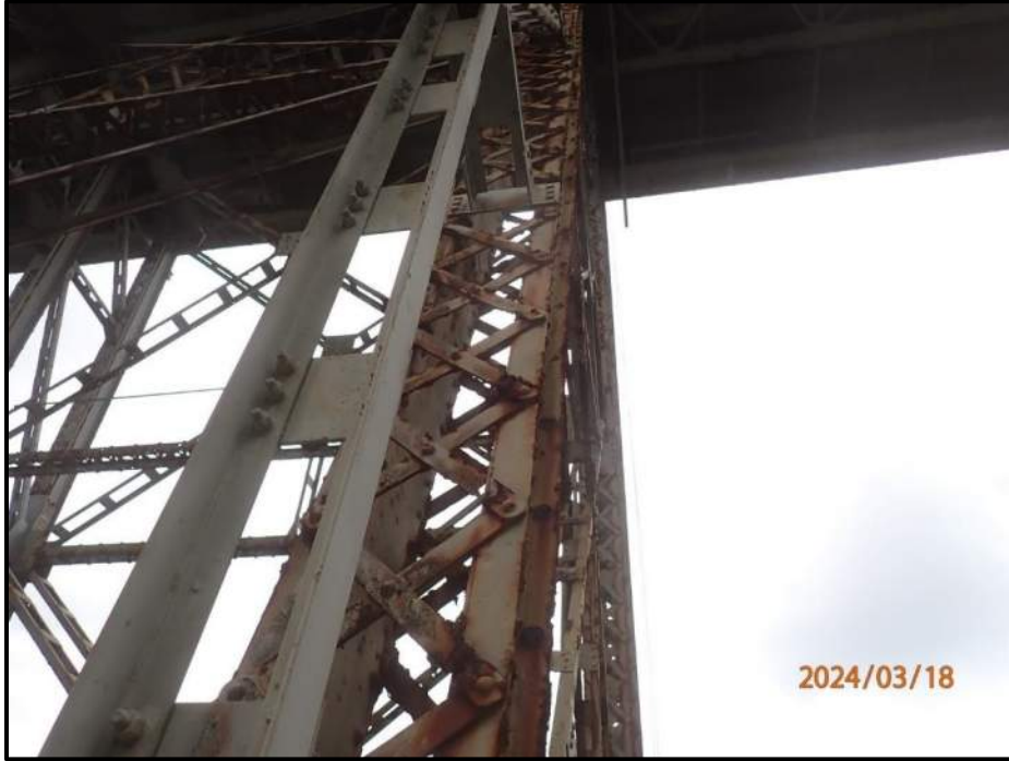
Photograph 49. Bent 4, Level 2, Column C, looking north. 50% of lacing bars on west face have 100% section loss, remaining bars on both faces have average 30% section loss, CS4.
