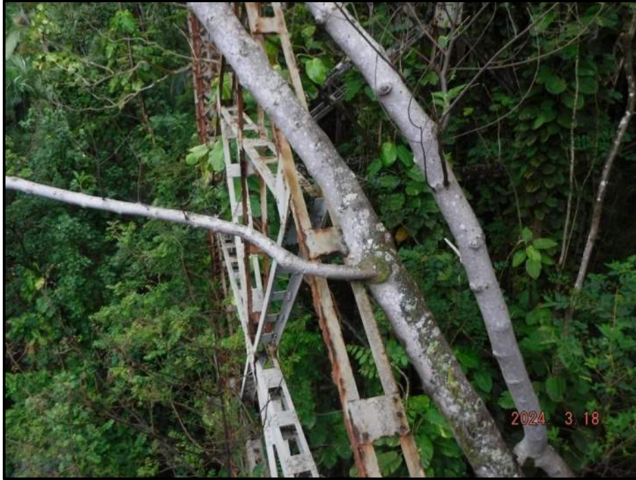
Photograph 93. Bent 6, Level 4, between Columns B and C, lower east diagonal bracing, looking west. Large tree leaning heavily on bracing, CS3.
