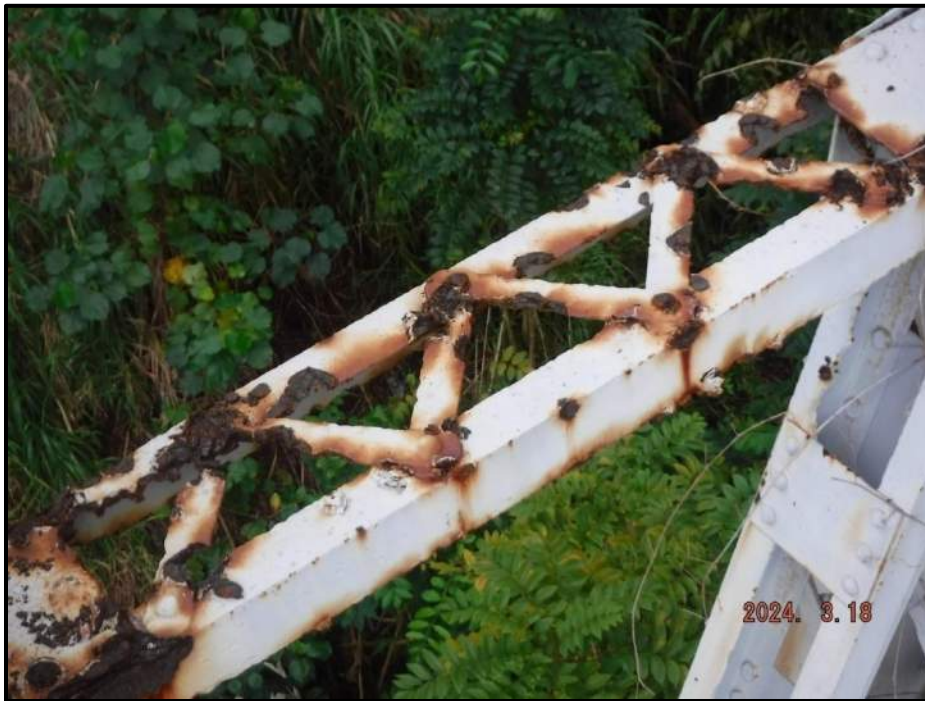
Photograph 14. Bent 2, Level 1, lower section, between Columns A and B, horizontal bracing, south face of angle, looking north. 1' 8" L x 1" H area of up to 100% section loss, with (3) lacing bars up to 75% section loss. The south angle has approximately 30% section loss near Column A. Angle original section is 3" x 4-1/2", remaining is 1-1/2" x 3-3/4", CS3.
