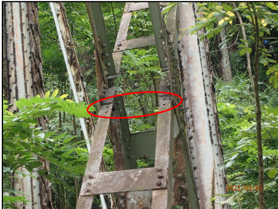
Photograph 104. Tower 3, Level 5, Column D, lower north diagonal bracing, at center gusset plate, looking south. Batten plates missing, CS3.
