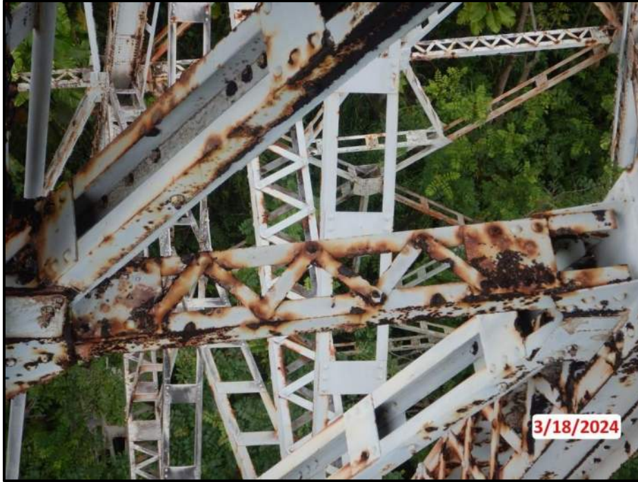
Photograph 85. Bent 6, Level 1, upper section, between Columns C and D, horizontal bracing, looking north. Heavy pitting with 1' 6" L x 2" H area of 100% section loss, CS3.
