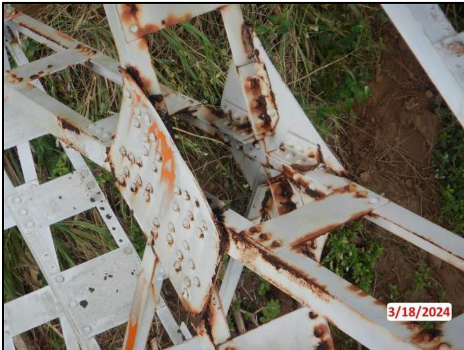
Photograph 124. Tower 5, Level 1, Columns C and D, center gusset, looking northeast. Pack rust up to 1" thick, CS3.
