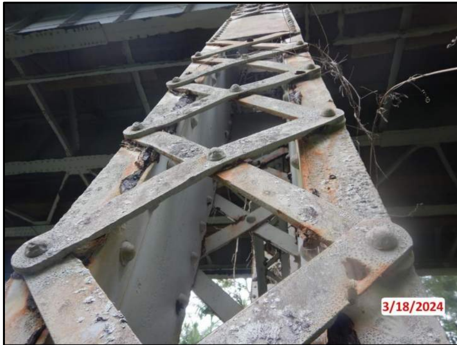
Photograph 10. Bent 1, Level 1, lower section, Column D, west face, lacing bars, looking east. (2) with corrosion holes, up to 2" diameter, CS3.
