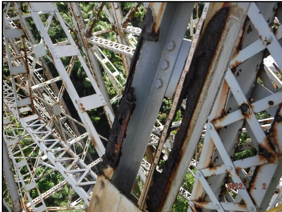
Photograph 143. Bent 7, Level 1, lower section, between Columns A and B, diagonal bracing top angle, looking southwest. section loss, 100% loss for 2' 4" L, CS3.
