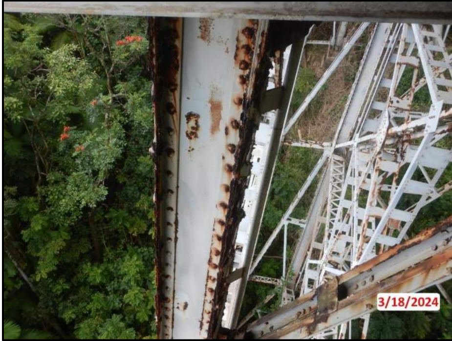
Photograph 37. Bent 3, Level 1, upper section, Column A, exterior face edges over top 12', looking south. Widespread laminar corrosion, CS3.
