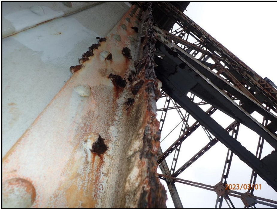
Photograph 91. Bent 4, Level 4, Column C, looking northeast. Knife-edging of flanges, CS3.
