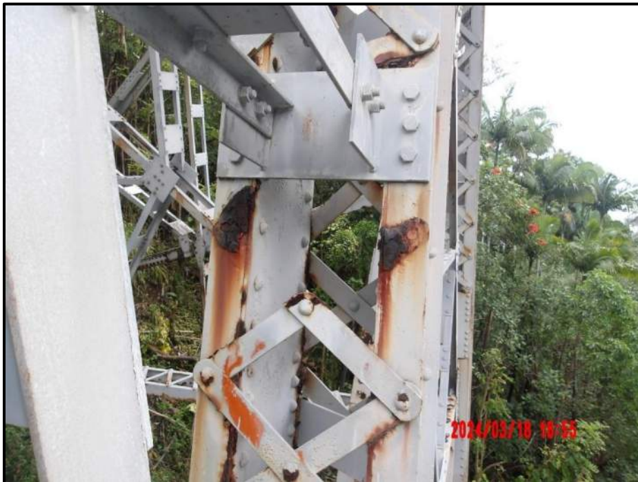
Photograph 122. Bent 8, Level 1, lower section, Column C, west face, (2) lacing bars, looking east. 100% section loss, CS3.
