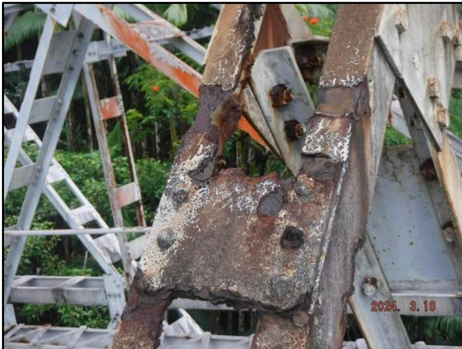
Photograph 38. Bent 3, Level 1, lower section, between Columns B and C, lower east diagonal bracing near Column B, adjacent to batton plates top flange of angles, looking west. Knife-edging with areas of 4" L x 2" W of up to 100% section loss, CS3.
