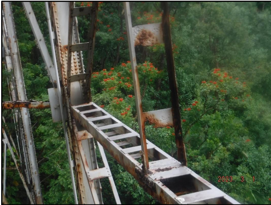
Photograph 97. Tower 3, Level 2, Column A, vertical bracing, looking north. Batten plates typically exhibit pitting up to 1/8" deep with corrosion holes up to 5" diameter, CS3.
