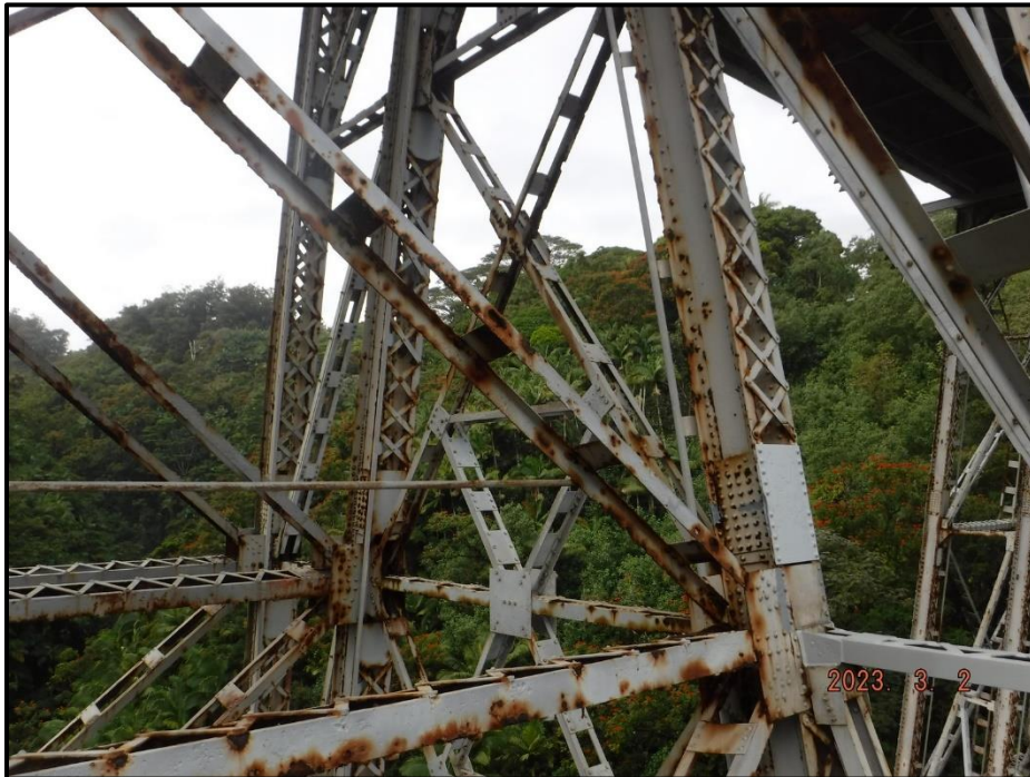
Photograph 93. Tower 3, Level 1, Column B, lower north diagonal bracing, looking west. Worst case is a 4" diameter corrosion hole near center gusset plate. Approximately 60% section remaining, CS3.
