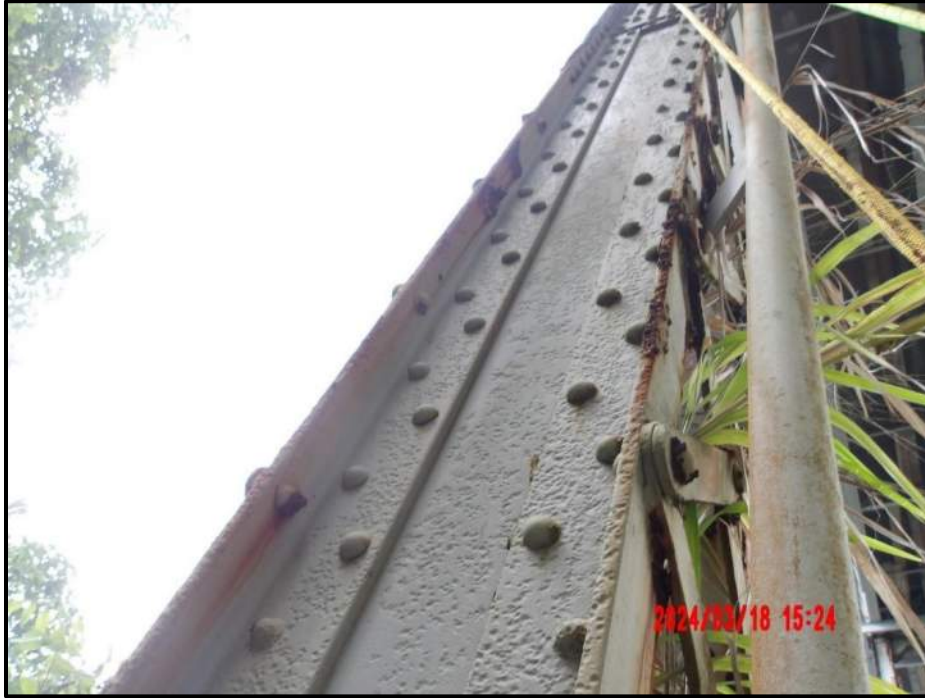
Photograph 123. Bent 8, Level 2, Column A, bottom section, north face angles and web, looking southeast. Painted over pitting, full height x up to 3/16" deep, CS3.
