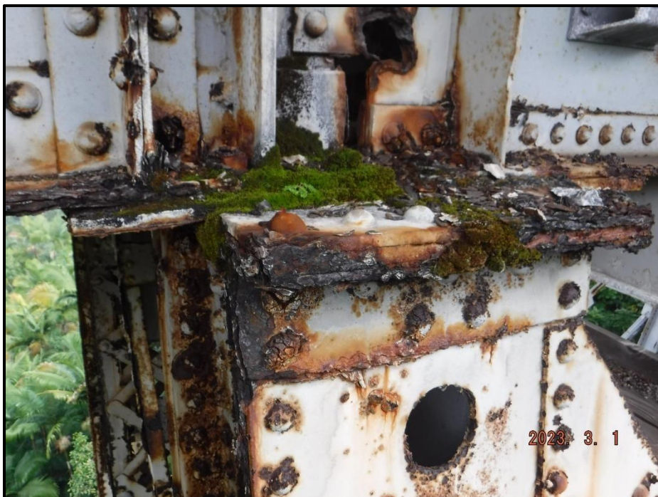
Photograph 48. Bent 3, Span 4, Girder 4 bearing, looking west. Peeling paint and heavy corrosion throughout. The bottom plate has 10% section loss along the edges and pack rust on the north side, CS3.
