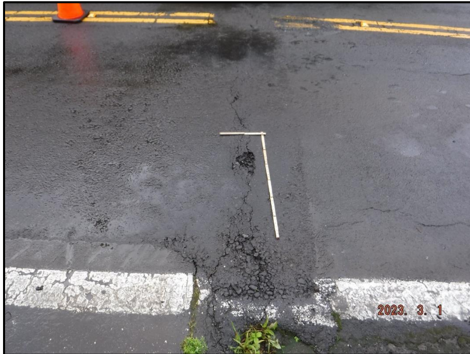
Photograph 23. South Abutment Joint, NB Lane, looking west. 12' L x up to 1/8" W transverse crack with adjacent spall, CS3.
