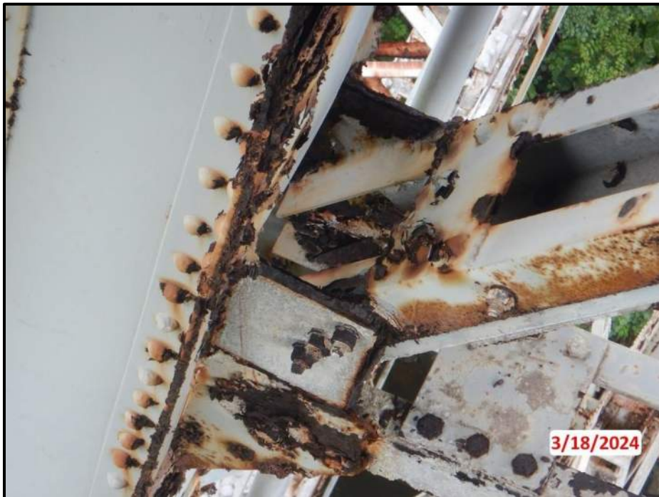
Photograph 46. Bent 4, Level 1, upper section, Column D, upper gusset plates, looking northwest. Heavy laminar corrosion and approximately 1/4" to 3/8" remaining section on gusset plate between diagonal and horizontal bracing member, CS3.
