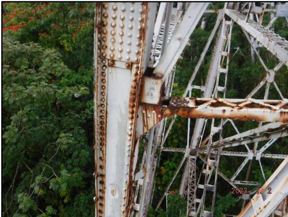
Photograph 121. Bent 6, Level 1, lower section, between Columns C and D, horizontal bracing, looking north. 25% section loss with knife-edging on south angle. Column D gusset plate has severe laminar corrosion between the horizontal and diagonal and appears to be failing at that location (deformation to the north), CS3.
