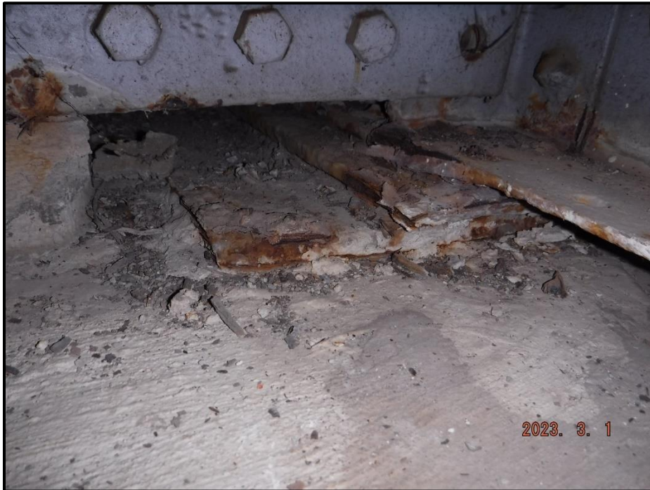
Photograph 47. South Abutment, Girder 3 bearing, looking southwest. Moderate corrosion with minor section loss, CS3.
