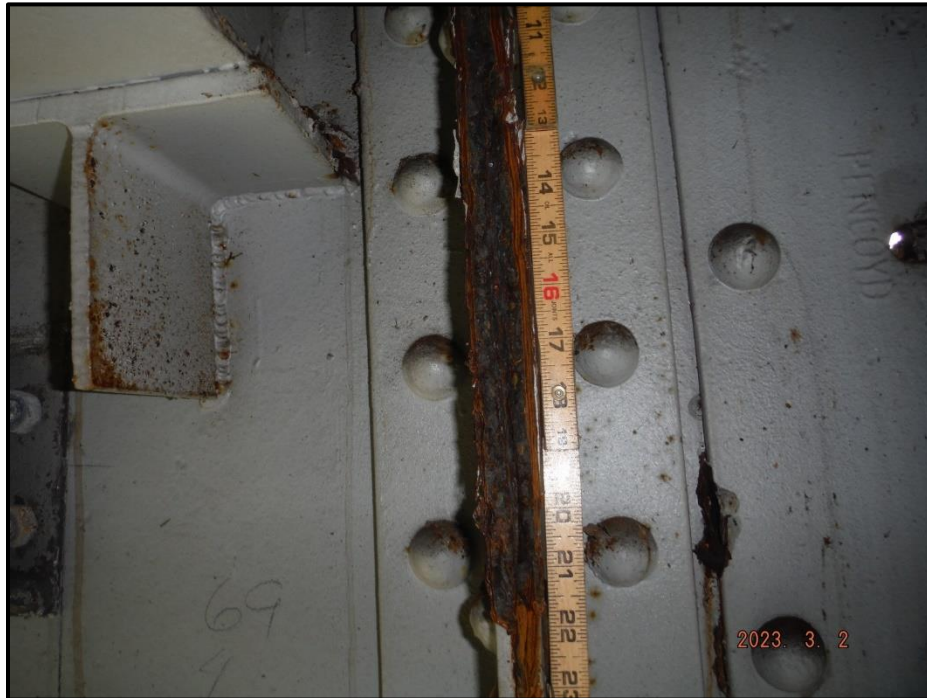
Photograph 37. Span 6, Bent 5, web stiffener above Girder 1 bearing, looking east. 3/16" thick pack rust causing a 1' 11" H x 1" deflection, CS3.
