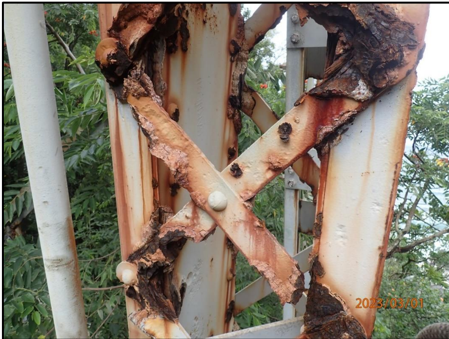
Photograph 125. Bent 6, Level 3, Column B, mid-height, west face, looking east. Multiple lacing bars with 100% section loss, CS3; similar condition on west face of Level 3, Level 2, west face, Level 4 both faces, and Level 5 east face. The west face of Level 5 only has five bars total intact.
