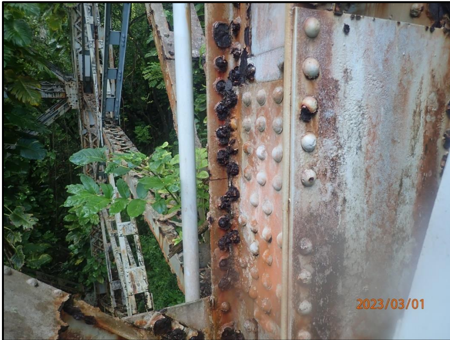
Photograph 150. Bent 7, Level 3, Column B splice plate, looking south. Majority of connection rivets for Column B have section loss and corrosion, CS3.
