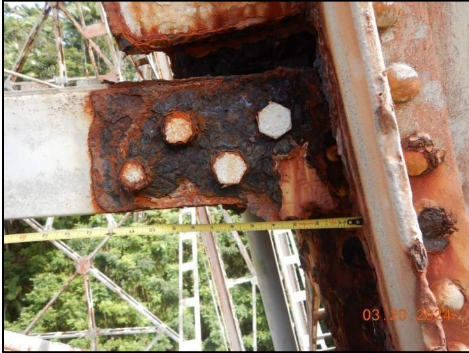
Photograph 75. Bent 5, Level 2, Column D, horizontal bracing gusset plates, looking south. Heavy laminar corrosion with up to 100% section loss with 15% section remaining of the north gusset plate and repair plates becoming ineffective. The gusset plate is completely detached from the column, CS4.
