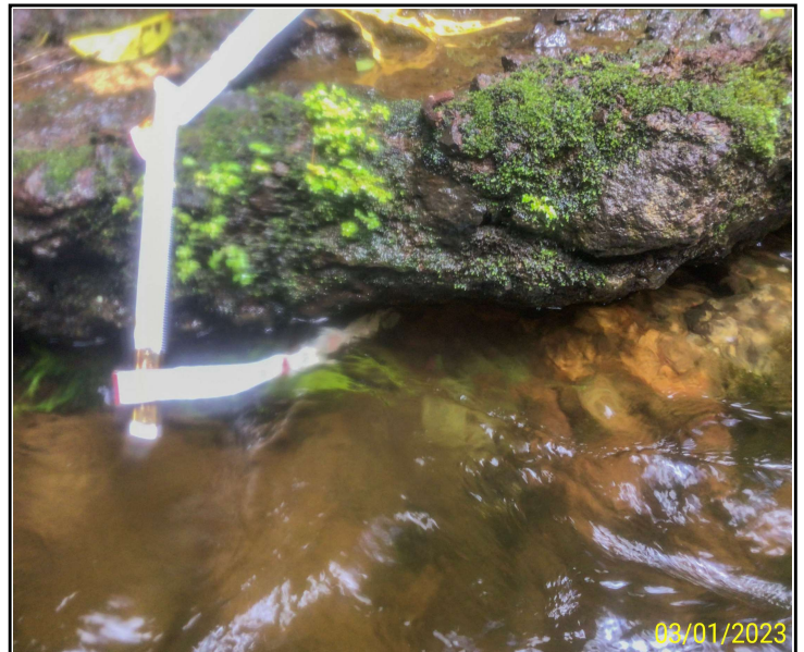
Photo 16. Bent 6, Column B footing, looking north. Undermined, up to 4" H x 6" D, CS2
