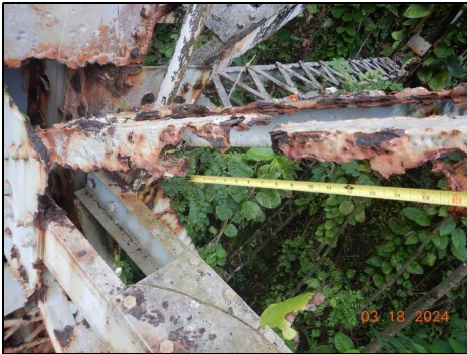
Photograph 92. Bent 6, Level 4, between Columns B and C, lower west diagonal adjacent to Column C, looking northwest. Corrosion holes and knife-edging at exterior vertical flange and section of missing vertical flange at lower end for 1' 6" L, CS3.
