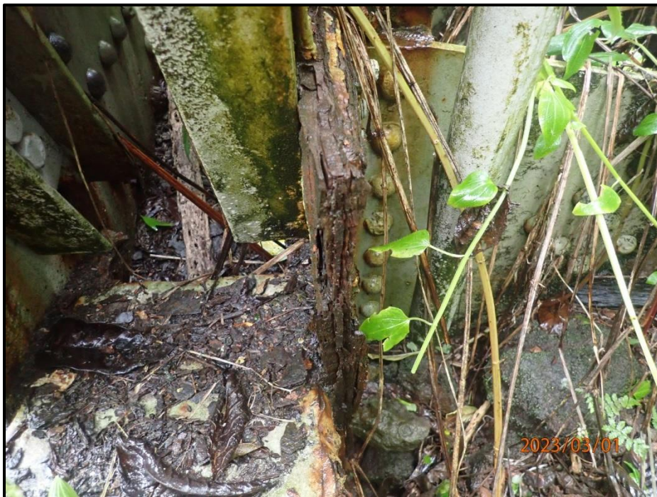
Photograph 82. Bent 3, Level 4, Column A, just above bearing, gusset plates, looking east. Plates are distorted and bowed to the south up to 1/8" for the horizontal bracing member, CS3.
