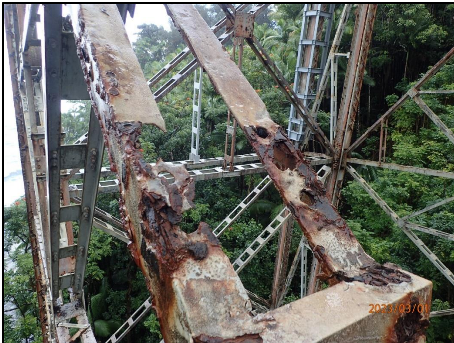
Photograph 113. Bent 5, Level 3, between Columns B and C, lower west diagonal near Column C, looking east. 10" of top flange missing on both angles, CS3.
