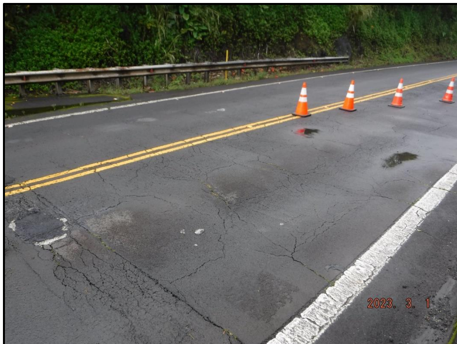
Photograph 52. North and south approach roadways, looking northwest. Depressed and worn surface in wheel lines of both lanes, up to 1/2" wide map cracks throughout, some with vegetation growth.
