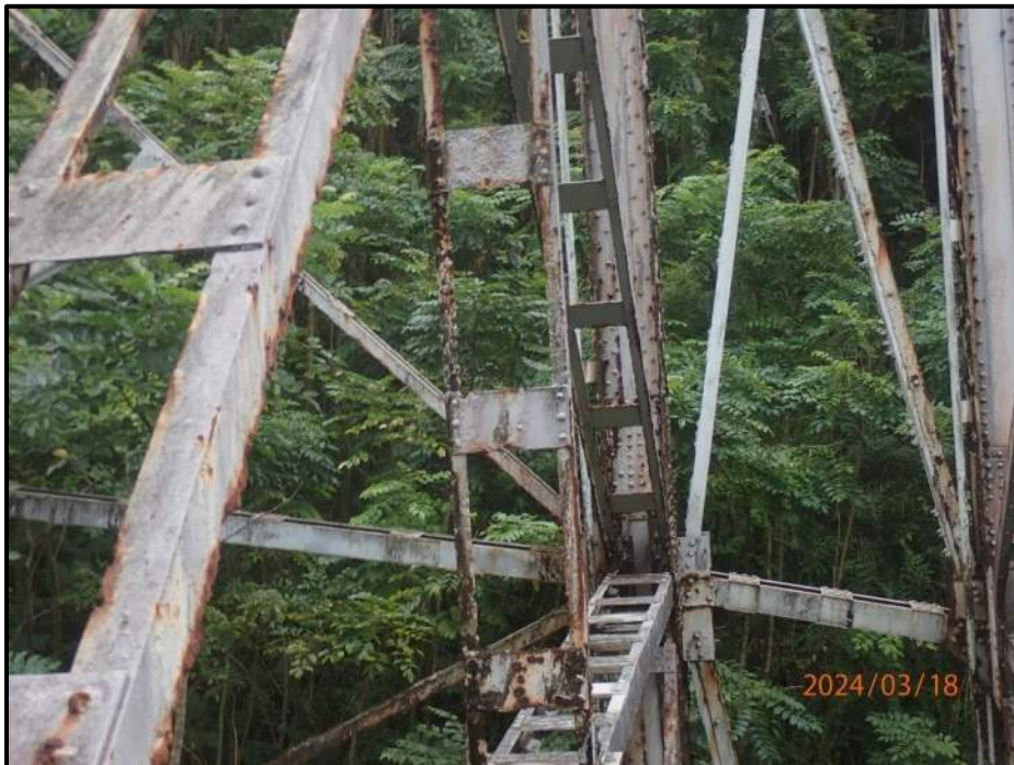
Photograph 68. Tower 3, Level 4, Column C, vertical bracing, looking east. Heavy corrosion of angles and batten plates on vertical with knife-edging, pitting up to 3/16" deep and corrosion holes up to 5" diameter, CS3.
