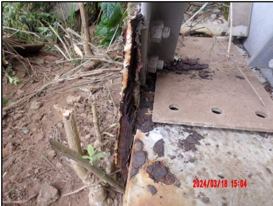
Photograph 126. Bent 9, Level 1, lower section, between Columns B and C, lower horizontal bracing center gusset plate, looking west. Heavy laminar corrosion, up to 1-1/4" W with up to 50% section loss, CS3.
