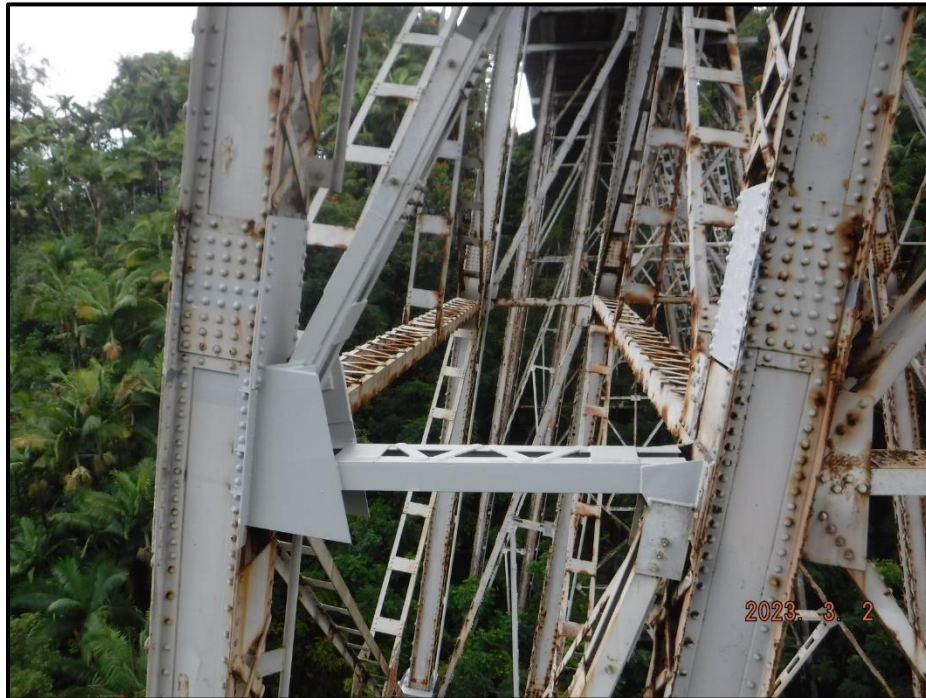
Photograph 107. Bent 5, Level 1, lower section, between Columns A and B, lower horizontal bracing, looking south. Column A lower gusset plates exhibit up to 100% section loss above and below horizontal member with 5" L segments of 25% section left holding members. – Repaired.
