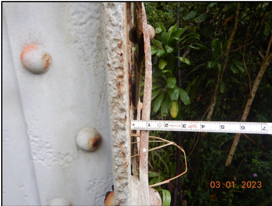
Photograph 153. Bent 8, Level 2, Column A, looking north. Batten plates and lacing bars are typically bent to the east on the east side, CS3.
