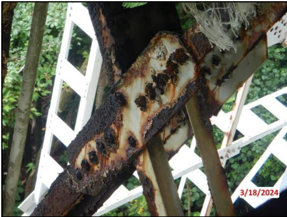
Photograph 36. Bent 3, Level 1, upper section, between Columns B and C, center gusset plates, looking southeast. Laminar corrosion on plates and transverse bracing members, CS3.
