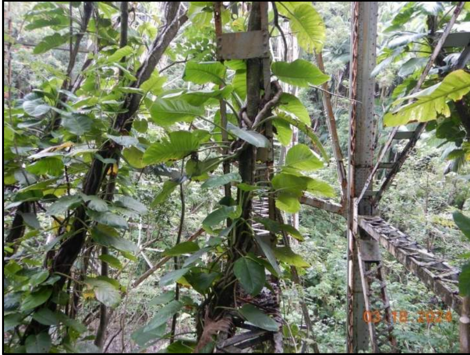
Photograph 111. Tower 4, Level 4, Column C, horizontal bracing, near center, looking south. Large tree growing through the structure (incidental).
