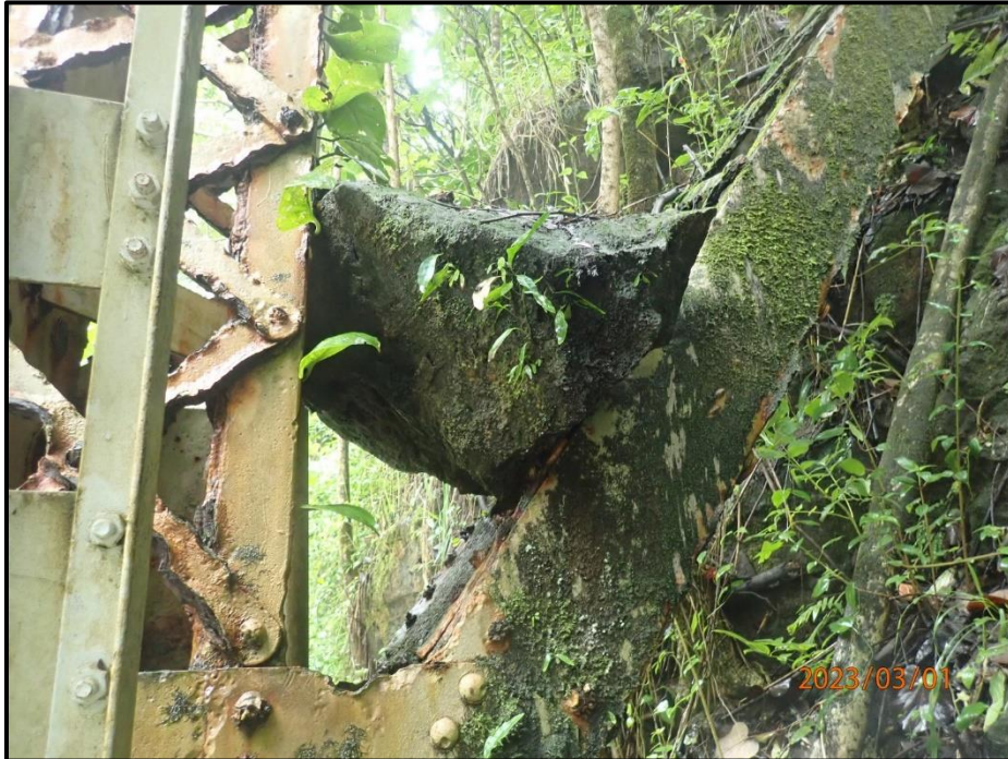
Photograph 136. Tower 4, Level 6, Column B, looking west. 3' diameter boulder on top of diagonal member at bottom connection; member appears to be deformed as a result.
