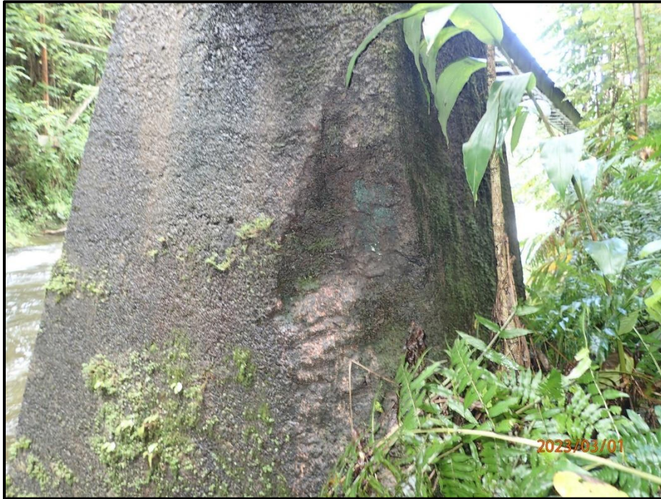
Photograph 118. Bent 5, Level 6, Column C, footing, southwest corner, looking east. 5' W x 1' 4" H x 1' deep spall, CS3.
