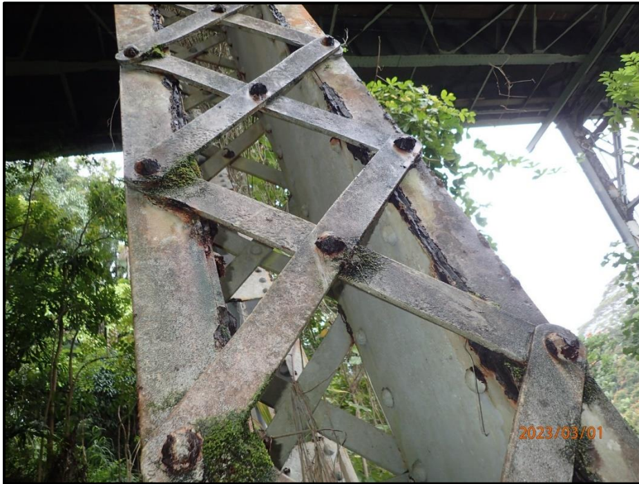
Photograph 55. Bent 1, Level 1, Column A, looking northwest. Typical pitting, pack rust and laminar corrosion, CS3.
