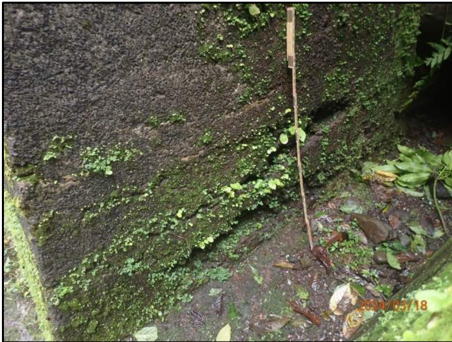
Photograph 84. Bent 5, Level 6, Column C, footing, base of pedestal on west side, looking east. 6' x 2' area of abrasion with course aggregate exposed and missing up to 4" deep, CS3.
