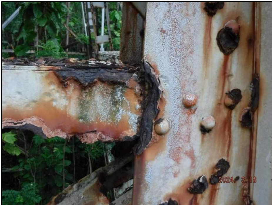
Photograph 88. Bent 6, Level 3, west of Column B, south gusset plate, looking north. 1-1/2" W x 8" H area of 100% section loss, CS3.
