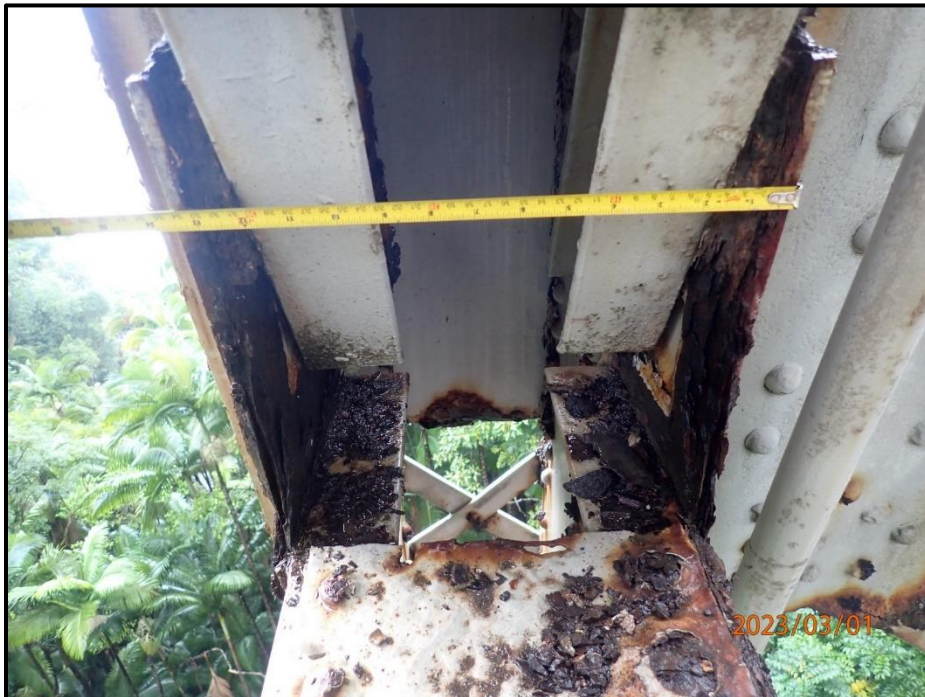
Photograph 78. Bent 3, Level 1, lower section, Columns A and B, horizontal bracing, looking east. Pack rust up to 1 1/2" thick with section loss up to 30% to gusset plates and 100% loss to rivet heads of batten plate, CS3.
