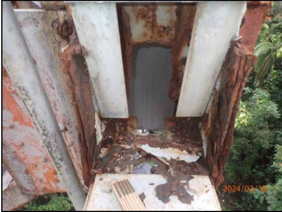
Photograph 77. Bent 5, Level 3, between Columns C and D, diagonal bracing, outboard angles, looking south. 10" L x up to full height section loss with adjacent corrosion holes, extreme deterioration up to 90% cross section reduction having no change from previous inspection, CS4.
