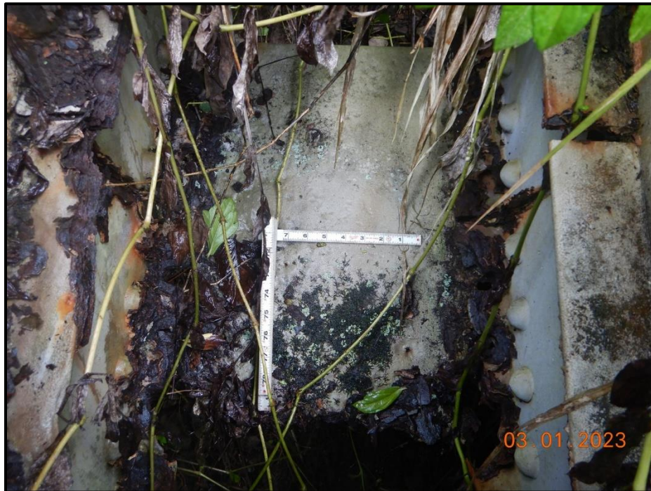
Photograph 155. Tower 5, Level 2, Column B, bottom horizontal, looking north. Underside batten plate has severe laminar corrosion and is not connected to the channels, CS3.
