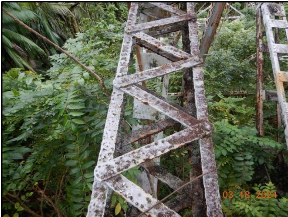
Photograph 32. Tower 2, Level 2, Column D, horizontal bracing, looking north. Pinholes (corrosion holes) throughout the length, CS3.
