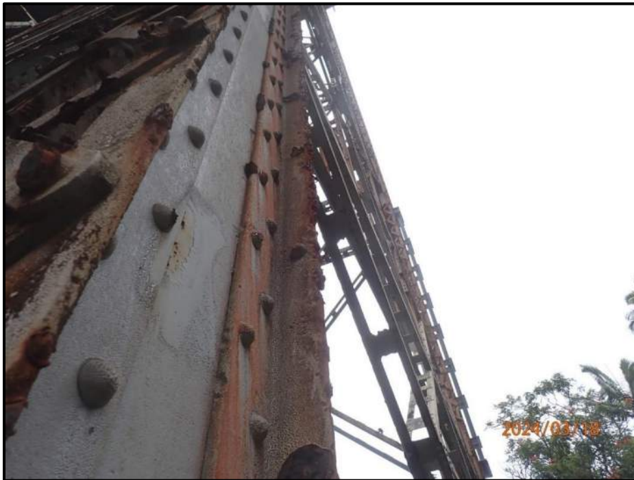
Photograph 54. Bent 4, Level 4, Column C, flanges, looking east. Knife-edging, CS3.
