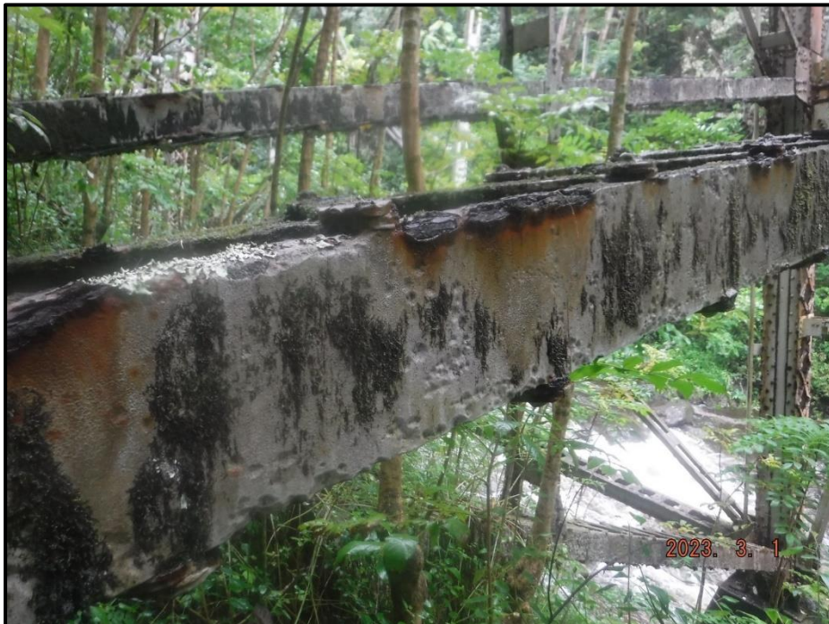
Photograph 100. Tower 3, Level 6, Column A, lower horizontal bracing, looking northwest. Knife-edging with 4" L x 1-1/2" H section loss, CS3.
