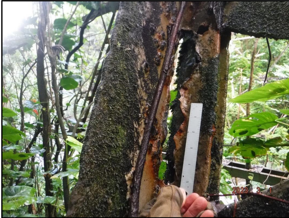
Photograph 140. Tower 4, Level 5, Column C, mid-diagonal mid-length, interior top angle, looking south. 100% section loss for most of length of horizontal flange. Approximately 20% loss of cross sectional area, CS3.
