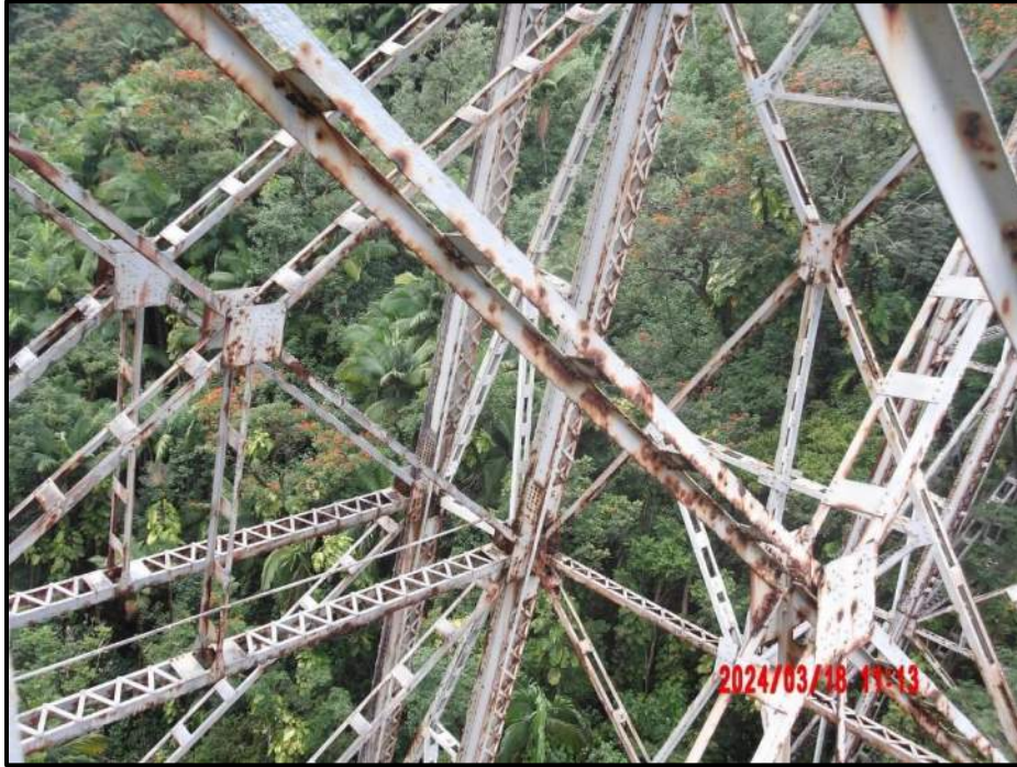
Photograph 61. Tower 3, Level 2, Column A, upper south to lower north diagonal bracing, looking north. Global distortion to the diagonal members within level. Upper south diagonal bracing, east leg has corrosion holes, up to 1" diameter, CS3.
