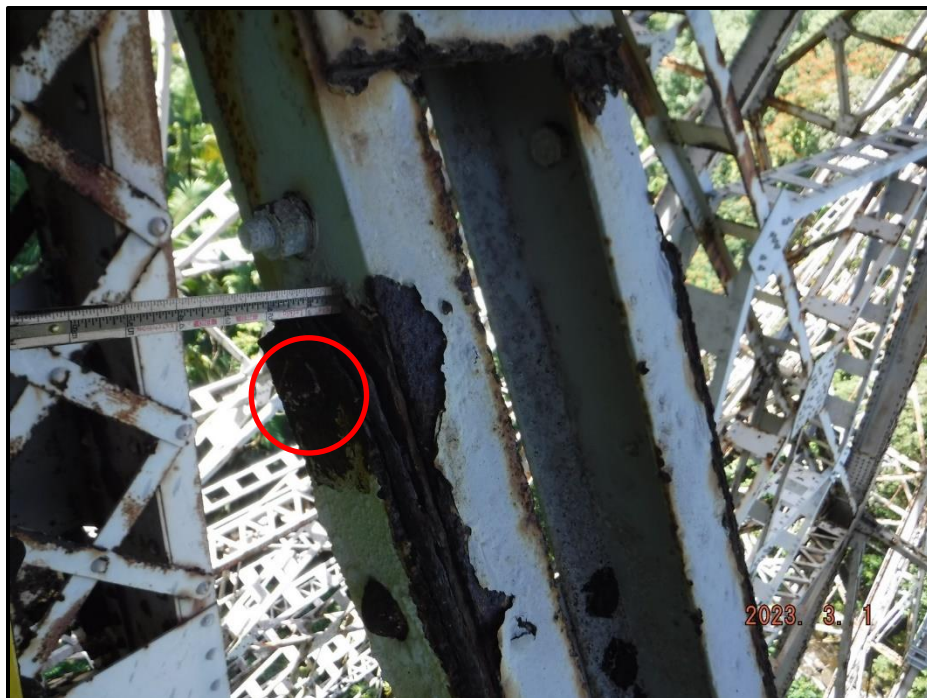
Photograph 58. Bent 2, Level 1, upper section, between Columns A and B, diagonal bracing, both cover plates at mid-length, looking north. Pack rust up to 3/4" thick causing separation of plate and one broken rivet on north cover plate, CS3.
