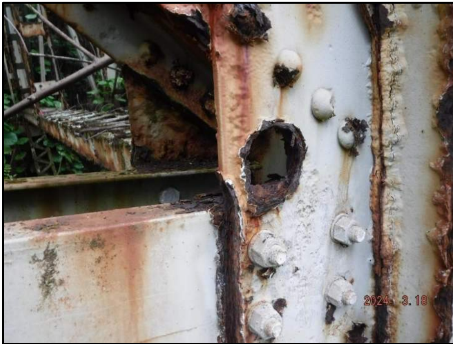
Photograph 90. Bent 6, Level 4, Column B, exterior gusset plate at horizontal bracing, looking south. 3-1/2" diameter corrosion hole, CS3.
