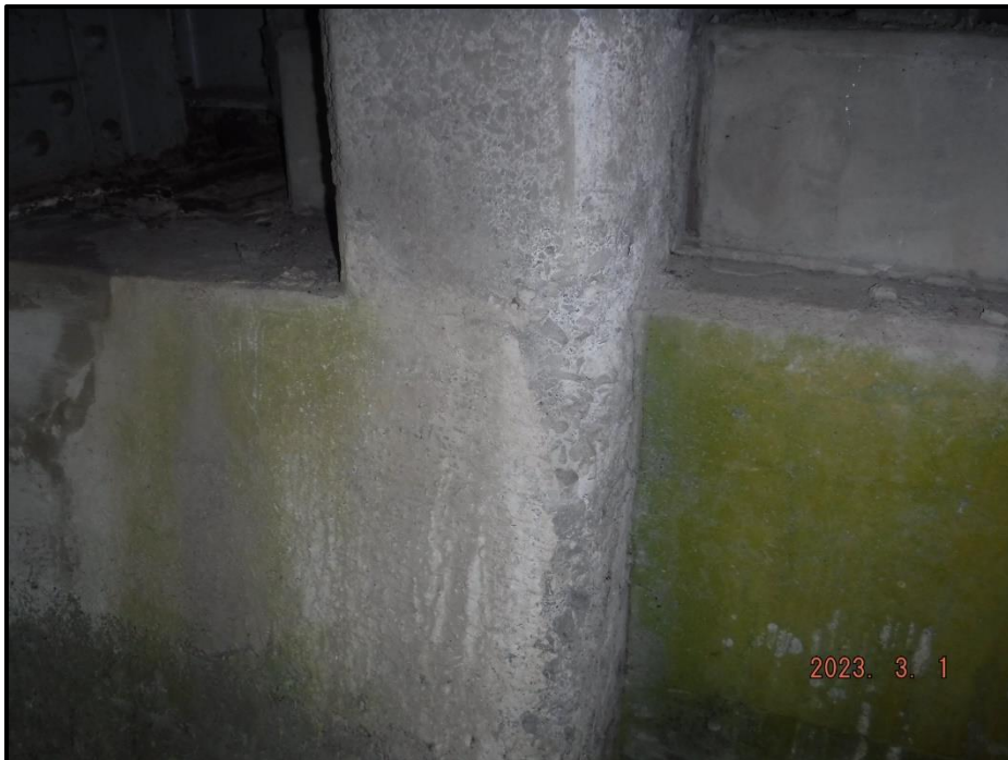
Photograph 42. South Abutment, Bay 3, center section, looking south. Spall, 1' 4" H x 8" W x 1" deep, CS3.
