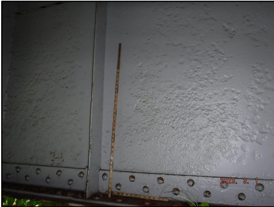
Photograph 31. Span 2, Girder 1, west face, looking east. 25' L section of painted over pitting up to 1/8" deep, CS3.
