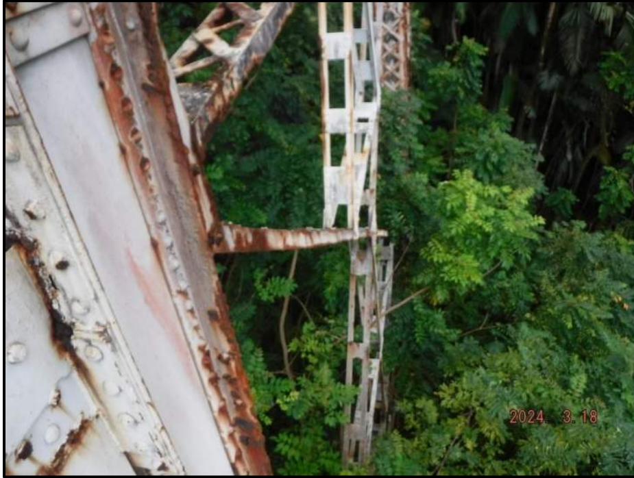
Photograph 43. Bent 3, Level 3, between Columns B and C, upper east diagonal, looking west. Bowed up to 1" out of plane over full length, CS3.
