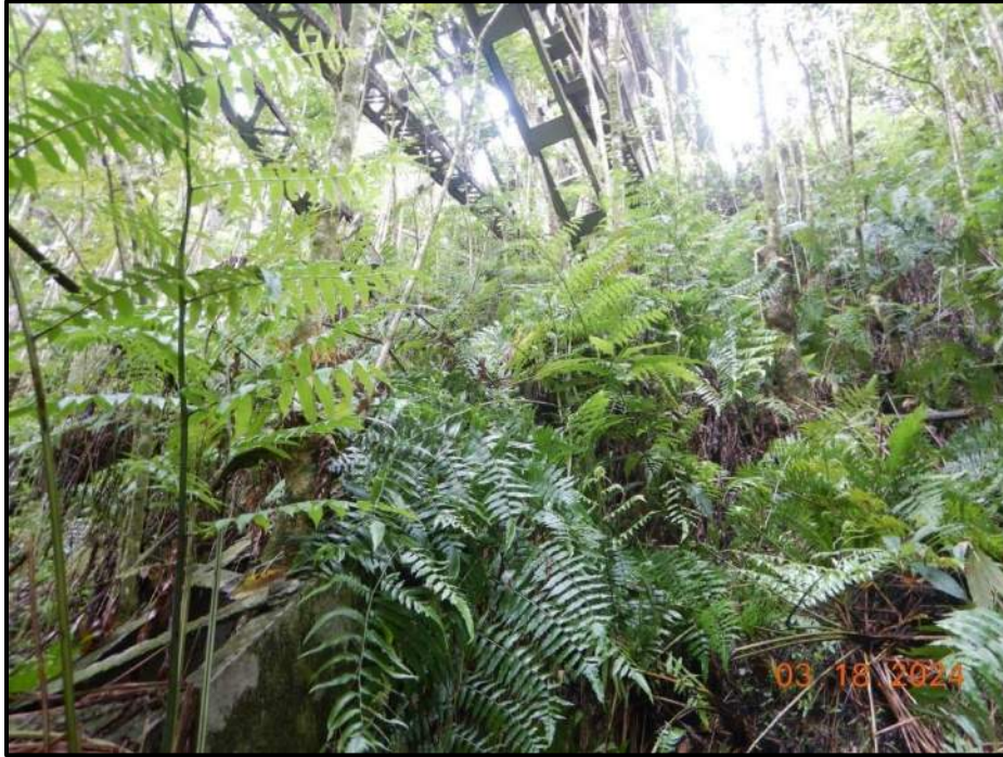
Photograph 33. Tower 2, Level 4, Column D, lower diagonal bracing, looking south. Heavy growth with trees growing through the members.
