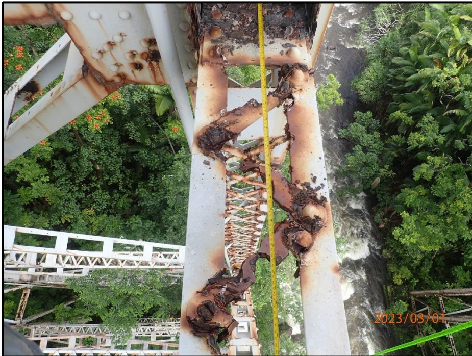
Photograph 120. Bent 6, Level 1, lower section, between Columns A and B, horizontal bracing, looking east. 100% section loss; (5) of (6) bars, CS3.
