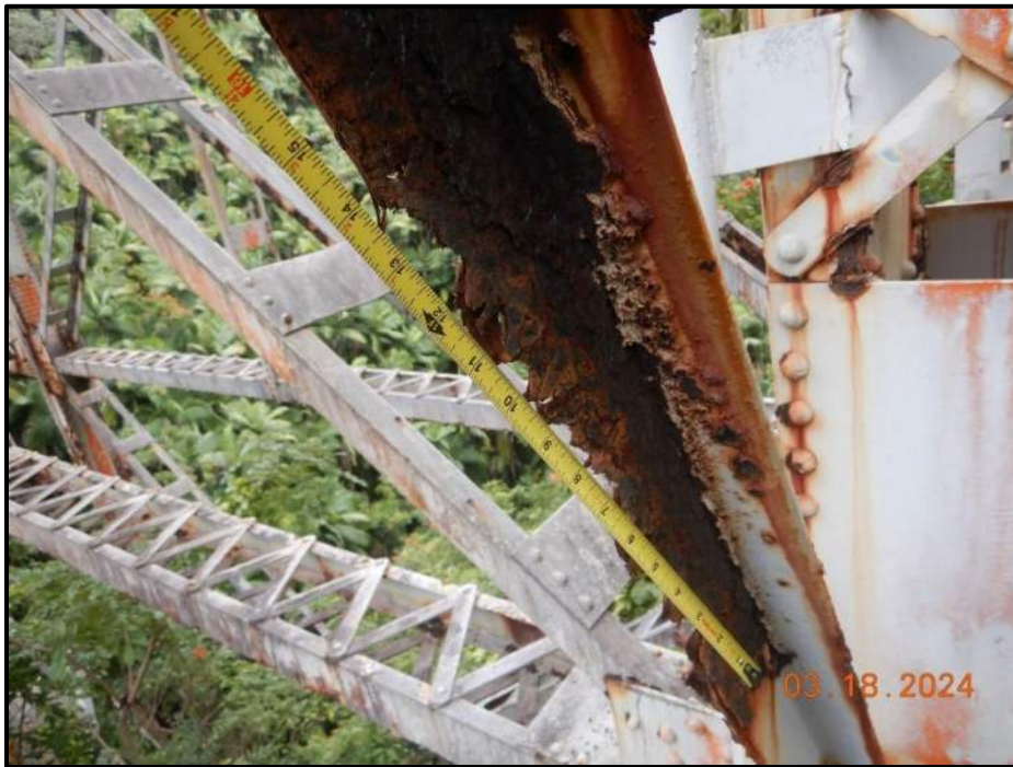
Photograph 116. Bent 7, Level 2, between Columns B and C, lower west diagonal bracing, south angle, looking southwest. Heavy laminar corrosion and knife-edging over 4' L, CS3.
