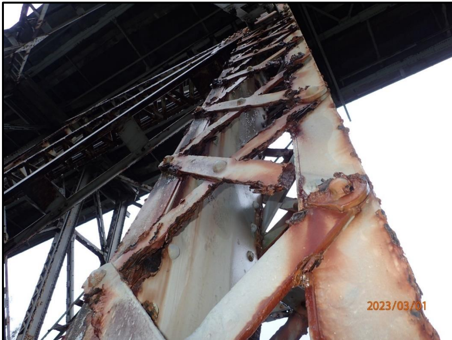
Photograph 88. Bent 4, Level 2, Column C, looking northeast. 50% of lacing bars on west face have 100% section loss, remaining bars on both faces have average 30% section loss, CS4.
