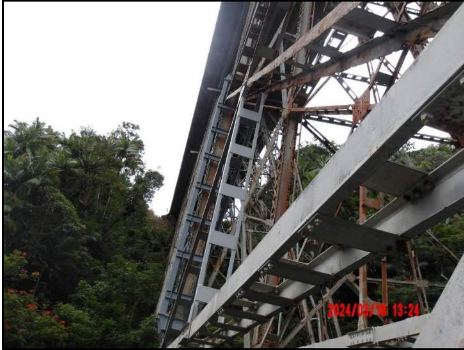
Photograph 63. Tower 3, Level 3, Column A, lower south diagonal, and vertical bracing, looking southeast. Repair in good condition.
