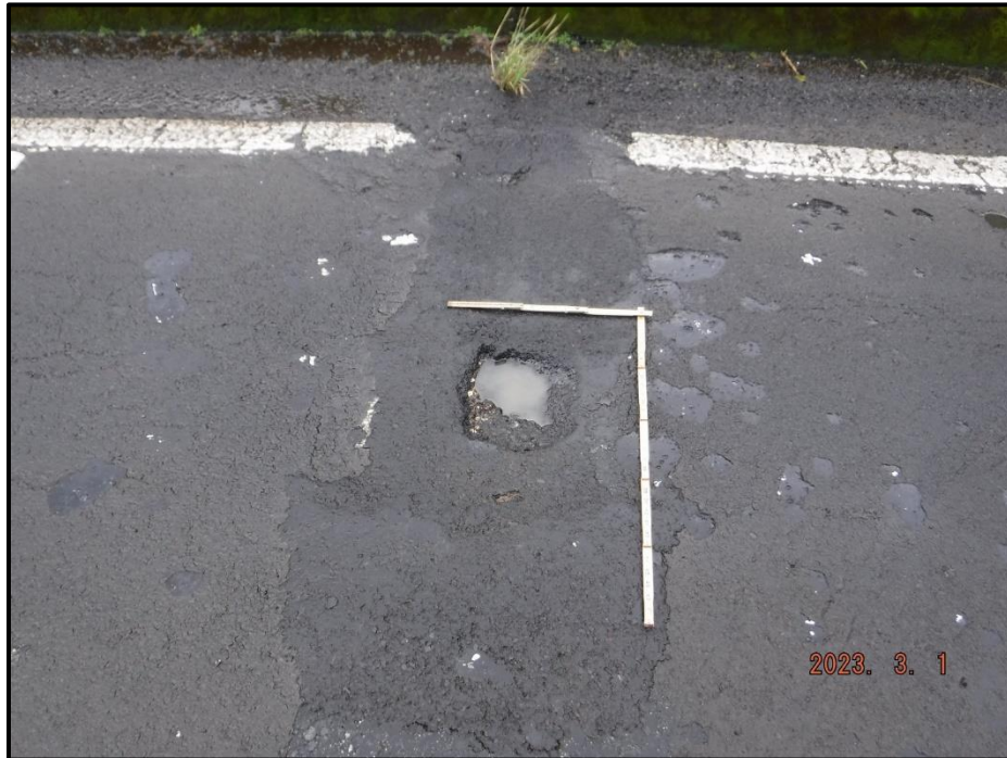
Photograph 21. Bent 9 Joint, SB lane, wearing surface, looking west. 1' 4" L x 1' 9" W x 1" deep cracked and settled patch with 5" L x 11" W x 1" deep pothole within with exposure of steel plate and joint material, CS2, CS4.
