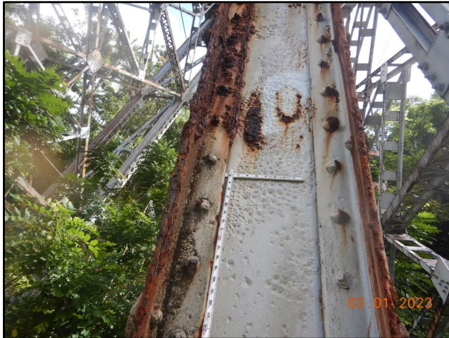
Photograph 83. Bent 3, Level 4, Column C, looking northeast. Typical painted over pitting, laminar corrosion, knife-edging, and corroded rivet heads, CS3.
