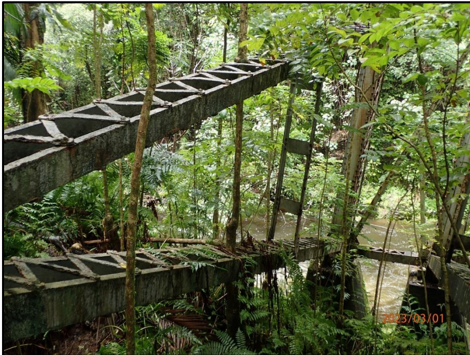
Photograph 105. Tower 3, Level 6, Column D, upper horizontal bracing, looking northwest. Vegetation, tree growing through members.
