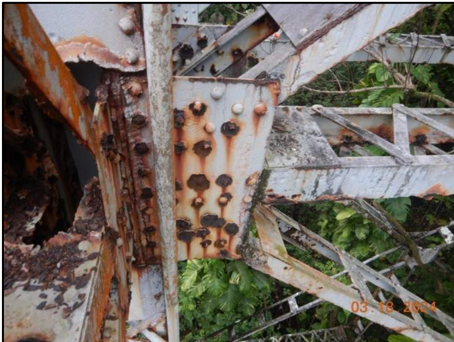
Photograph 108. Tower 4, Level 3, Column C, gusset plate connecting bracing to Bent 6, looking west. (14) of (18) rivet heads connecting the gusset plate to the column have 20% remaining on the inside face. East channel of bracing has more severe section loss at this location with (5) corrosion holes in the web up to 1" diameter, CS4.
