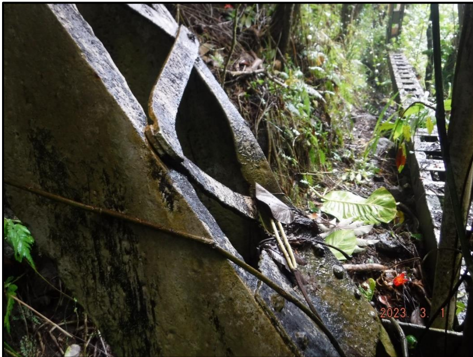
Photograph 141. Tower 4, Level 6, Column C, adjacent to Bent 6 pedestal, interior channel, looking east. 3" downward deformation over 1' 6", CS3.
