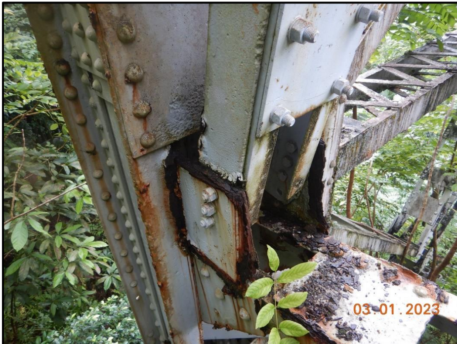
Photograph 64. Bent 2, Level 2, Column D, transverse bracing gusset plates, looking northwest. Typical heavy laminar corrosion, CS3.
