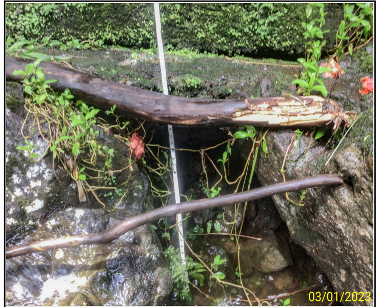
Photo 14. Bent 6, Column A, looking north. Undermined, 3' L x 2' H x 1.5" D, CS3
