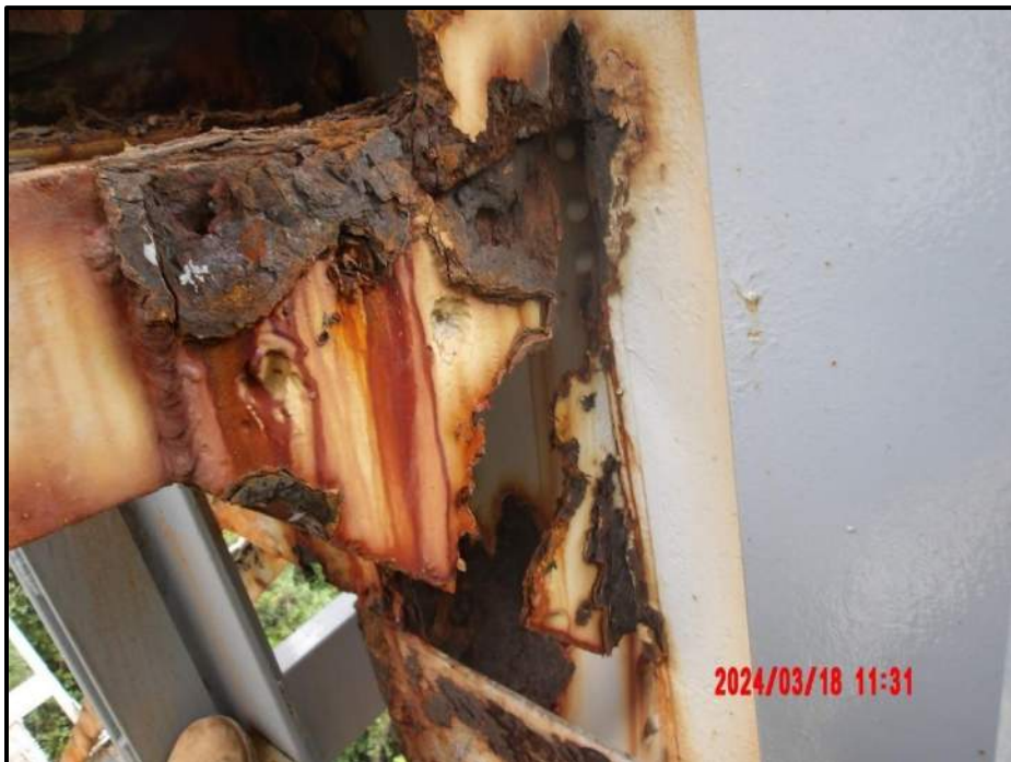
Photograph 48. Bent 4, Level 2, Column A, exterior gusset plate, looking northeast. Corrosion, pack rust up to 1" thick with areas of up to 100% loss and only retrofit gusset plate remaining, CS3.
