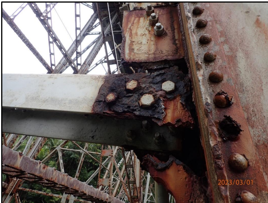
Photograph 111. Bent 5, Level 2, Column D, horizontal bracing gusset plates, looking south. Heavy laminar corrosion with up to 100% section loss with 15% section remaining of the north gusset plate and repair plates becoming ineffective, CS4.
