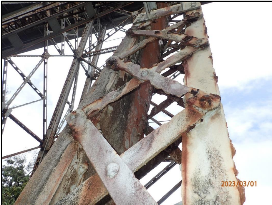
Photograph 89. Bent 4, Level 3, Column C, looking east. Lacing bars have an average 75% section loss in this section of column. Except for top 10' of west face which are in good condition, CS3.
