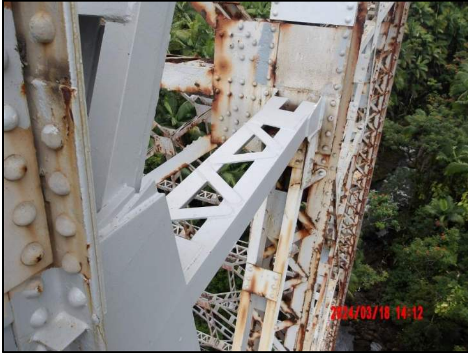
Photograph 71. Bent 5, Level 1, lower section, between Columns A and B, lower horizontal bracing, looking west. Column A lower gusset plates exhibit up to 100% section loss above and below horizontal member with 5" L segments of 25% section left holding members. - Repaired
