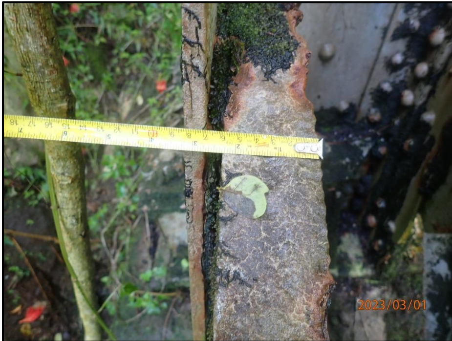
Photograph 65. Bent 2, Level 3, Column A, horizontal bracing, gusset plate, looking south. Pack rust up to 1/4" thick, CS3.
