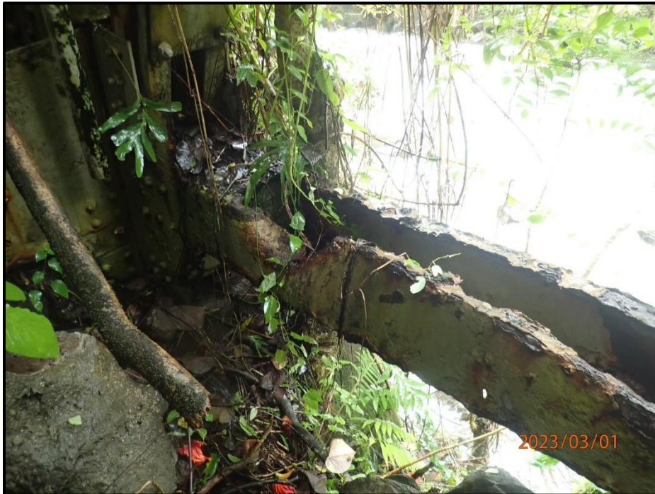
Photograph 132. Bent 6, Level 6, between Columns A and B, horizontal bracing, looking northeast. Member impacted by falling rocks, CS3.
