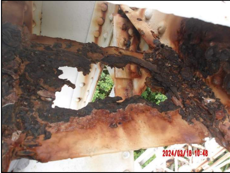
Photograph 57. Tower 3, Level 1, Column A, horizontal bracing, lower batten plate, looking south. Corrosion hole, 5" L x 10" W, CS3.
