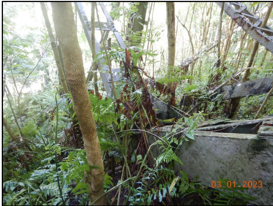
Photograph 74. Tower 2, Level 4, Column D, lower diagonal bracing, looking north. Heavy growth with trees growing through the members.
