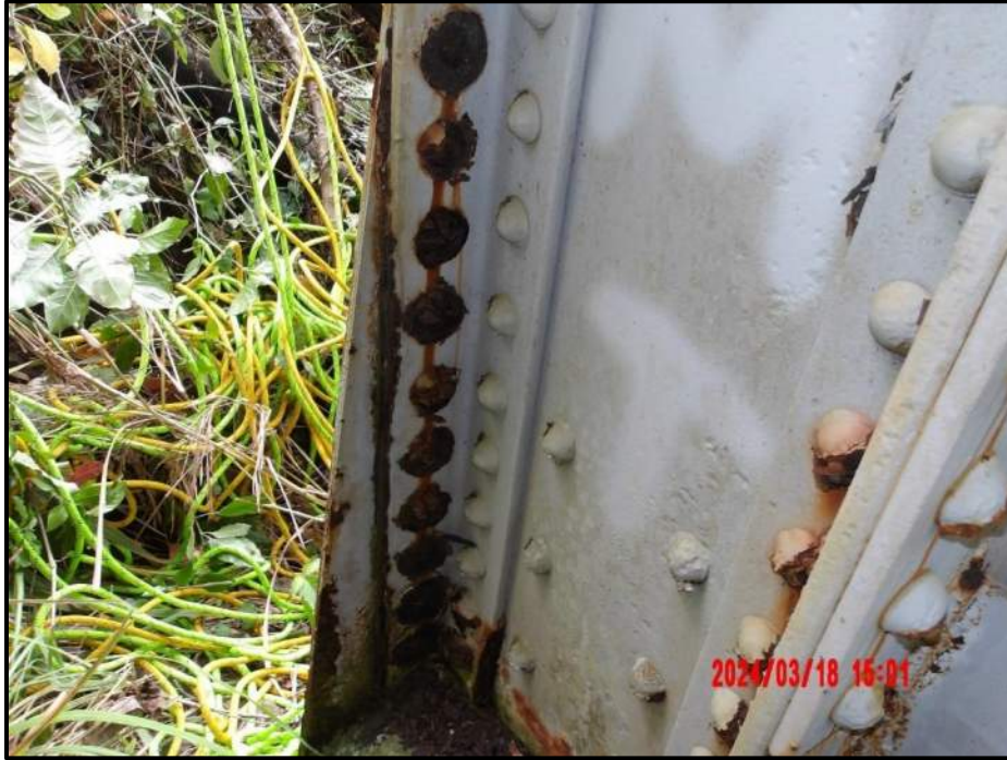
Photograph 73. Bent 5, Level 2, Column B, exterior gusset plate, looking south. Multiple corrosion holes up to 5" x 2-1/2" and pitting up to 1/16" deep in exterior gusset plate; interior rivet heads at connection to column typically have up to 100% section loss in this location, CS3.
