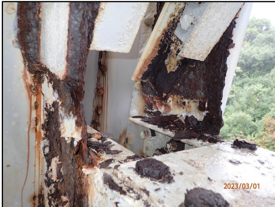
Photograph 84. Bent 4, Level 1, upper section, Column D, upper gusset plates, looking northwest. Heavy laminar corrosion and approximately 1/4" to 3/8" remaining section on gusset plate between diagonal and horizontal bracing member, CS3.
