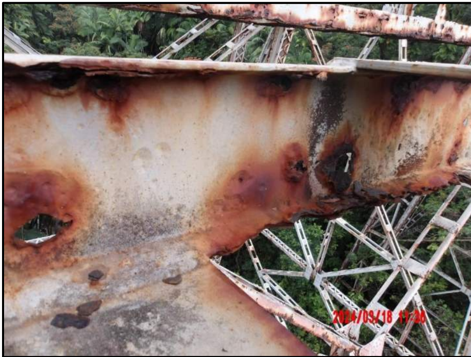
Photograph 60. Tower 3, Level 2, Column A, horizontal bracing, near Bent 4, looking northwest. 50% section loss to entire member with holes throughout, CS4.
