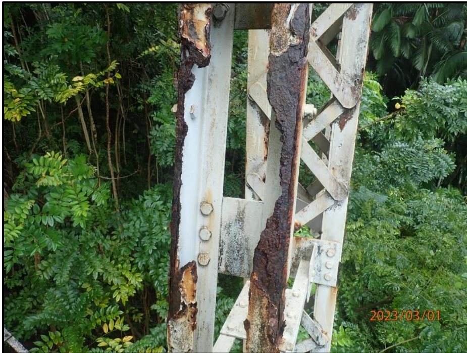
Photograph 81. Bent 3, Level 3, between Columns A and B, diagonal bracing above interior connection, looking east. 3' L x full width of angle area of section loss on top flanges (CS3). Note this member has been retrofitted and retrofit is in good condition.
