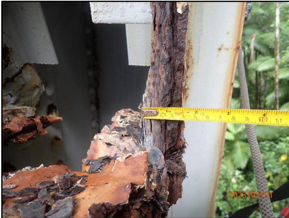
Photograph 61. Bent 2, Level 1, lower section, Column A, interior gusset plates, looking east. Up to 1" W x full length section loss where all members frame in, CS3.
