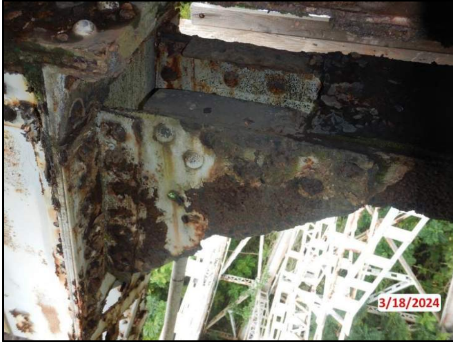
Photograph 35. Bent 3, Level 1, upper section, west of Column A, north gusset plate, looking south. Knife edging and corrosion holes up to 3" x 2" along bottom edge of gusset plate, CS3.
