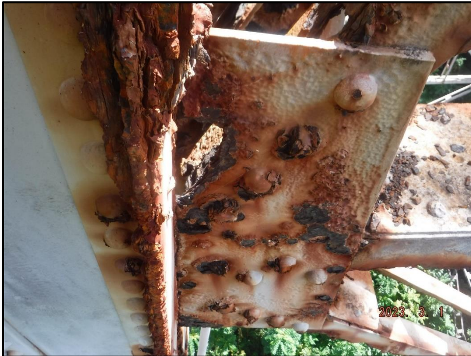
Photograph 110. Bent 5, Level 2, Column B, exterior gusset plate, looking south. Multiple corrosion holes up to 5" x 2 1/2" and pitting up to 1/16" deep in exterior gusset plate; interior rivet heads at connection to column typically have 10% section remaining in this location, CS3.
