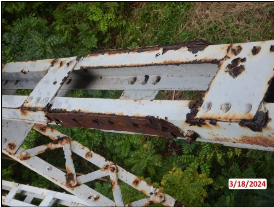
Photograph 12. Bent 2, Level 1, upper section, between Columns A and B, diagonal bracing, both cover plates at mid-length, looking north. Pack rust up to 3/4" thick causing separation of plate and one broken rivet on both cover plates, CS3.
