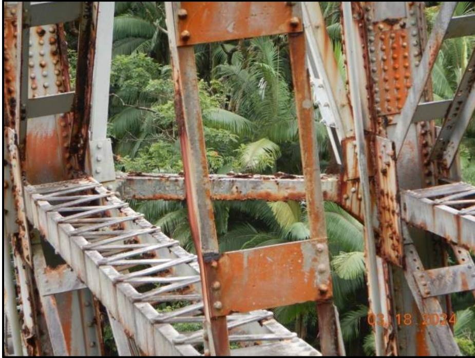
Photograph 107. Tower 4, Level 2, Column C, vertical bracing, looking south. East angles bent out-of-plane 1/2" and west angle, (3) rivets have 90% section loss, CS3.
