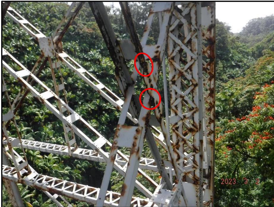
Photograph 144. Bent 7, Level 1, lower section, between Columns B and C, center gusset plate, looking southwest. Heavy pitting, lamellar corrosion, and knife-edging with 2" and 1" diameter corrosion holes, CS3.
