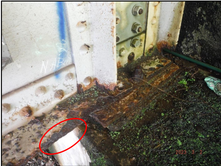
Photograph 39. Span 10, Girder 1, east face at North Abutment, looking northwest. (2) bearing stiffeners have effectively no remaining section at the lower 2" at the base. The eastern bottom flange has 2" W knife-edging, CS3.
