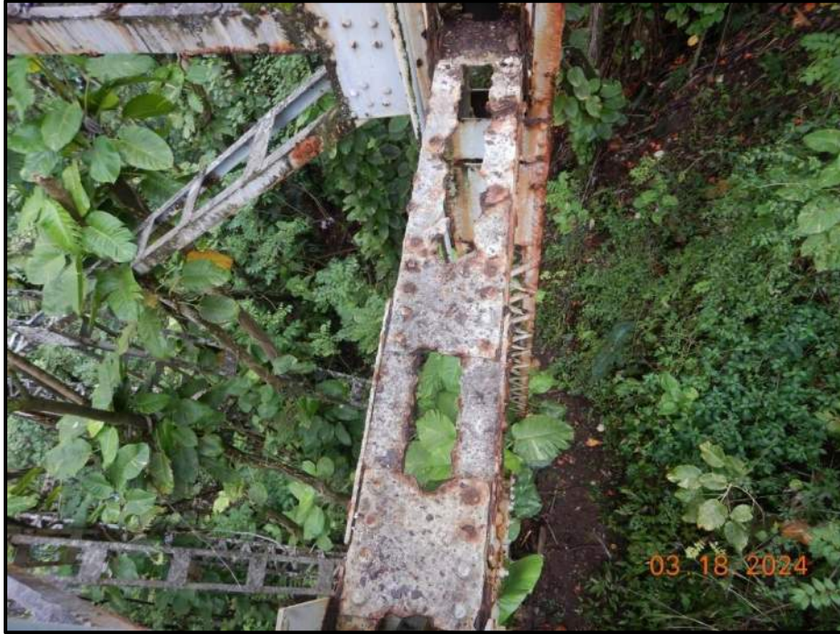
Photograph 121. Bent 7, Level 3, between Columns C and D, horizontal bracing, looking west. Up to 100% section loss to batten plates, knife edging on top flange angles, and missing lacing bars, CS3.
