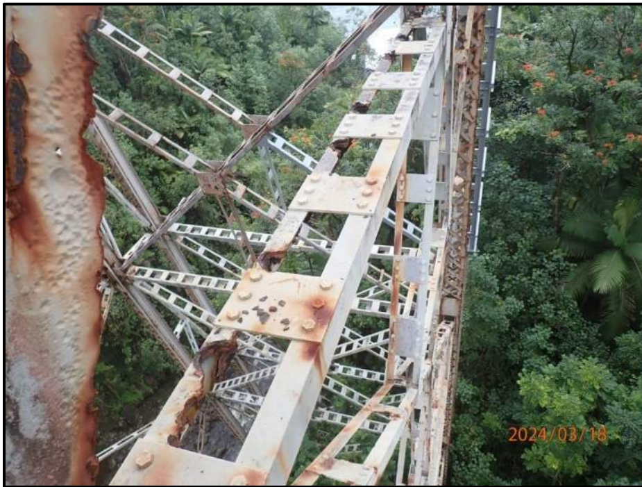
Photograph 50. Bent 4, Level 2, between Columns B and C, horizontal bracing adjacent to Column C, vertical connection, interior top flange along member, looking east. (7) corrosion holes, up to full width of top flange x 5" L, CS3.
