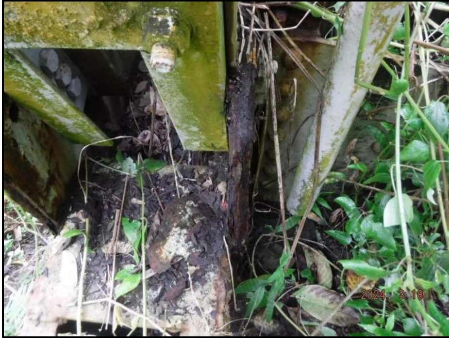
Photograph 45. Bent 3, Level 4, Column A, just above bearing, gusset plates, looking east. Plates have minor distortion and bowed to the south less than 1/8" due to laminar corrosion, CS3.
