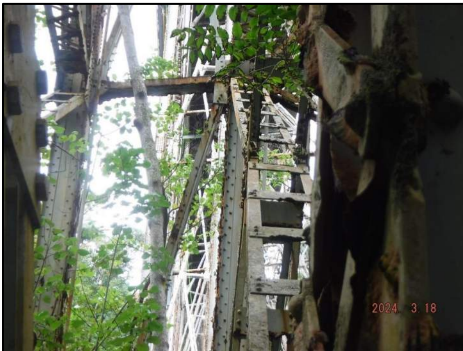
Photograph 104. Tower 4, Level 4, Column B, looking south. All bracing in this level bowed up to 6" inwards (west); vertical member angles have deformations up to 1" over 2', CS3.
