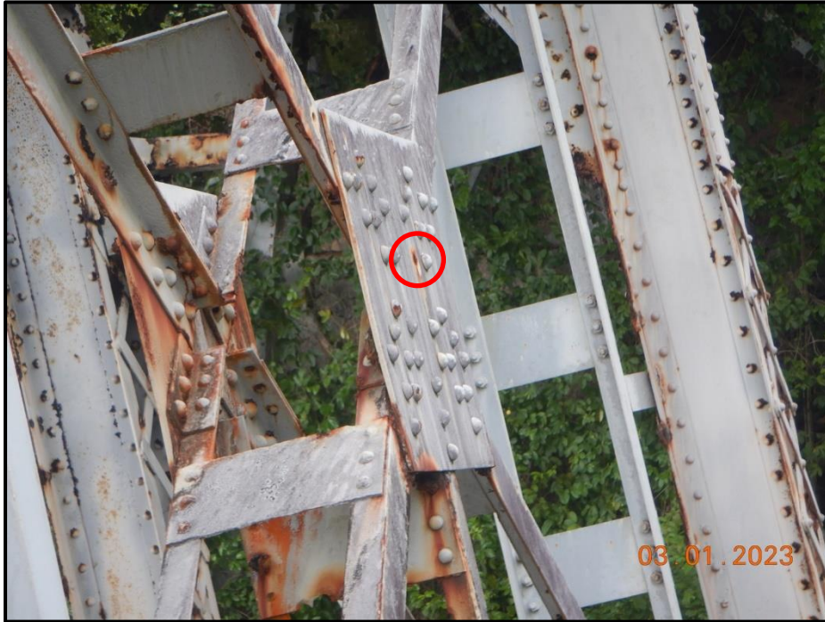
Photograph 71. Tower 2, Level 1, Column D, center gusset plate, looking north. (1) missing rivet, CS3.
