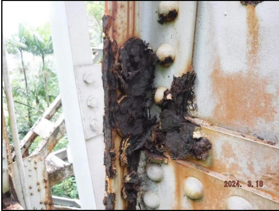
Photograph 119. Bent 7, Level 3, Column B splice plate, looking south. Majority of connection rivets for Column B have section loss and corrosion, CS3.
