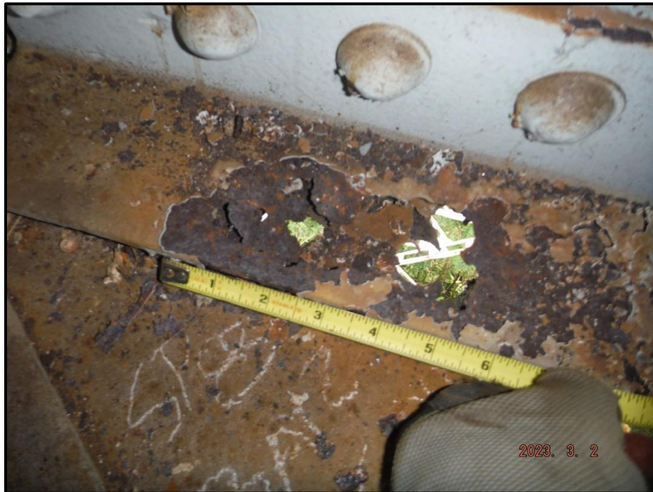
Photograph 28. Span 8, Bay 2, 2nd lower strut, looking south. (2) missing bolts and (1) corrosion hole, 5" L x 2" W.
