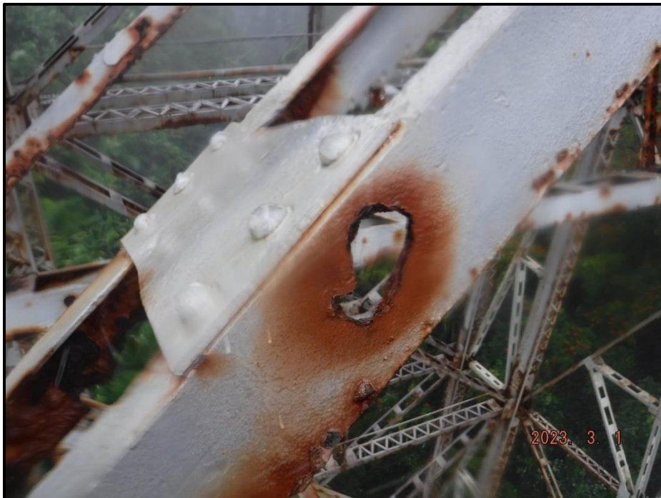
Photograph 92. Tower 3, Level 1, Column A, lower south diagonal bracing, looking west. Several corrosion holes along the west and east angle legs up to 2" diameter, 3' L x 2" H area of 100% section loss on west angle near Bent 4, CS3.
