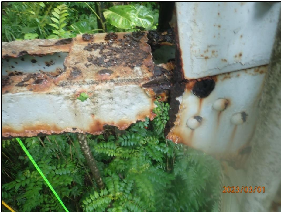
Photograph 149. Bent 7, Level 3, Column A, south horizontal bracing angle, looking north. 3" W x 4" H corrosion hole in vertical angle, CS3.
