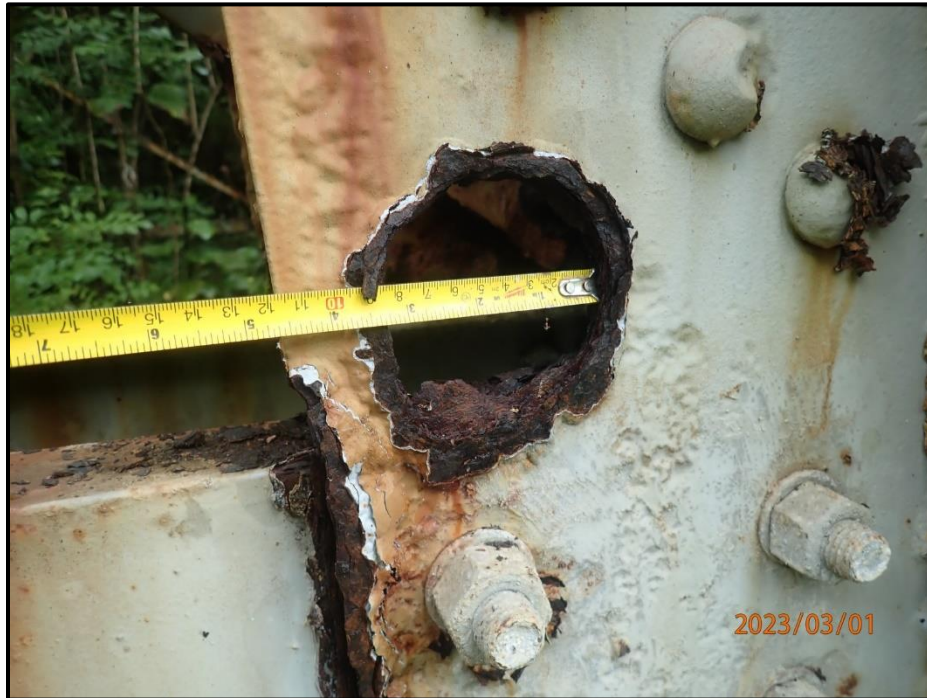
Photograph 130. Bent 6, Level 4, Column B, exterior gusset plate at horizontal bracing, looking south. 3 1/2" diameter corrosion hole, CS3.
