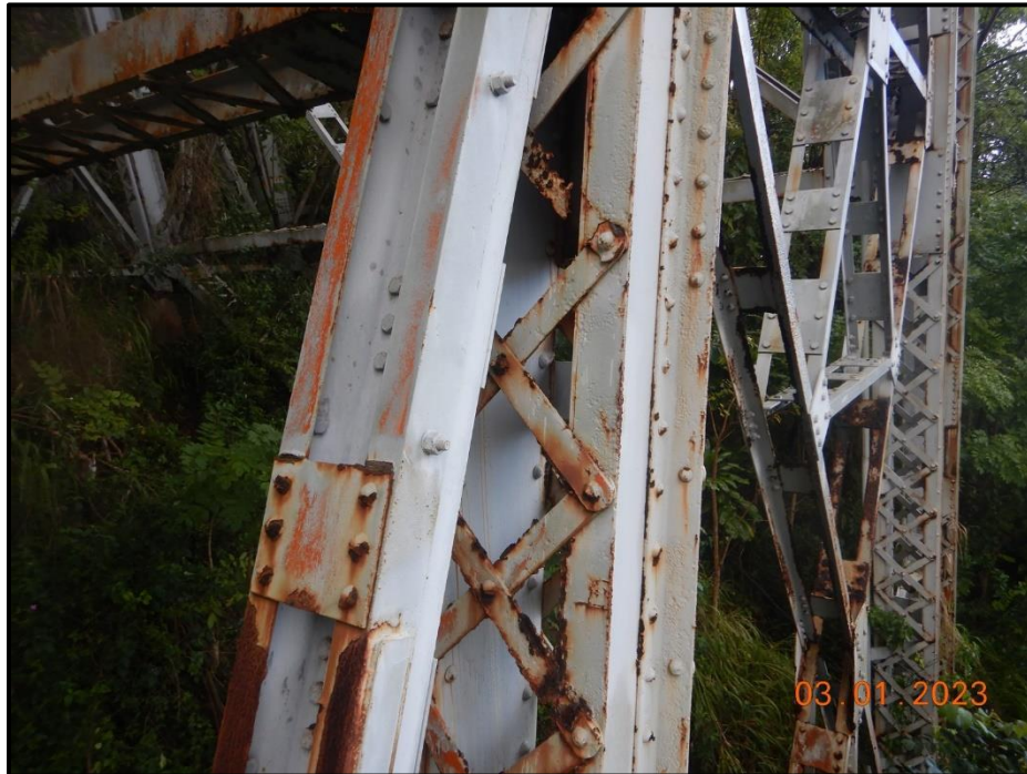
Photograph 154. Bent 8, Level 2, Column C, looking east. (3) lacing bars on west face have 100% section loss. (1) lacing bar on east face has 100% section loss, CS3.
