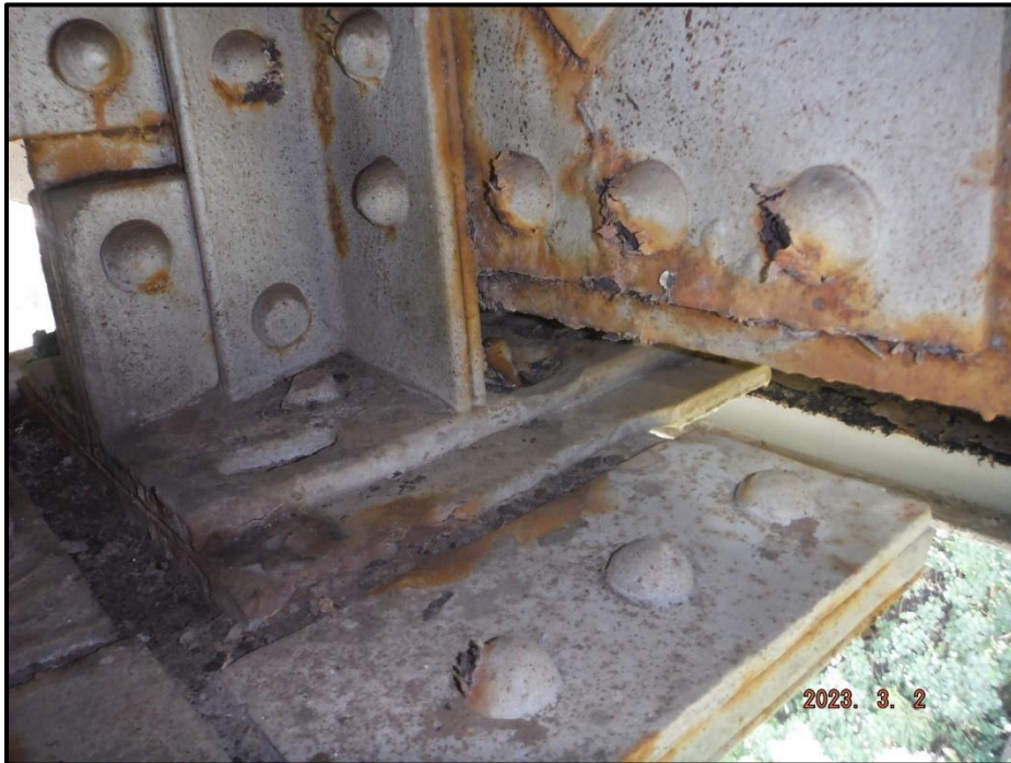
Photograph 49. Bent 7, Span 8, Girder 3 Bearing, looking northwest. Missing southeast, southwest, and northwest anchor bolts, missing northeast anchor nut, CS3.
