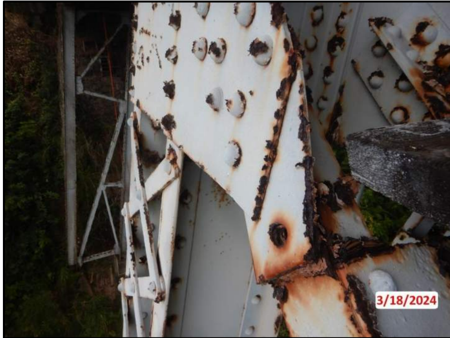
Photograph 21. Tower 2, Level 1, north of Column A, diagonal bracing gusset plate, looking southwest. (1) missing rivet with pack rust up to 1/2" thick, CS3.
