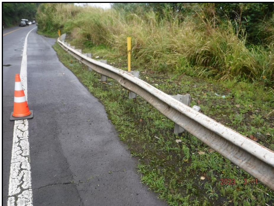
Photograph 54. Northeast guardrail, looking northeast. (2) areas of impact damage, (1) 10' L x 3" deflection and (1) 2' L x 2" deflection.
