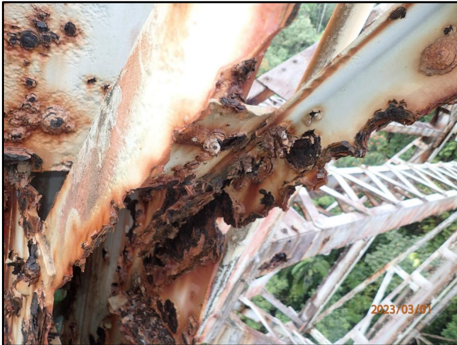
Photograph 87. Bent 4, Level 2, between Columns B and C, lower west diagonal bracing, near Column C, looking northwest. Knife-edging and 80% section loss to the interior angle, CS3.
