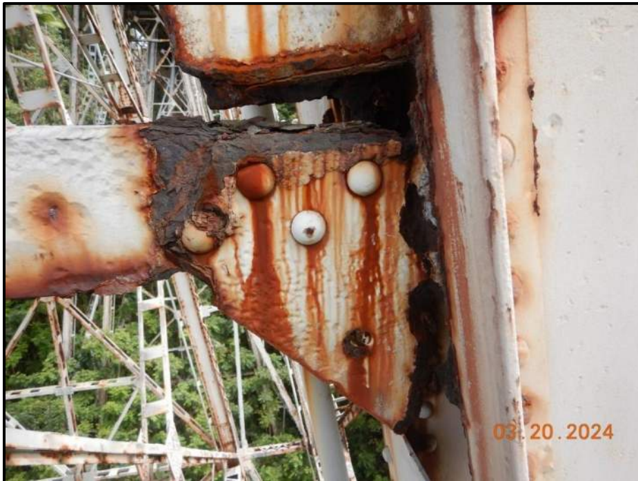
Photograph 72. Bent 5, Level 1, lower section, Column D, horizontal bracing, gusset plate, looking south. North gusset plate has 9" H x up to 3" W area of 100% section loss at connection to Column D, CS4. South gusset plate (6) corrosion holes up to 2" diameter and (1) on north gusset plate, CS3.
