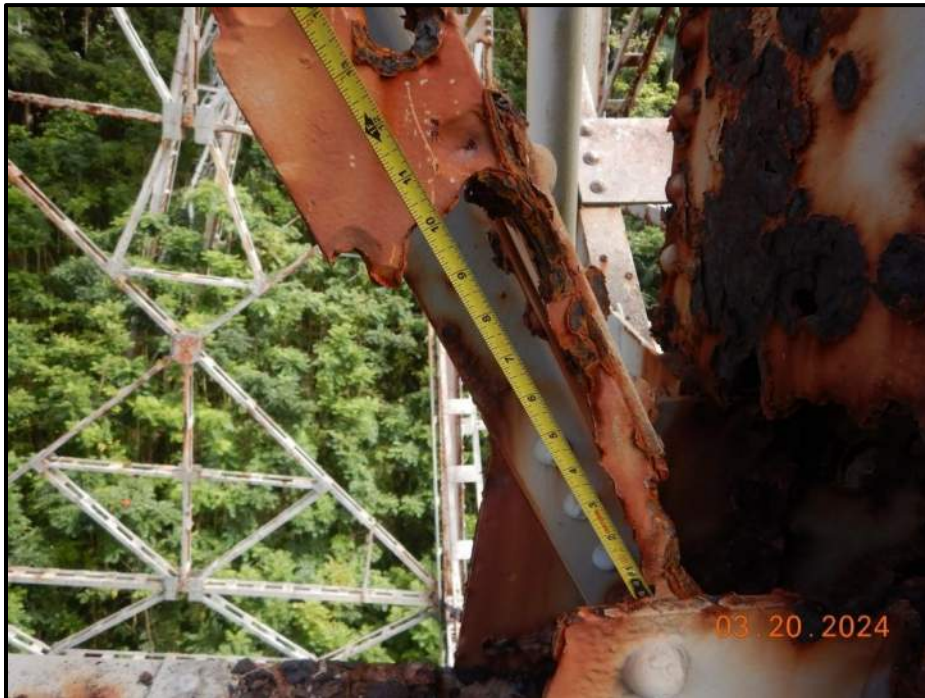
Photograph 74. Bent 5, Level 2, between Columns B and C, lower west diagonal bracing, connection to Column C, looking south. North angle exhibits (2) 10" L x up to 4" H holes with 1" x 3" remaining section. Remaining length of diagonal exhibits knife-edging and pitting, CS4.
