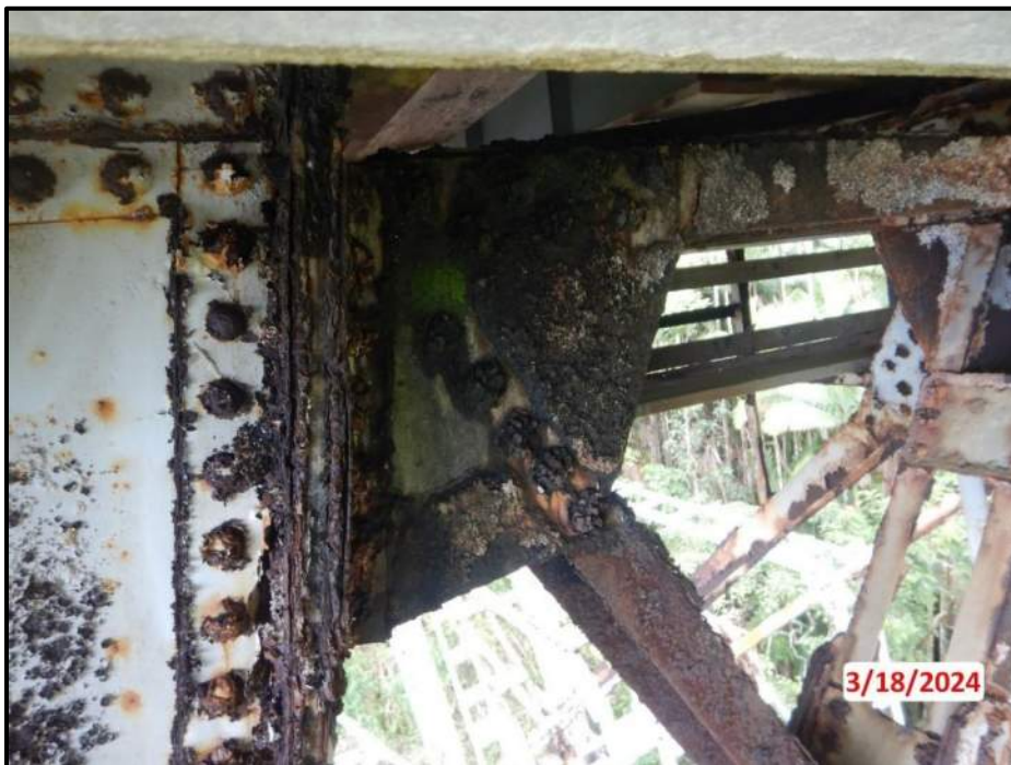
Photograph 34. Bent 3, Level 1, upper section, Column B, top gusset plate and longitudinal bracing, looking southeast. Laminar corrosion and areas of section loss on members and rivet heads due to active water leakage from the bridge, CS3.
