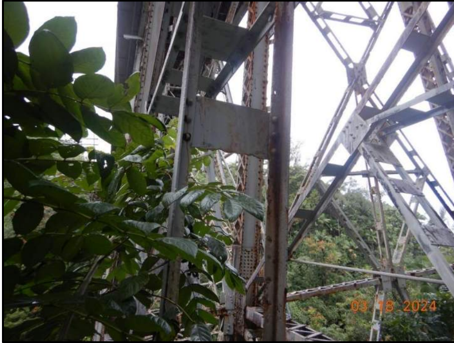
Photograph 31. Tower 2, Level 2, Column D, vertical bracing, looking north. Up to 1/8" deep pitting with scattered areas of knife-edging, CS3.
