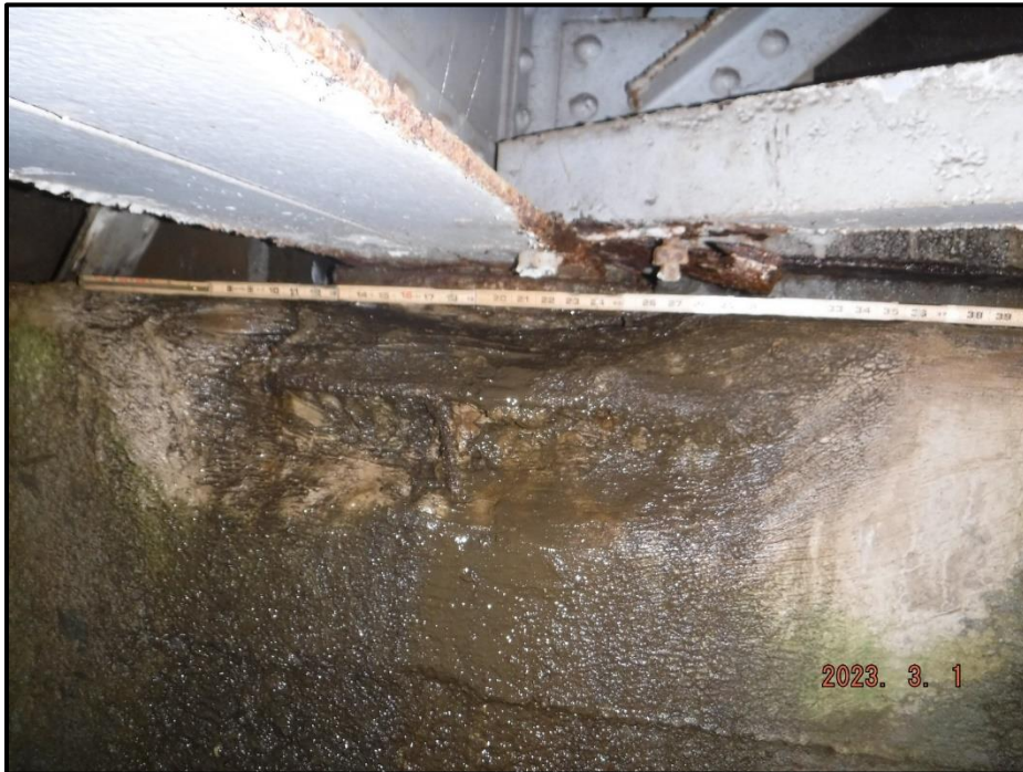
Photograph 43. North Abutment, Girder 3 seat, looking north. Failed repair, 2' 11" L x 10" H x 3" deep exposing (2) reinforcing bars with no section loss, CS3.
