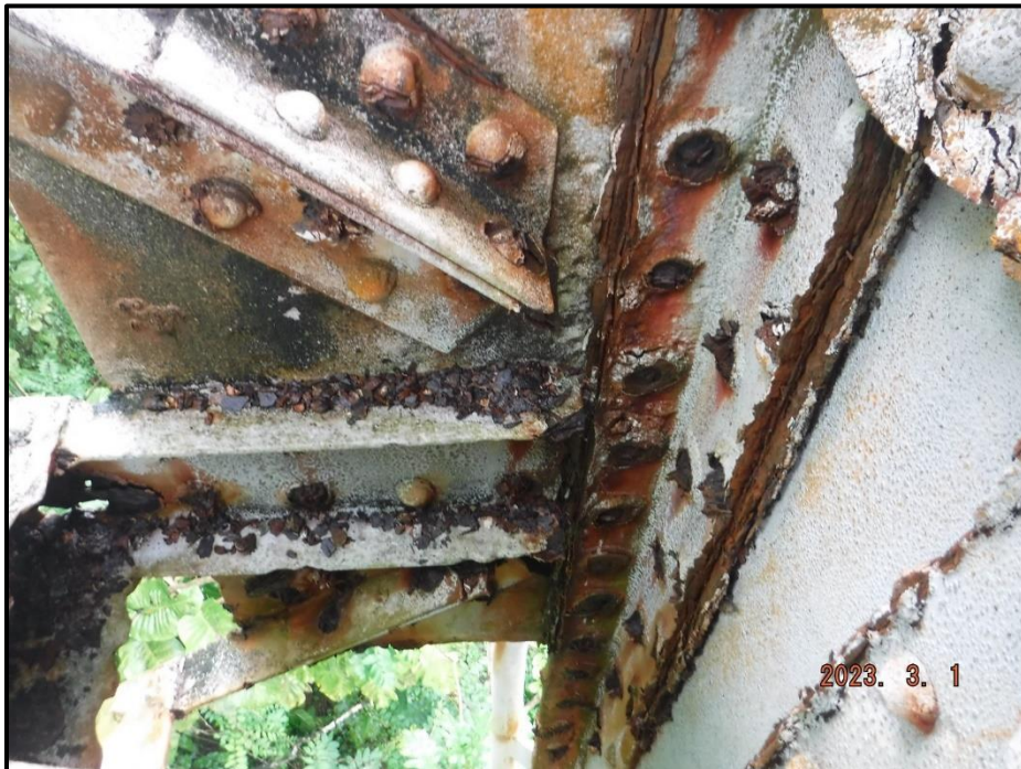
Photograph 137. Tower 4, Level 3, Column C, gusset plate connecting bracing to Bent 6, looking east. 14 of 18 rivet heads connecting the gusset plate to the column have 20% remaining on the inside face. East channel of bracing has more severe section loss at this location with five corrosion holes in the web up to 1" diameter, CS4.
