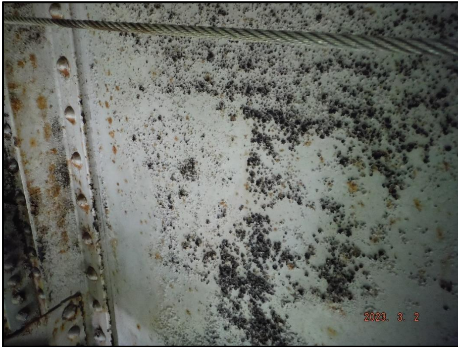
Photograph 41. Span 5, Bent 4, Girder 2, looking west. Steel protective coating exhibits peeling/ bubbling, CS3.
