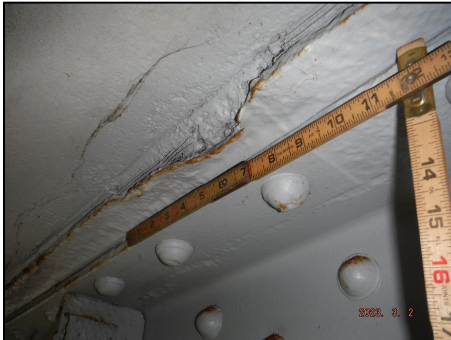
Photograph 30. Span 2, Bay 1, top flange plate of Girder 1, looking northeast. Intermittent areas of up to 2' L x 2" W x 1/2" deep painted over pitting, CS3.
