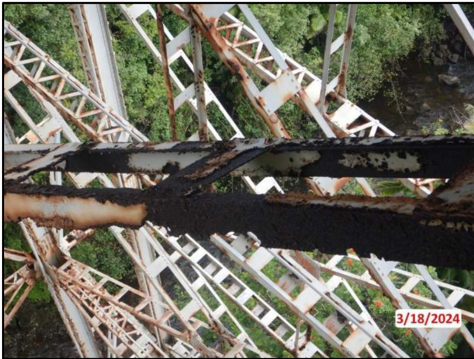
Photograph 66. Tower 3, Level 1, Column C, upper south to lower north diagonal bracing, looking northeast. Up to 6" L x 2" H corrosion holes with knife edging throughout both angles, CS3.
