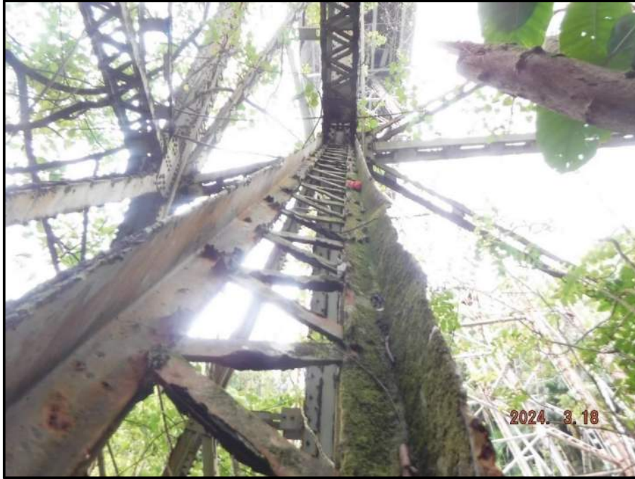
Photograph 105. Tower 4, Level 5, Column B, mid-diagonal bracing, interior angle, looking south. Twisted over full length with deformation up to 6" over 2' 6", CS3.
