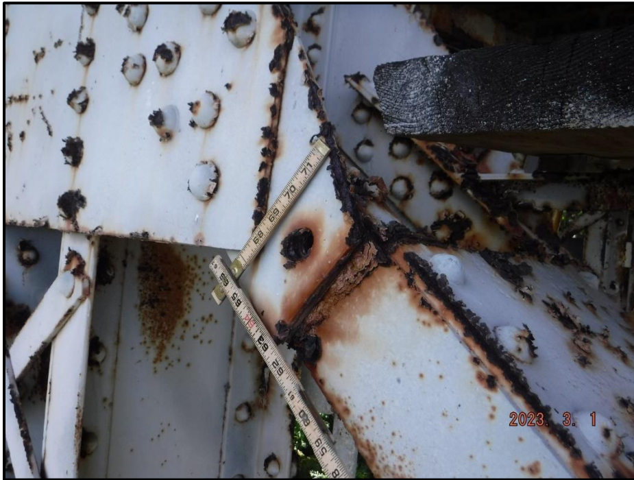
Photograph 67. Tower 2, Level 1, Column A, Bent 2, gusset plate to diagonal connection, looking west. (1) missing rivet with pack rust up to 1/2" thick, CS3.
