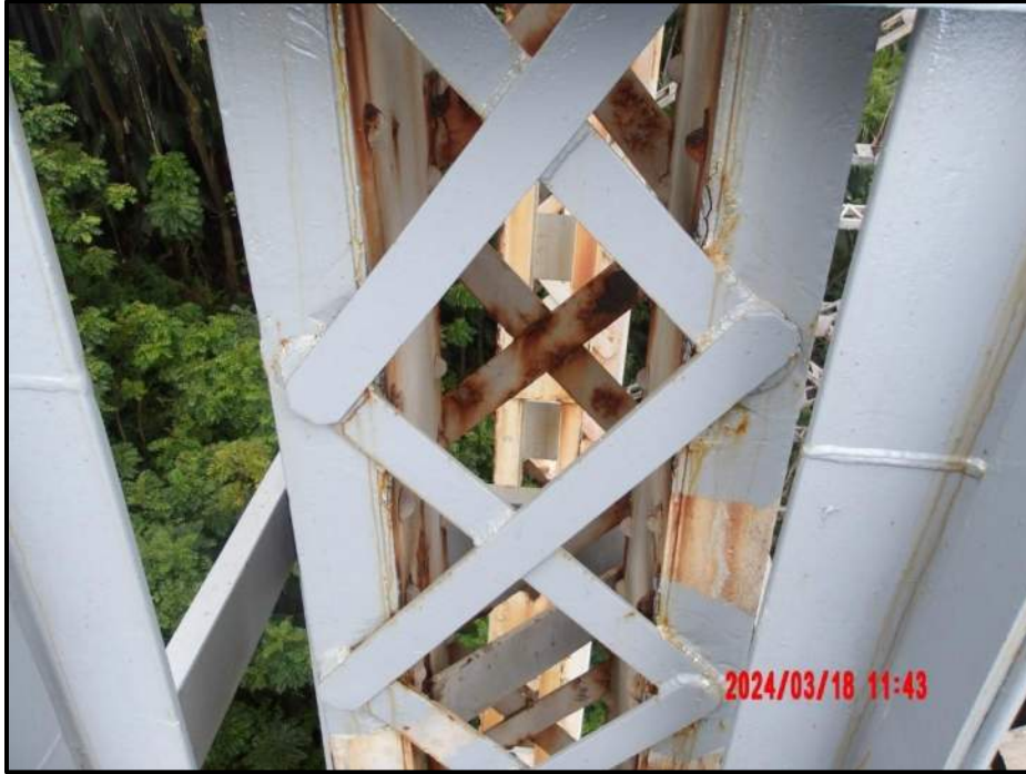
Photograph 51. Bent 4, Level 3, Column A above lower connection, looking west. Retrofit, four interior and three exterior lacing bars cut or removed, (CS3). - Repaired.
