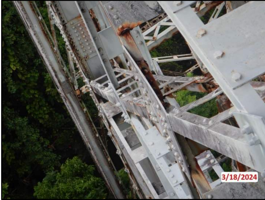
Photograph 29. Tower 2, Level 1, Column D, center west gusset plate, looking north. (1) missing rivet, CS3.
