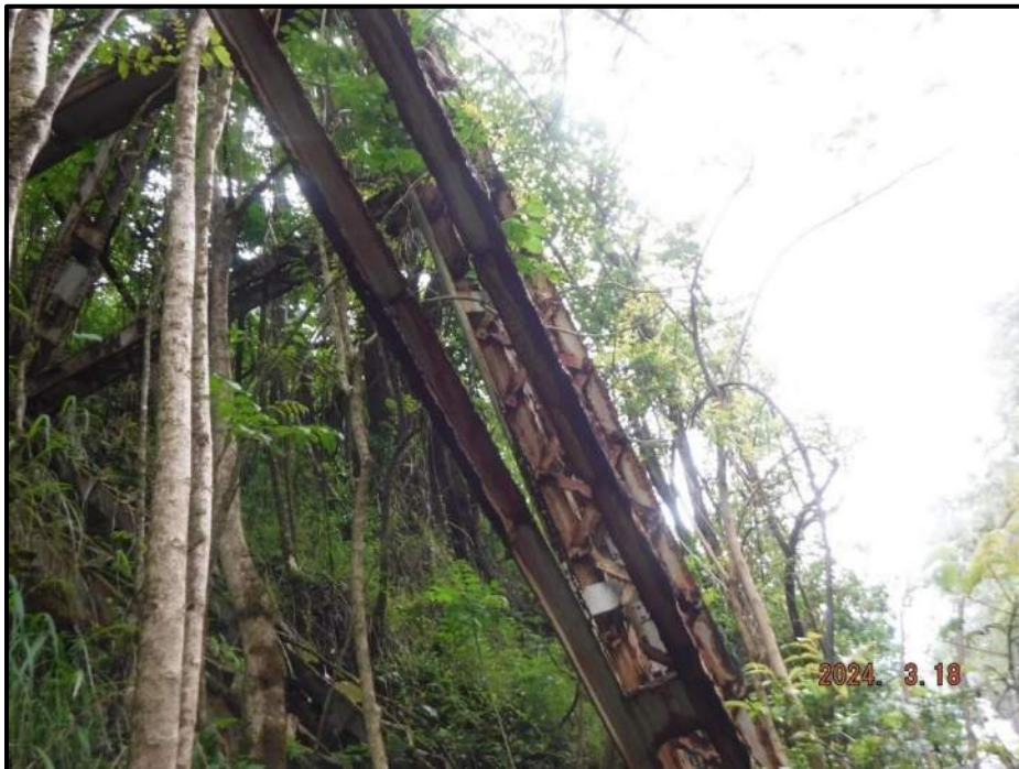
Photograph 98. Bent 6, Level 6, between Columns B and C, lower east diagonal at third point closest to Column B, looking east. Missing batten plate, CS3.
