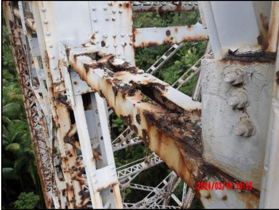
Photograph 47. Bent 4, Level 1, lower section, between Columns A and B, horizontal bracing, looking west. Vertical legs have knife-edging with areas of up to 100% section loss and corrosion holes up to 1" diameter. (1) lacing bar has 100% section loss and batten plate has area of 100% loss, CS3.
