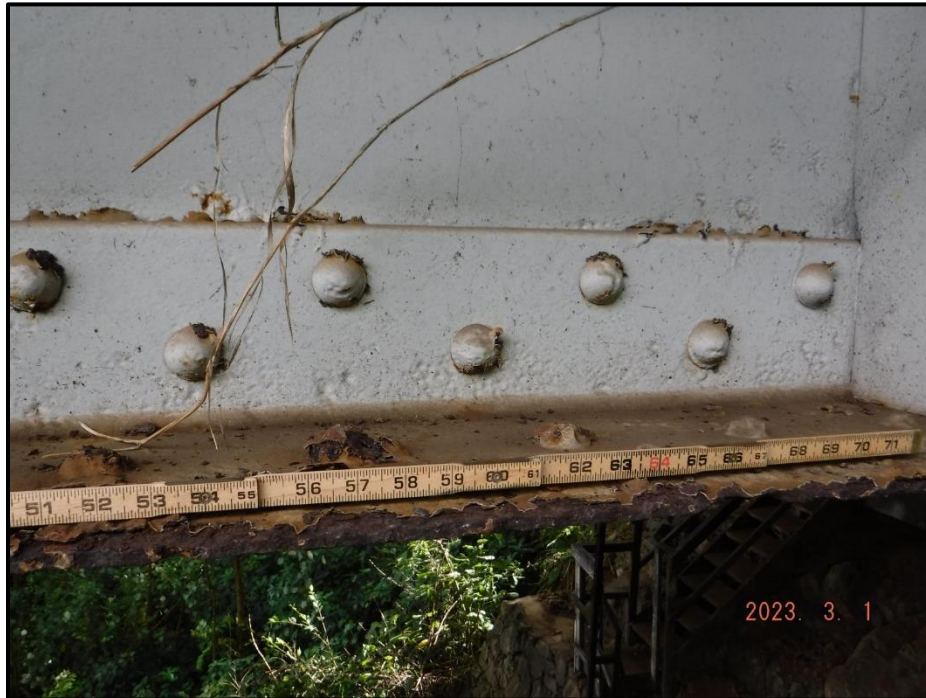
Photograph 29. Span 1, Girder 4 bottom flange (top and bottom faces), at midspan, looking east. Typical peeling paint and moderate corrosion along the ends of all exterior girders , typically 4' L x 5' W, with up to 3/16" deep section loss, CS3.
