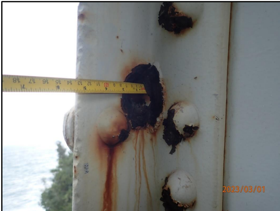
Photograph 145. Bent 7, Level 1, lower section, Column A, looking southeast. 2" diameter corrosion hole in northeast flange angle, CS3.
