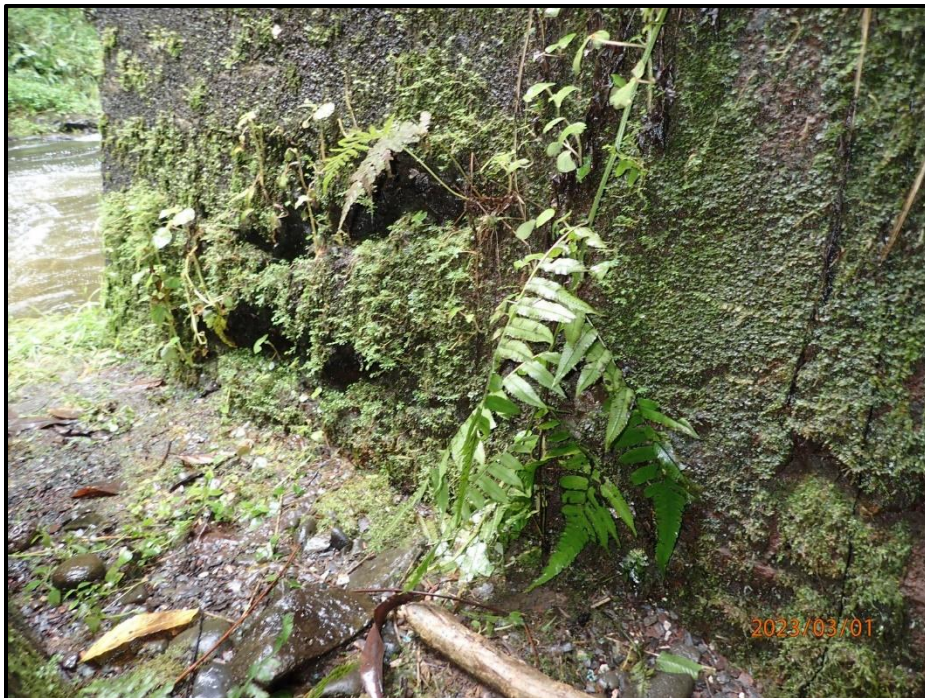
Photograph 117. Bent 5, Level 6, Column C, footing, base of pedestal on west side, looking northeast. 3' x 2' abrasion with course aggregate exposed and missing, CS3.
