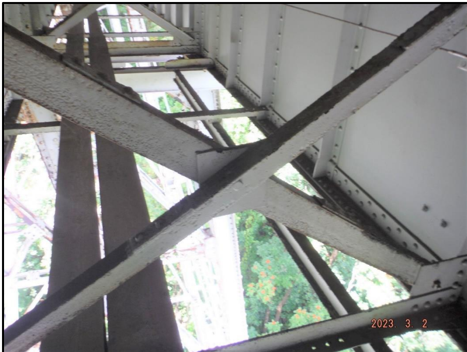
Photograph 26. Span 6, Bay 1, near Bent 6, looking north. Cross frames typically have painted over pitting 1/16" D with isolated areas up to 1/4" D and areas of reactivating corrosion.
