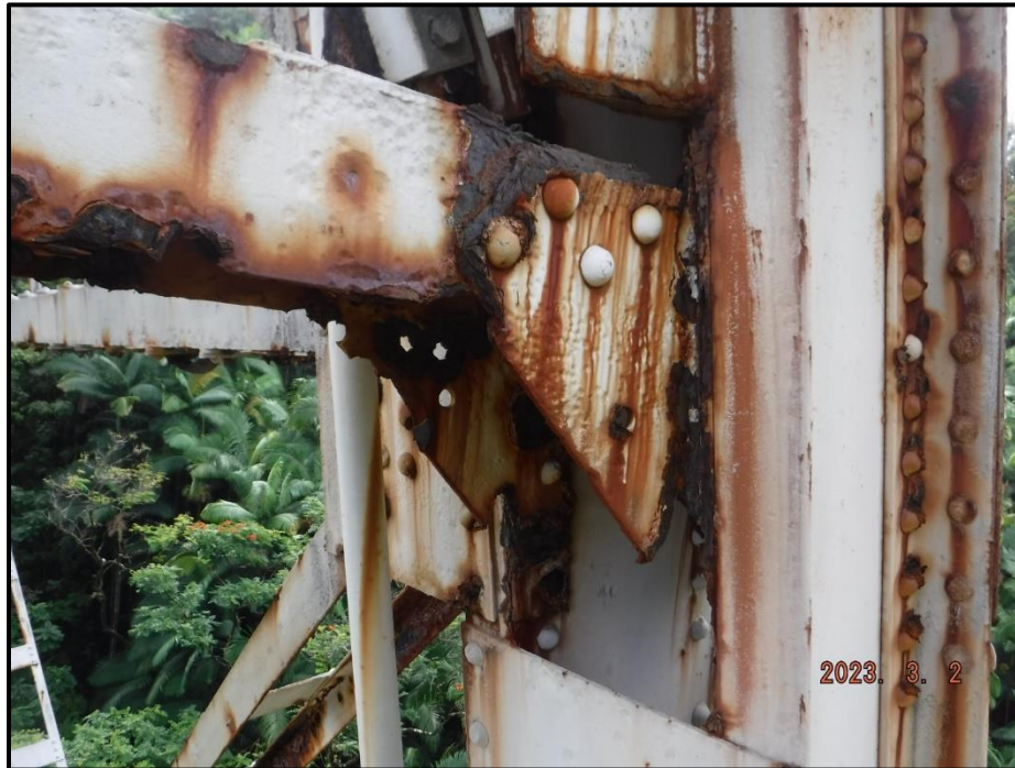
Photograph 108. Bent 5, Level 1, lower section, Column D, horizontal bracing, gusset plate, looking south. North gusset plate has 8" L area of 100% section loss at connection to Column D, CS4. South gusset plate (4) corrosion holes up to 2" diameter and (1) on north gusset plate, CS3.
