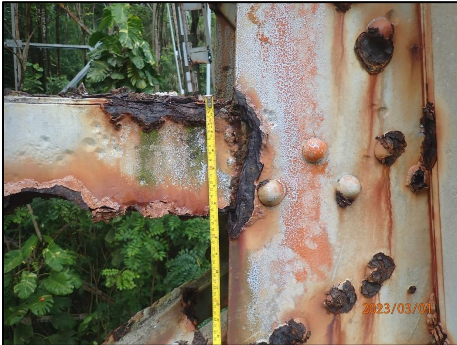
Photograph 126. Bent 6, Level 3, Column B, south gusset plate, west side, looking east. 1 1/2" W x 8" H area of 100% section loss, CS3.
