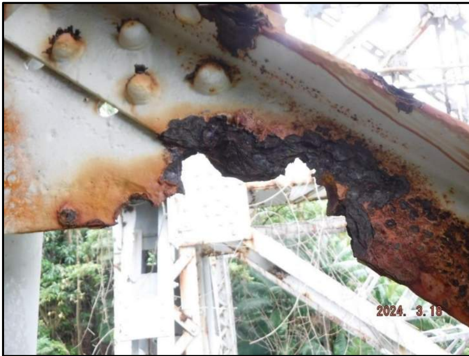
Photograph 24. Tower 2, Level 2, Column A, upper south diagonal and gusset plate at Column A connection, looking west. Interior angle, 8" L x 3" W area of 100% section loss, CS3.
