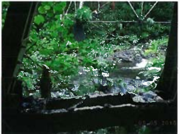
Column 6 bottom brace has corrosion and missing lacings.
