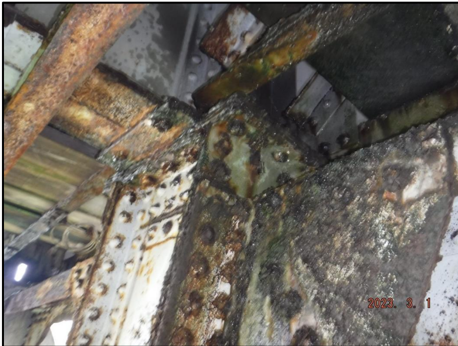
Photograph 46. Bent 3 Joint, Bay 2, looking southeast. Active leakage, CS3.
