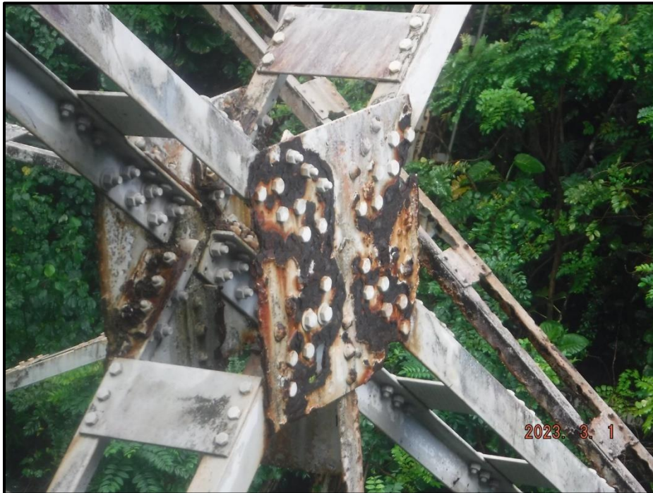
Photograph 99. Tower 3, Level 4, Column B, center gusset plate, looking southwest. Numerous corrosion holes on both gusset plates, CS3.
