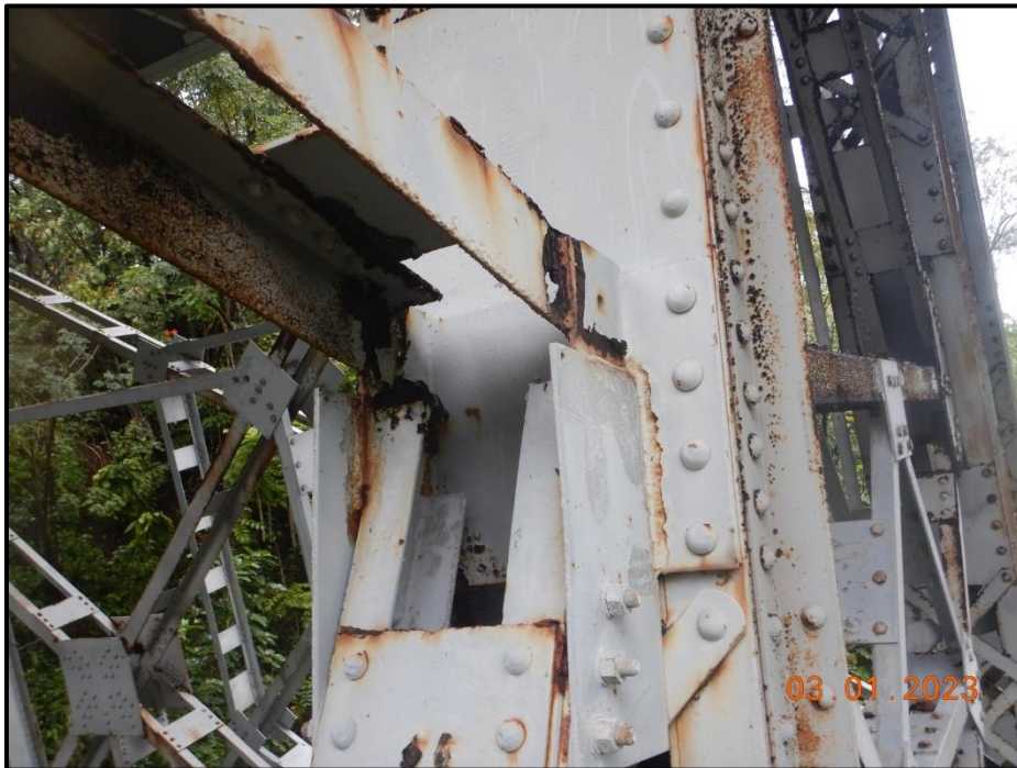
Photograph 151. Bent 8, Level 1, upper section, Column C, lower horizontal bracing, looking northeast. South angle has 3" H x 1" W corrosion hole adjacent to the gusset plate, CS3.
