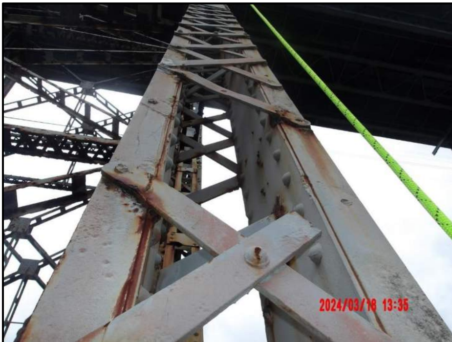
Photograph 76. Bent 5, Level 3, Column A, (9) lacing bars, looking west. Removed from column, CS3.
