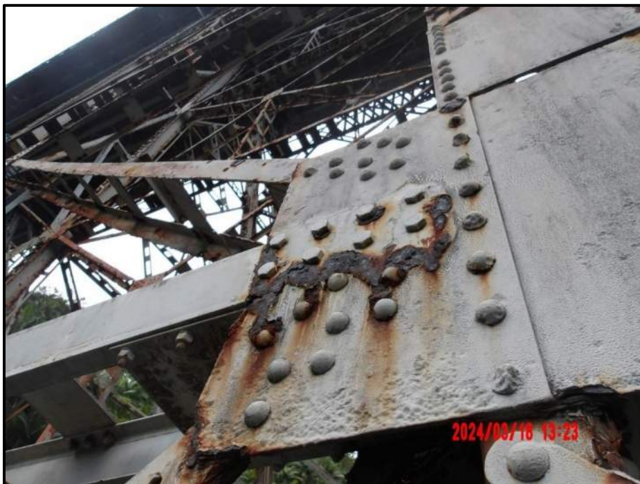
Photograph 64. Tower 3, Level 3, Column A, Bent 5, interior and exterior gusset plates, between horizontal and lower diagonal bracing, looking west. Pack rust with section loss, CS3.
