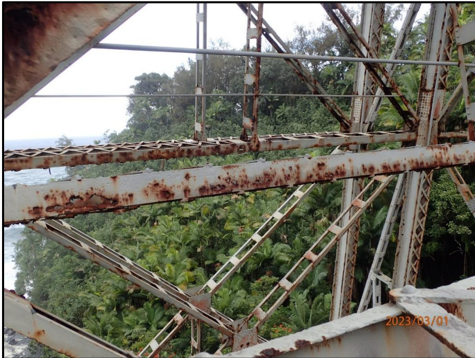
Photograph 101. Tower 3, Level 1, Column C, lower horizontal bracing, looking east. Multiple corrosion holes up to 6" diameter in east and west channels, CS3.
