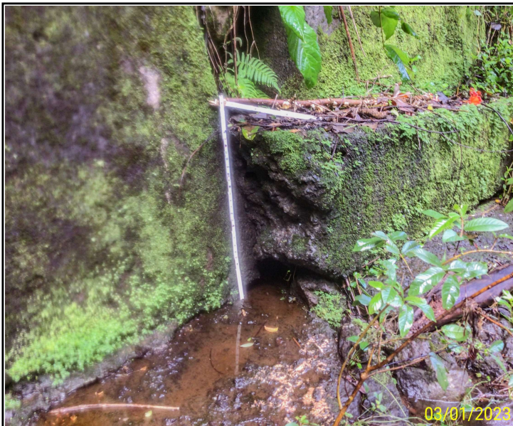
Photo 15. Bent 6, Column A Footing, looking north. Void below southwest corner, 8" L x 6" H x 9" D, CS2
