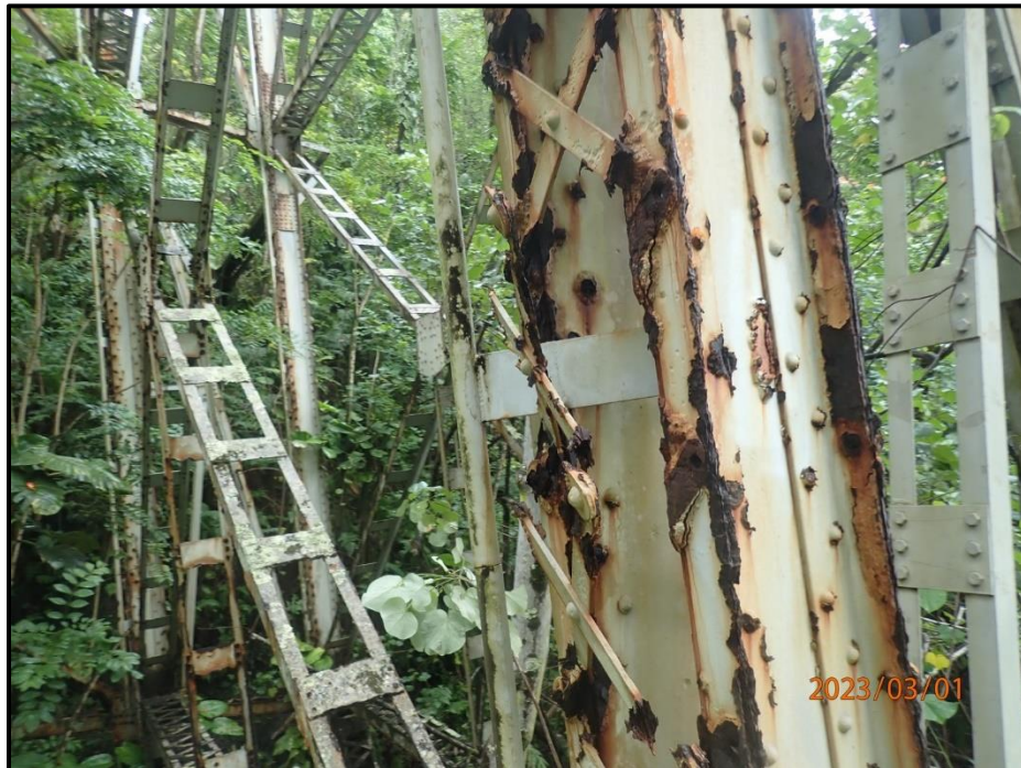
Photograph 131. Bent 6, Level 5, Column B, looking northeast. Almost all lacing bars on the west side of the column have 100% section loss; (6) bars with section loss remaining intact at time of inspection, CS4.
