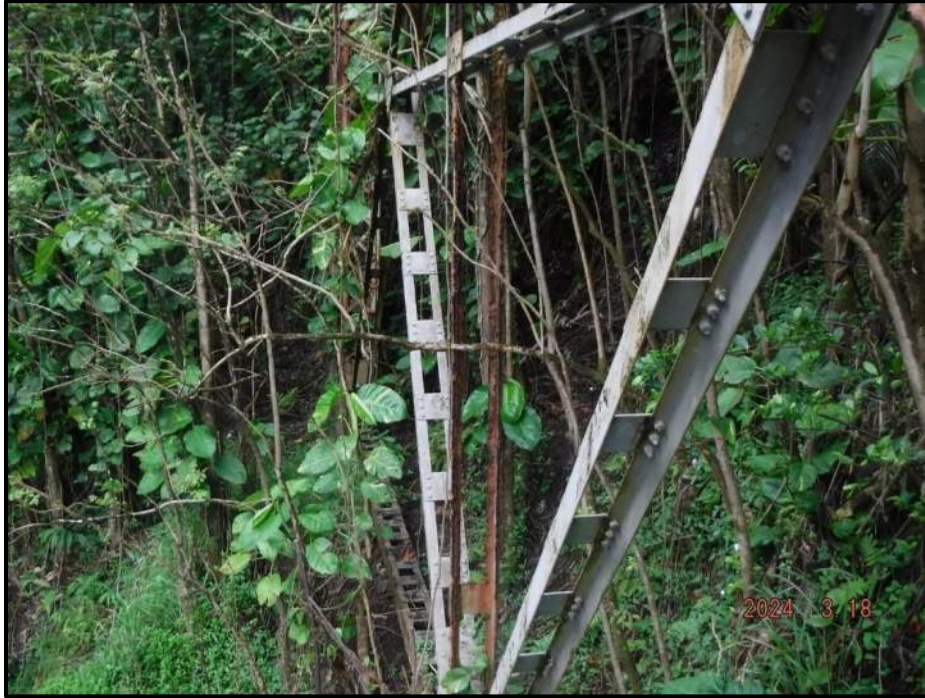
Photograph 99. Bent 6, Level 6, between Columns B and C, mid-length vertical bracing above crossing horizontal, looking west. Detached batten plate, CS3.
