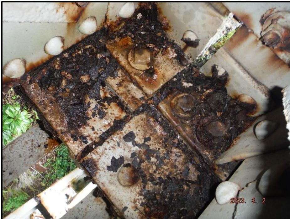
Photograph 50. Bent 9, Span 9, Girder 1 bearing, looking east. Up to 1/4" thick laminar corrosion, CS3.
