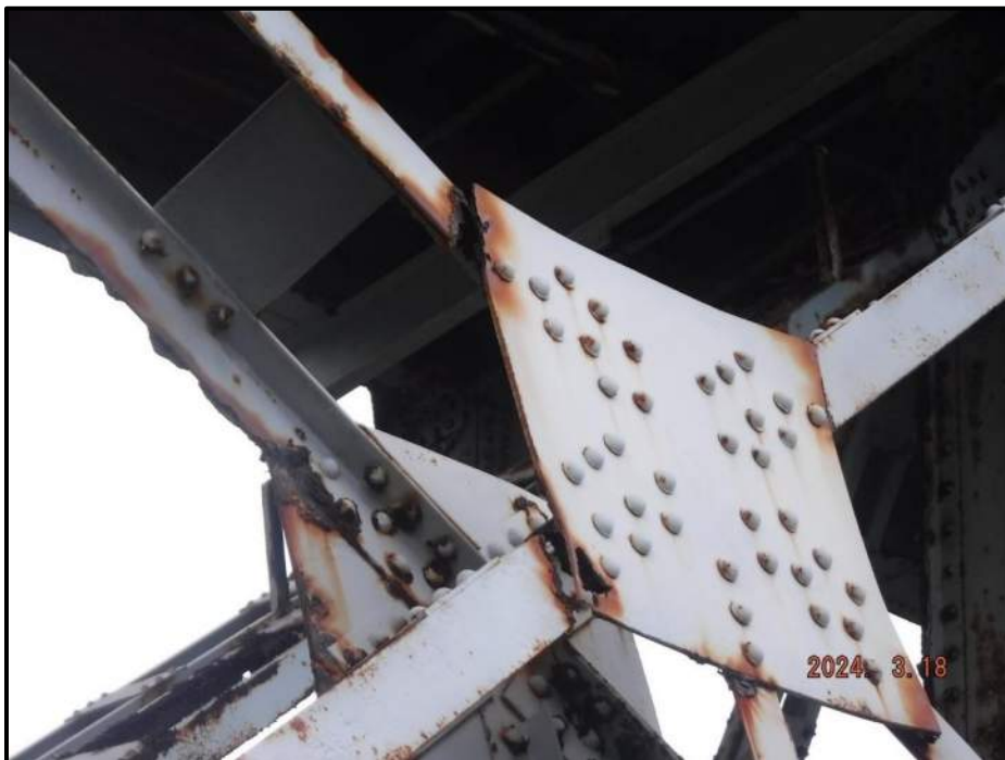
Photograph 100. Tower 4, Level 1, Column B, lower south diagonal bracing, looking northwest. Exterior angle of diagonal has 100% section loss to vertical leg and only 2-1/2" of section remaining on horizontal leg; angle is deformed 1/4" over 10" near section loss; gusset plate has 3" diameter corrosion hole, CS4.
