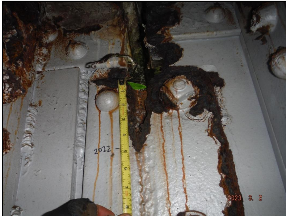
Photograph 35. Bent 3, Girder 1, top of sliding web plate, looking east. 5" H x 2" W area of 1/8" to 100% section loss, area of 100% loss is 1" W, CS3.
