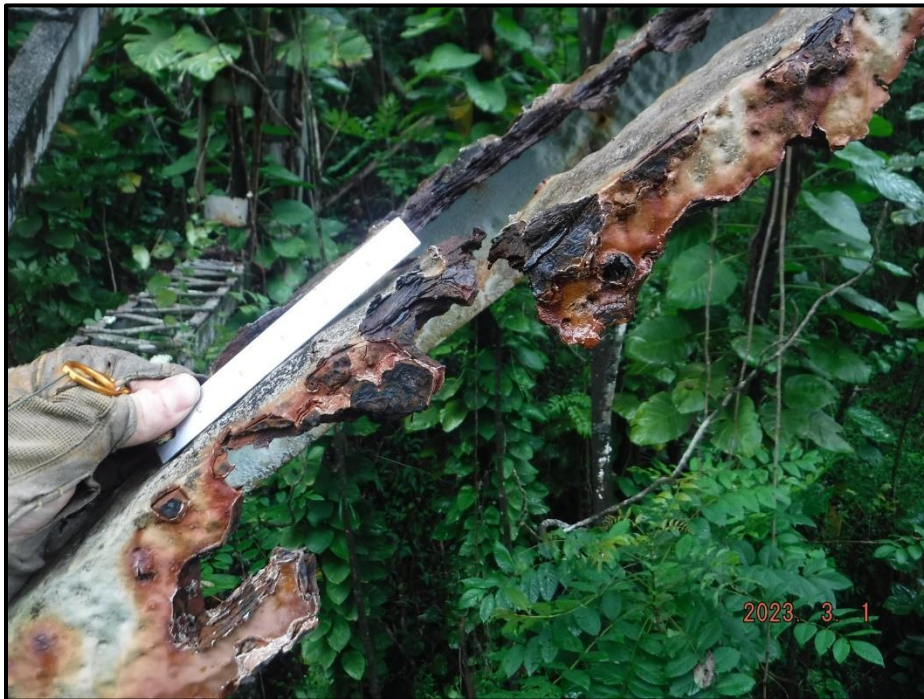
Photograph 127. Bent 6, Level 4, between Columns B and C, lower west diagonal adjacent to Column C, looking north. Corrosion holes and knife edging at exterior vertical flange and section of missing vertical flange at lower end for 1' 6" L, CS3.
