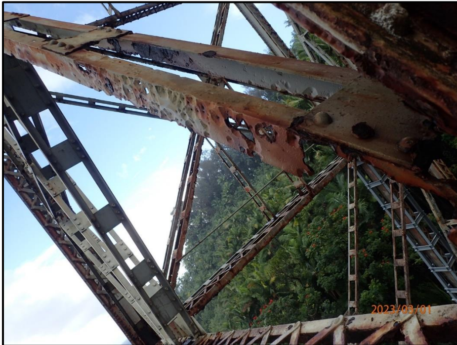
Photograph 109. Bent 5, Level 2, between Columns B and C, lower west diagonal bracing, connection to Column C, looking south. North angle exhibits two 10" L x up to 4" H holes with 1" x 3" remaining section. Remaining length of diagonal exhibits knife-edging and pitting, CS4.
