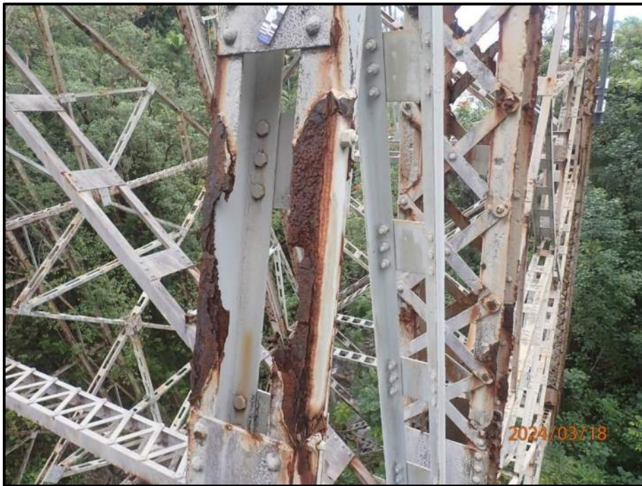
Photograph 52. Bent 4, Level 3, between Columns C and D, diagonal bracing, looking northeast. 3' L x full width of angle area of up to 100% section loss to top flanges, CS3. -Note this member has been retrofitted and retrofit is in good condition.
