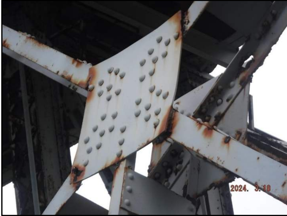
Photograph 101. Tower 4, Level 1, Column B, upper north diagonal bracing, looking southwest. Interior angle of diagonal has 3" diameter corrosion hole in vertical leg of angle at connection, CS4.
