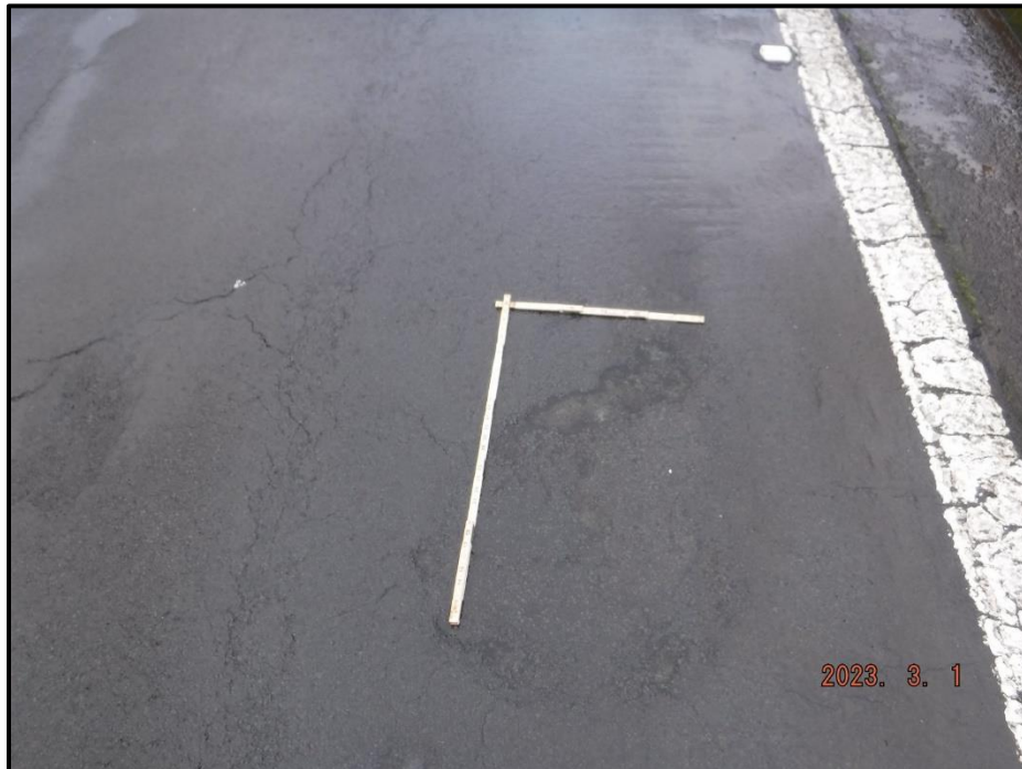
Photograph 20. Span 8, NB lane, 15' north of Bent 7 joint, looking north. 8" L x 1' 3" W x 1/2" deep patched pothole that is failing and has ponding water, CS3.
