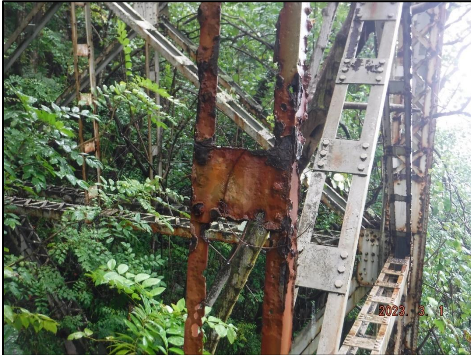
Photograph 128. Bent 6, Level 4, between Columns B and C, vertical bracing, looking north. Severe corrosion throughout this member with 40% section remaining, CS4.
