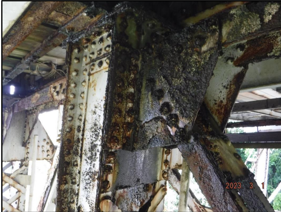
Photograph 75. Bent 3, Level 1, upper section, Column B, top gusset plate and longitudinal bracing, looking southeast. Laminar corrosion and areas of section loss on members and rivet heads due to active water leakage from the bridge, CS3.
