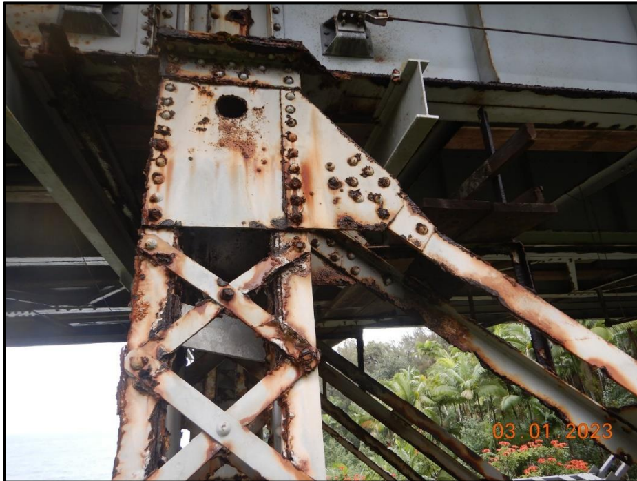
Photograph 77. Bent 3, Level 1, upper section, Column D, vertical near top, looking north. Typical laminar corrosion at upper levels, CS3.
