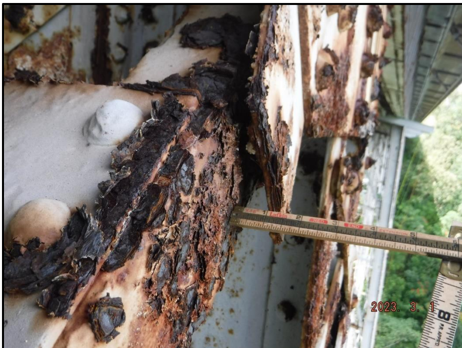
Photograph 66. Tower 2, Level 1, Column A , upper north diagonal bracing, near Bent 3, looking north. 6" x 2" corrosion hole in vertical leg of interior angle near Column A connection. Exterior leg has area of pack rust causing separation of gusset plate up to 1", CS3
