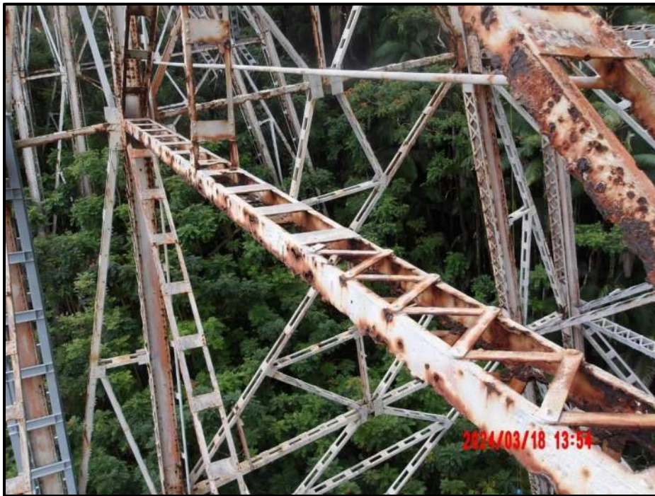
Photograph 62. Tower 3, Level 2, Column B, horizontal bracing, looking southwest. Numerous corrosion holes, up to 6" L x 3" H throughout full length of both channels, CS3.
