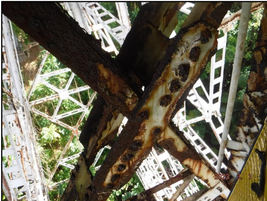
Photograph 76. Bent 3, Level 1, upper section, between Columns B and C, center gusset plates, looking south. Laminar corrosion on plates and transverse bracing members, CS3.
