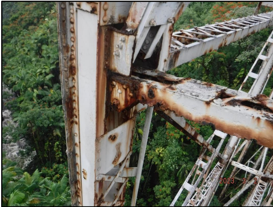
Photograph 85. Bent 4, Level 1, lower section, Column D, lower gusset plates, looking northwest. Pack rust up to 1" thick with areas of 100% section loss and only retrofit gusset plate remaining, no change from previous inspection, CS3.
