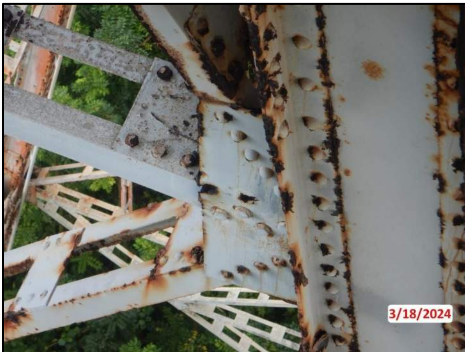
Photograph 70. Bent 5, Level 1, upper section, Column C, north gusset plate, looking southeast. (1) 1" diameter and (1) 2" diameter corrosion hole, CS3.
