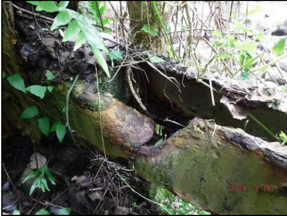
Photograph 97. Bent 6, Level 6, between Columns A and B, horizontal bracing, looking northeast. Damage, member impacted by falling rocks, CS3.
