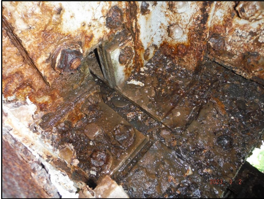
Photograph 33. Bent 3, Bay 1, Girder 1 and 2 bottom flange connection, looking northwest. Rivet heads have corrosion with up to 50% section loss, CS3.
