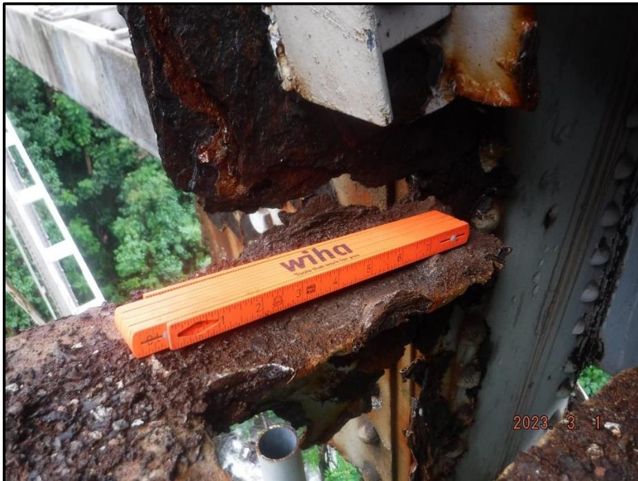
Photograph 90. Bent 4, Level 3, horizontal bracing at gusset plates at Column A, looking north. Horizontal bracing gusset plate has 100% section loss on all sides. This member is not connected to Column A anymore, CS4.
