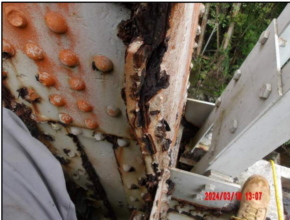
Photograph 78. Bent 5, Level 4, Column B, vertical at southeast flange splice, looking north. Column is deformed, 1' 10" L x 1" deflection, CS3.
