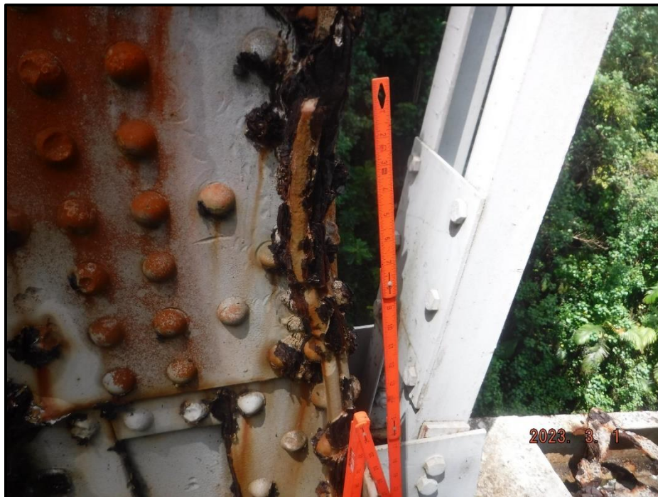
Photograph 115. Bent 5, Level 4, Column B, vertical at southeast flange splice, looking north. Column is deformed, 1' 10" L x 1" deflection, CS3.
