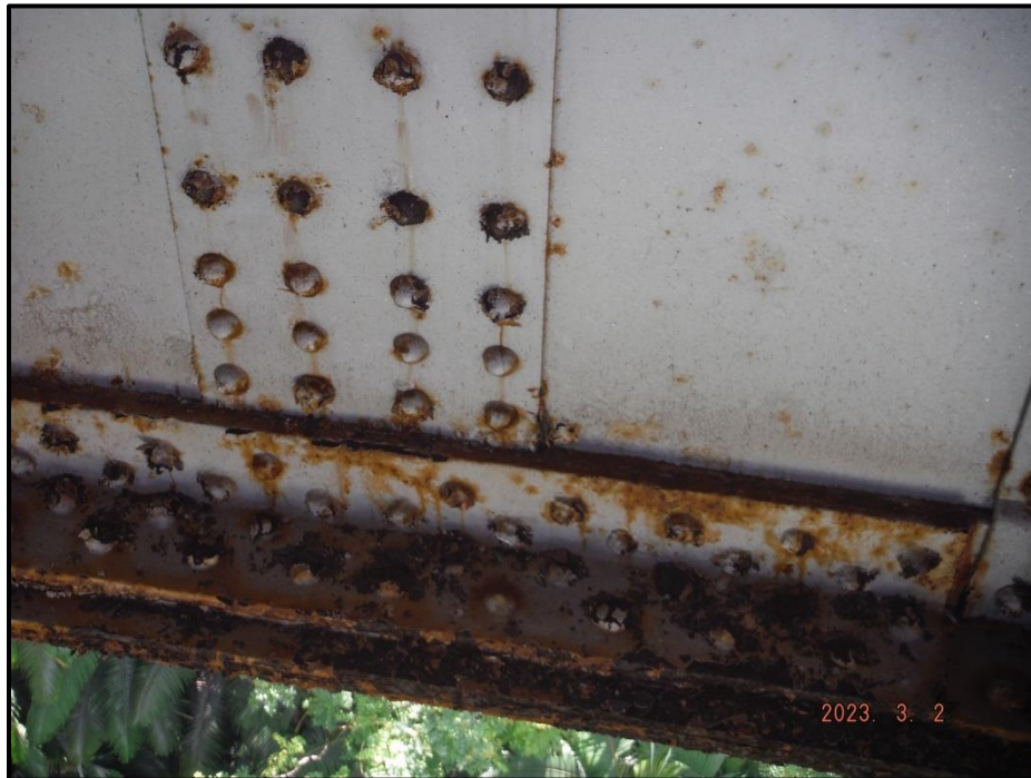
Photograph 36. Span 4, Girder 3 splice and bottom flange, looking west. 3' L x up to 1/8" W pitting and rivet head corrosion with up to 25% section loss, as well as peeling paint, CS3.
