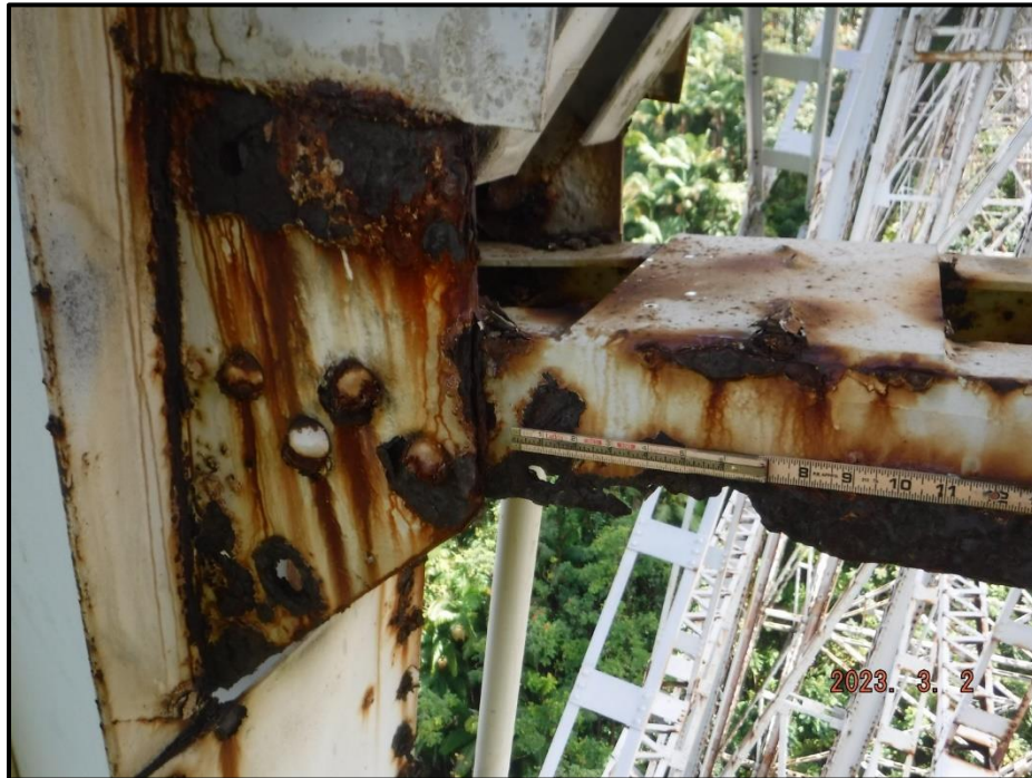
Photograph 142. Bent 7, Level 1, upper section, Column A, gusset plate, looking south. (2) corrosion holes up to 1" diameter and horizontal bracing connection to Column B has a 5" L x 1" H area of 100% section loss.
