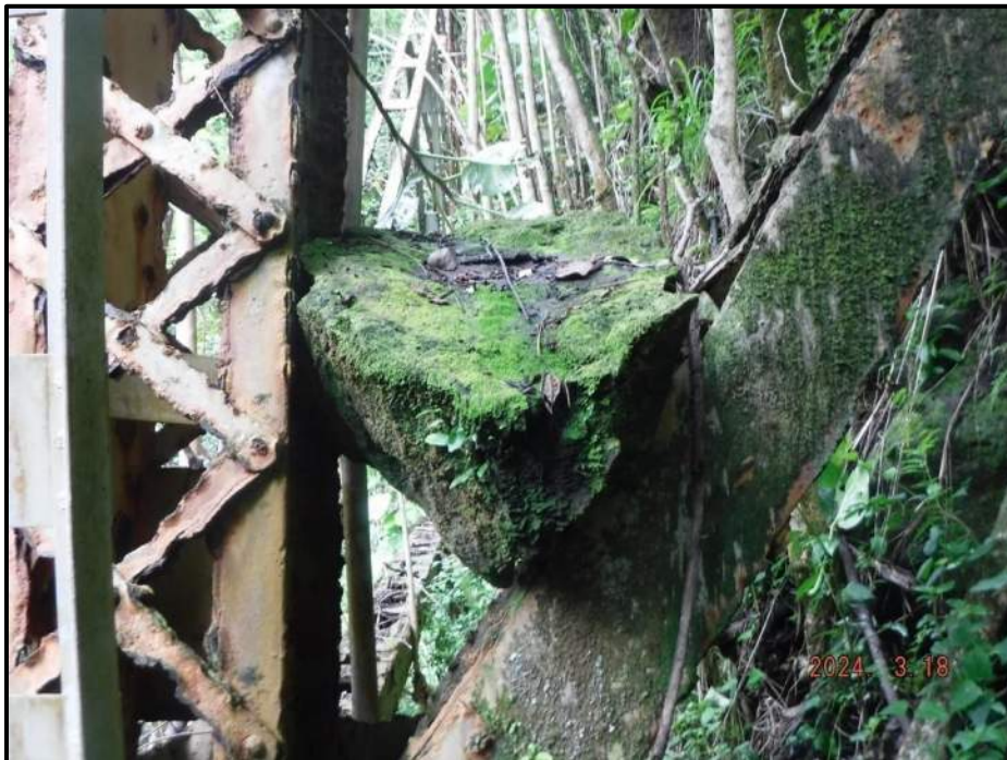
Photograph 106. Tower 4, Level 6, Column B, looking west. 3' diameter boulder on top of diagonal member at bottom connection; member appears to be deformed as a result.
