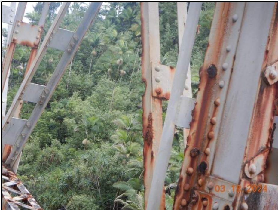
Photograph 86. Bent 6, Level 2, between Columns B and C, lower west diagonal bracing near Column C, north angle vertical leg, looking southeast. Corrosion hole, 3" L x 2" H, CS3.
