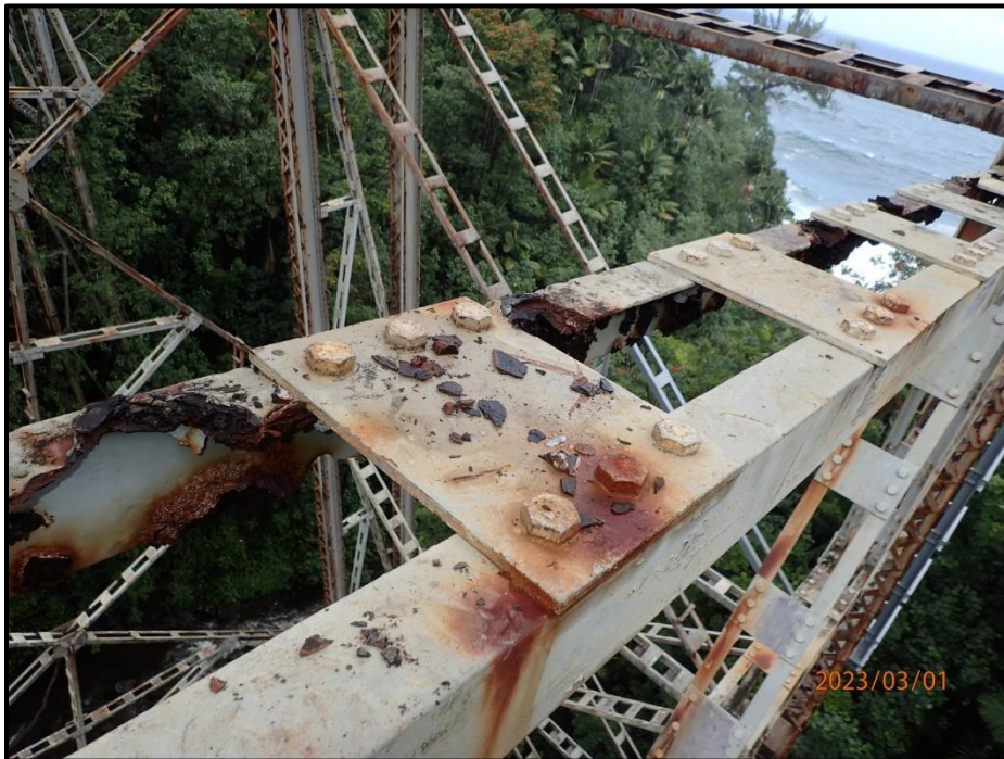
Photograph 86. Bent 4, Level 2, between Columns B and C, horizontal bracing adjacent to Column C, vertical connection, looking northeast. (7) 2" diameter corrosion holes in interior top flange along member, CS3.
