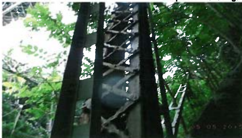
Center up right brace between bent 6 and 7 has corrosion on lacings.
