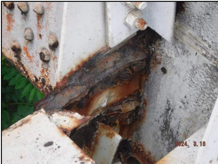
Photograph 42. Bent 3, Level 2, between Columns A and B, horizontal bracing, south flange, horizontal leg, looking north. 9" L x full-width of angle area of 100% section loss, CS3.
