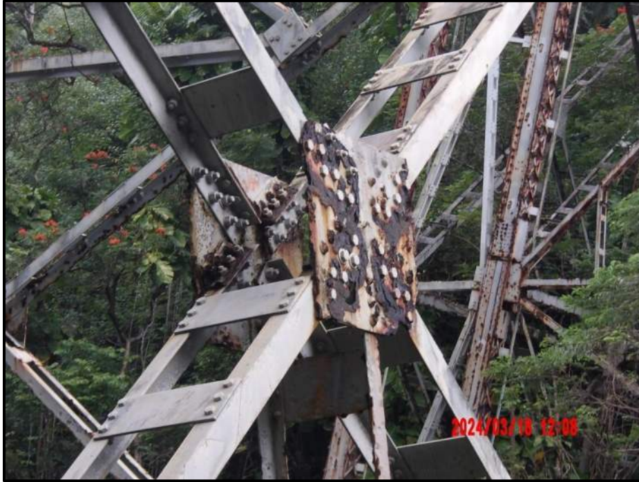
Photograph 65. Tower 3, Level 4, Column B, center gusset plate, looking northwest. Numerous corrosion holes on both gusset plates, CS3.
