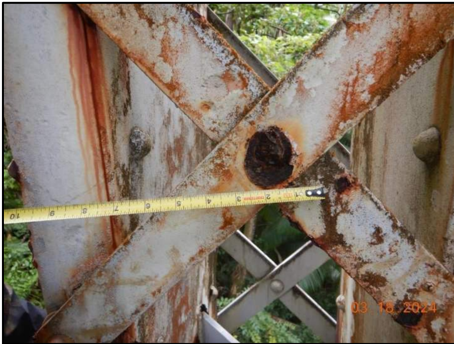
Photograph 16. Bent 2, Level 2, Column D, 7' from Level 1, east face, lacing bar, center rivet head, looking west. 100% section loss, CS3.
