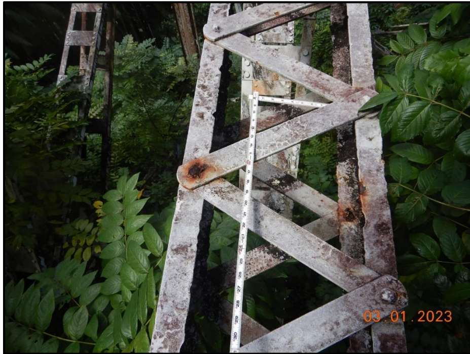
Photograph 73. Tower 2, Level 2, Column C, horizontal bracing, near mid-length slightly closer to Bent 2, looking north. Up to 3/16" deep pitting throughout with areas of knife-edging to original members of interior west face and isolated corrosion holes up to 1/2" diameter.
