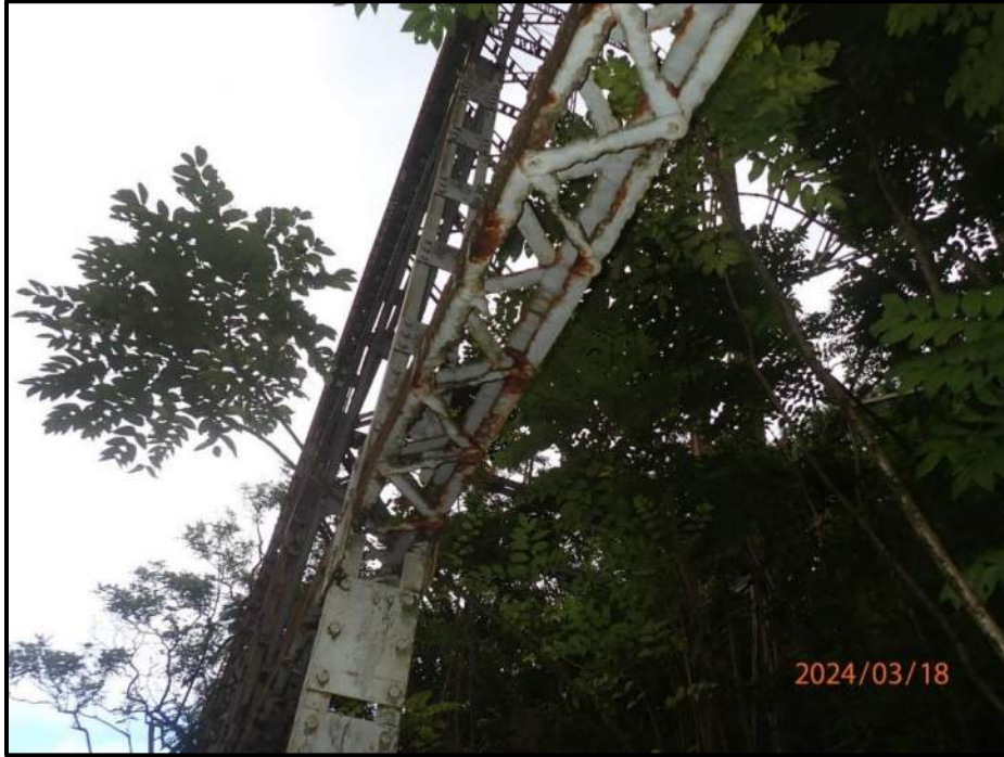
Photograph 81. Bent 5, Level 5, between Columns B and C, horizontal bracing, top and bottom lacing bars, looking east. Up to 100% section loss, CS3.
