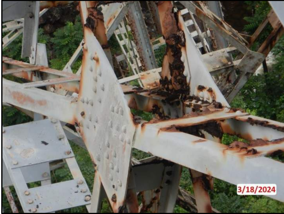
Photograph 27. Tower 2, Level 1, Column C, both center gusset plates, looking northeast. Pack rust at the incoming angles up to 1/2" thick; Laminar corrosion adjacent to angles throughout with up to 1" diameter x 100% section loss, CS3.
