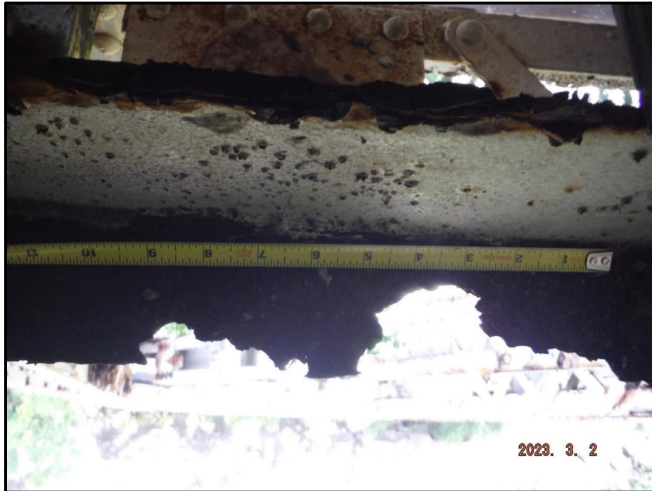
Photograph 27. Span 6, Bay 1 at Bent 5, adjacent to Girder 1, lower bracing (wind bracing), looking north. 100% section loss on bottom flange over 10" L x up to 1 1/2" deep.
