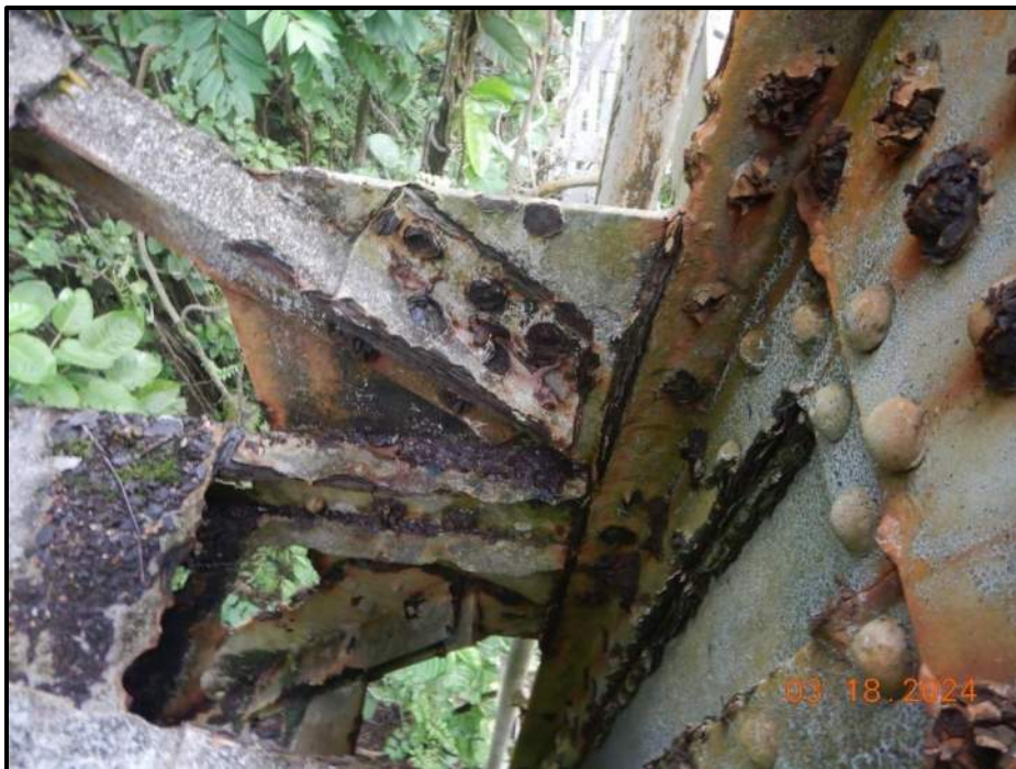
Photograph 110. Tower 4, Level 4, Column C, gusset plate at Bent 6, looking east. (9) of (18) rivet heads connecting the gusset plate to the column have 10% remaining on the inside face, CS3.
