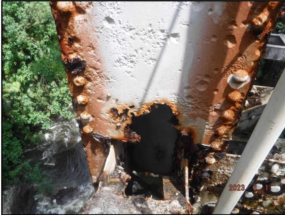
Photograph 116. Bent 5, Level 4, Column B, west batten plate, looking east. 9" diameter corrosion hole, CS3.
