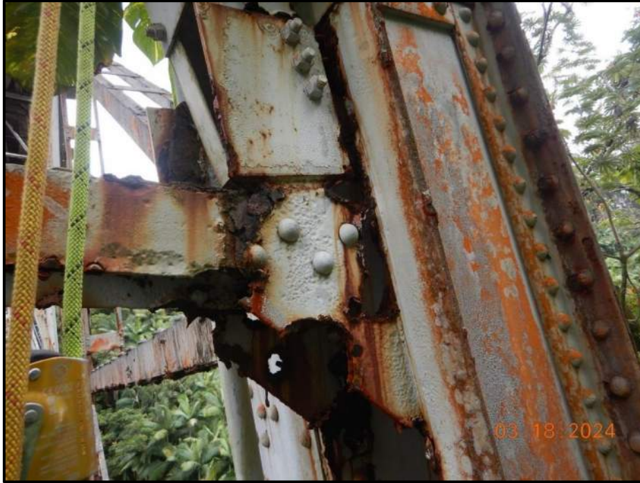
Photograph 117. Bent 7, Level 2, Column D, gusset plates, looking south. Corrosion, heavy laminar corrosion with diagonal lateral bracing corroded away and detached, CS4.
