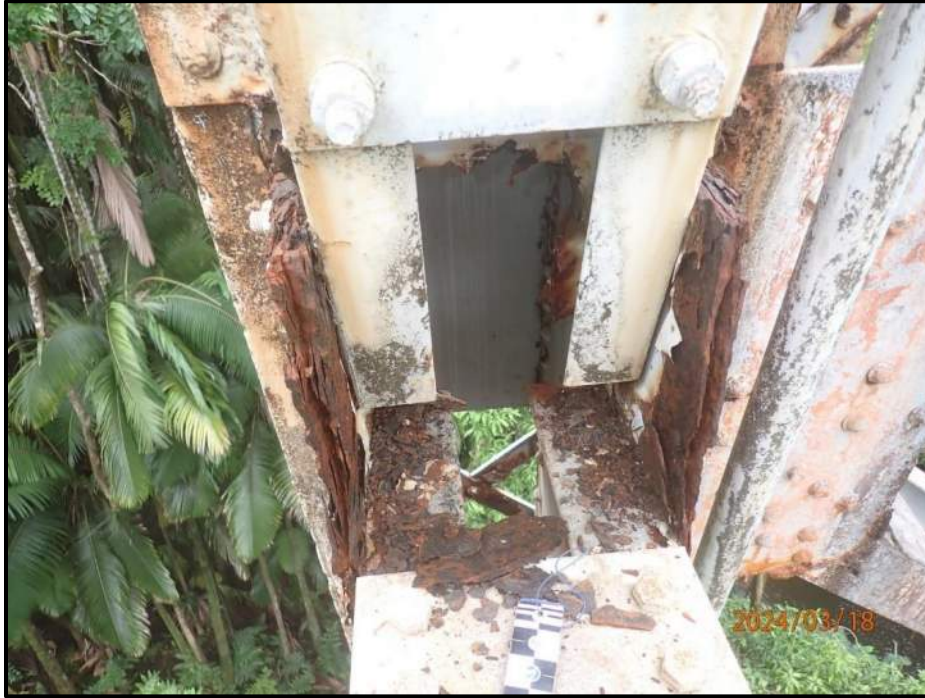
Photograph 67. Tower 3, Level 3, Column D, Bent 4 gusset plate, looking south. Heavy laminar corrosion with up to 50% section loss, CS3.
