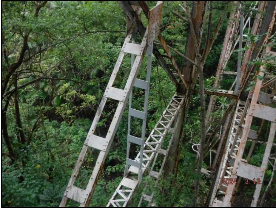
Photograph 103. Tower 4, Level 3, Column A, vertical bracing, looking southeast. Section loss, exterior leg with 80% loss. - Repaired. Top connection bolts of repaired section is not painted and exhibits surface corrosion, CS2.
