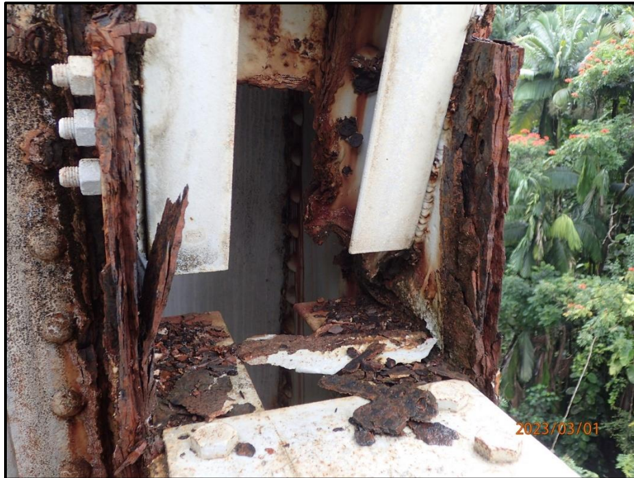
Photograph 114. Bent 5, Level 3, between Columns C and D, diagonal bracing, outboard angles, looking west. 10" L x up to Full Height section loss with adjacent corrosion holes, extreme deterioration up to 90% cross section reduction having no change from previous inspection, CS4.
