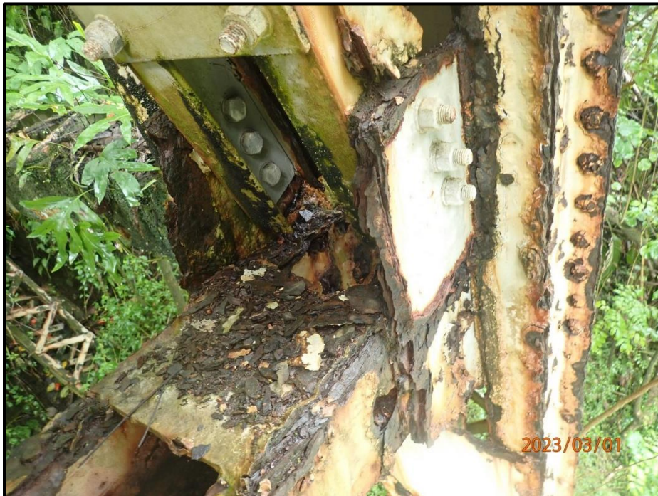
Photograph 129. Bent 6, Level 4, Column A, gusset plate at horizontal bracing, looking northeast. 75% section loss with corrosion holes, CS3.
