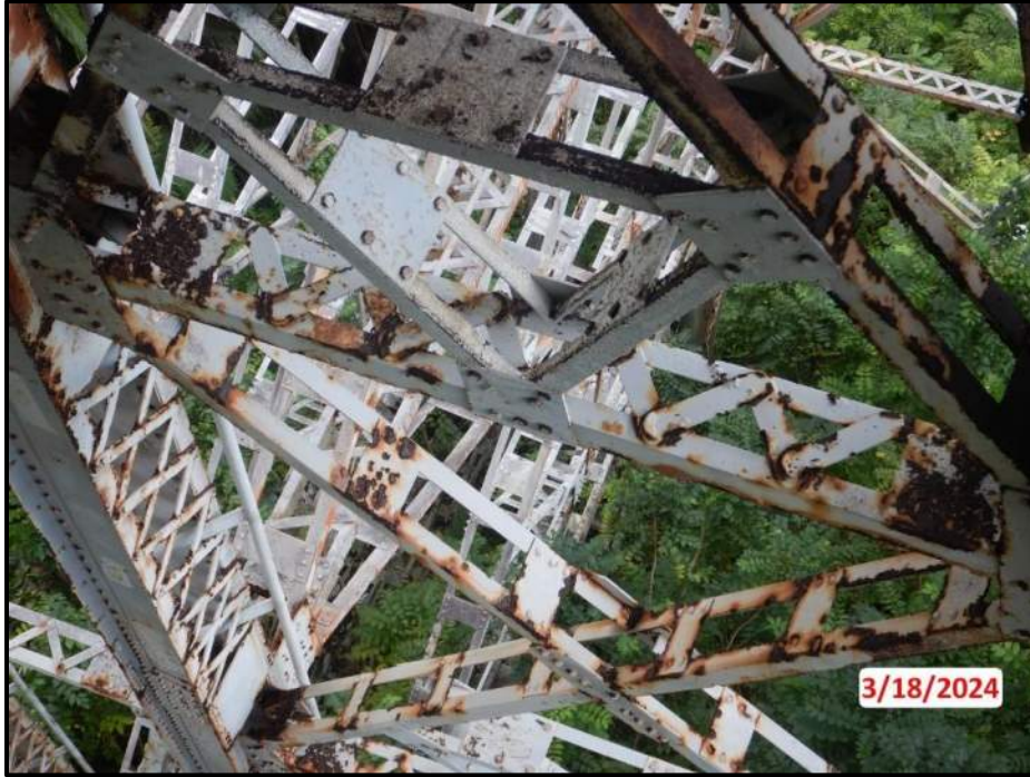
Photograph 13. Bent 2, Level 1, upper section, between Columns B and C, horizontal bracing, west face, lacing bars, looking north. (3) with 50% section loss and (1) with 90% section loss, CS3.
