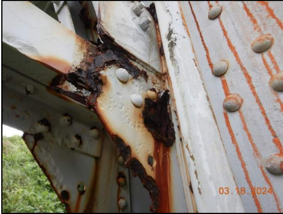
Photograph 15. Bent 2, Level 1, lower section, Column D, lower horizontal gusset plate, looking south. Laminar corrosion up to 100% section loss with knife edging, painted over pitting, and 4" corrosion hole, CS3.
