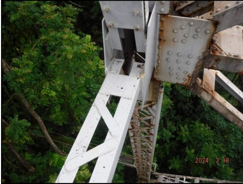
Photograph 115. Bent 7, Level 2, between Columns A and B, horizontal bracing and gusset plate at Column A, looking east. - Repaired and repair is in good condition.
