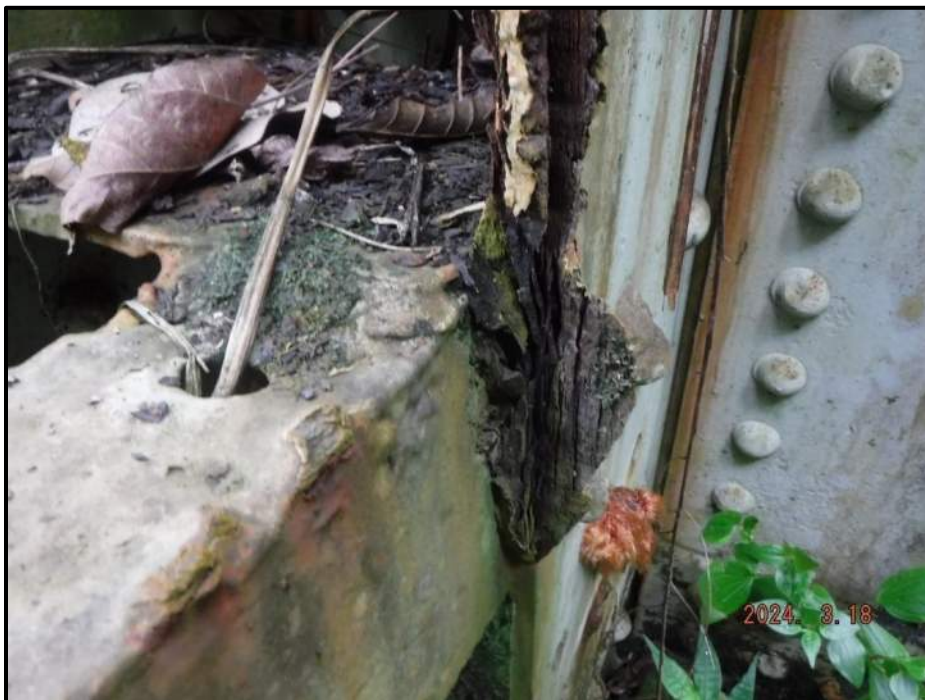
Photograph 20. Bent 2, Level 3, north of Column A, west gusset plate, looking south. Pack rust up to 1/4" thick, CS3.
