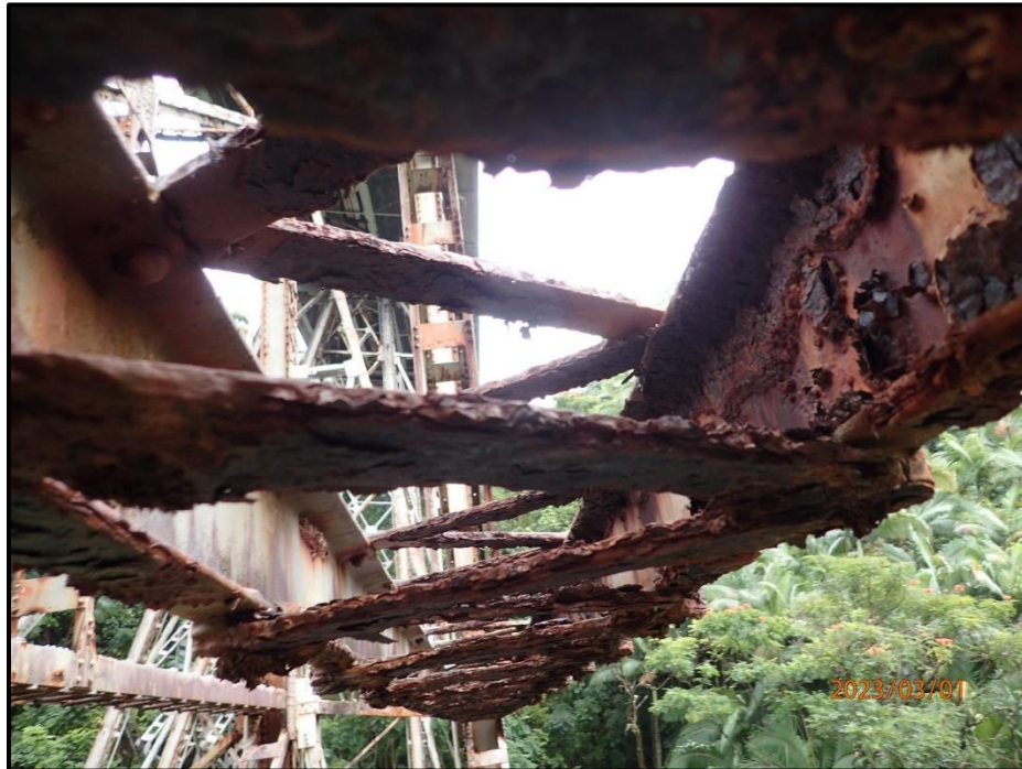
Photograph 103. Tower 3, Level 2, Column D, horizontal bracing, exterior channel side face, looking south. Heavy laminar corrosion, CS3.
