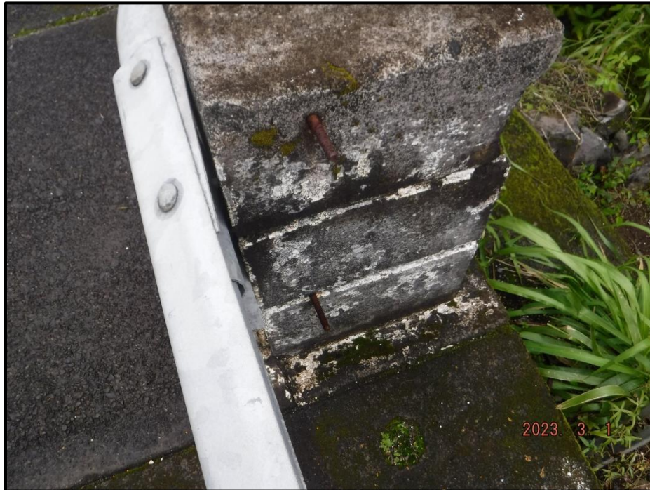
Photograph 53. East railing, south end, looking north. (2) reinforcing bars sticking out of concrete towards NB traffic.
