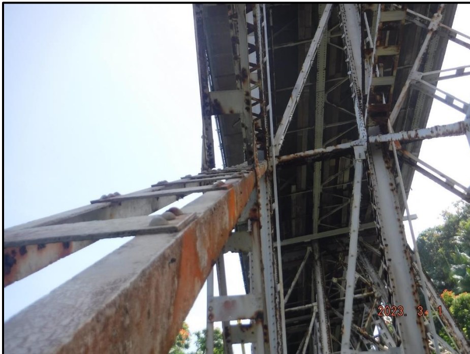
Photograph 96. Tower 3, Level 2, Column A, upper south to lower north diagonal bracing, looking south. Global distortion to the diagonal members within level, CS3.
