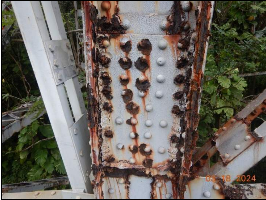
Photograph 89. Bent 6, Level 3, Column C, south face cover plate, looking north. 50% of rivet heads have up to 20% remaining section, CS3.
