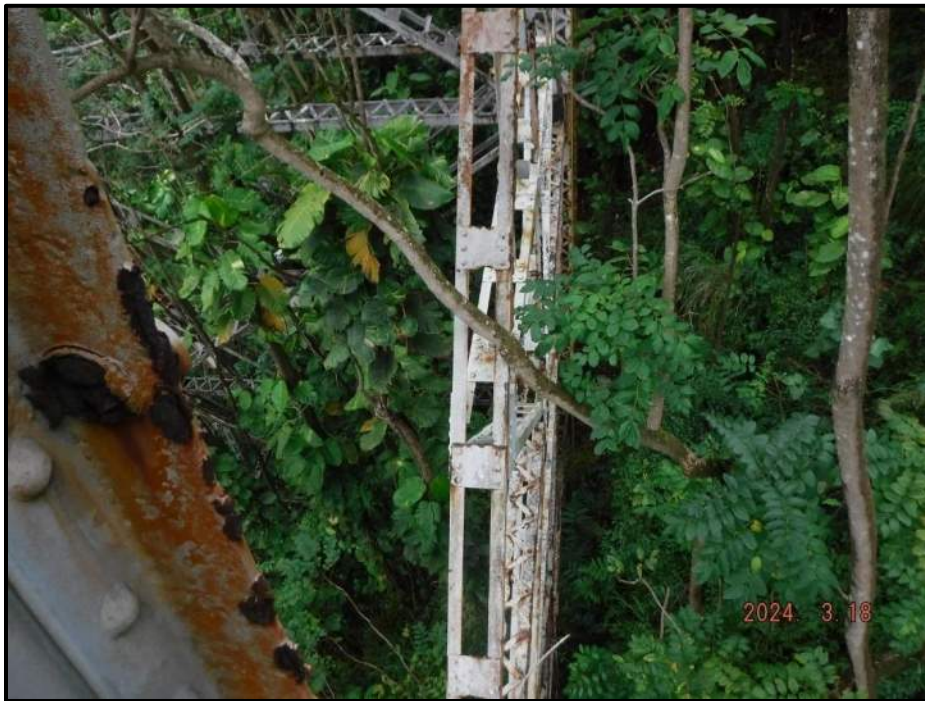
Photograph 118. Bent 7, Level 3, between Columns C and D, lower east diagonal, looking west. Tree growing against structure.
