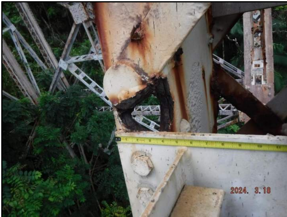
Photograph 40. Bent 3, Level 2, Column B, looking west. 2-1/2" diameter corrosion hole in southeast angle above horizontal brace connection, CS3.
