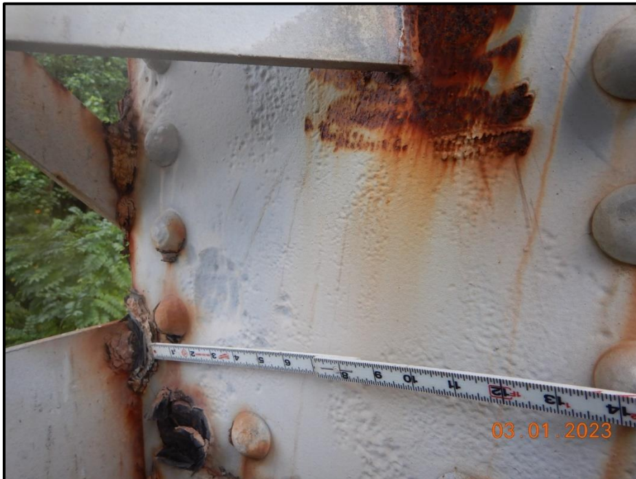
Photograph 62. Bent 2, Level 1, lower section, Column C, interior face of south web cover plate, looking southeast. Painted-over pitting up to 3" diameter x 1/4" deep, CS3.
