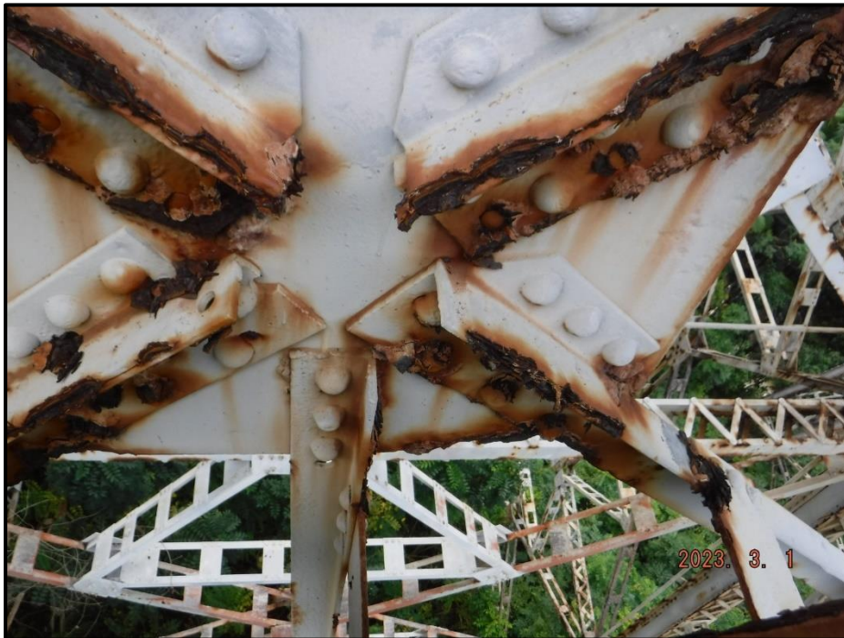
Photograph 68. Tower 2, Level 1, Column A, lower north diagonal bracing, east face of diagonal, interior center gusset plate, looking west. 9" W x 3" H area of 100% section loss and areas of laminar corrosion, CS3.
