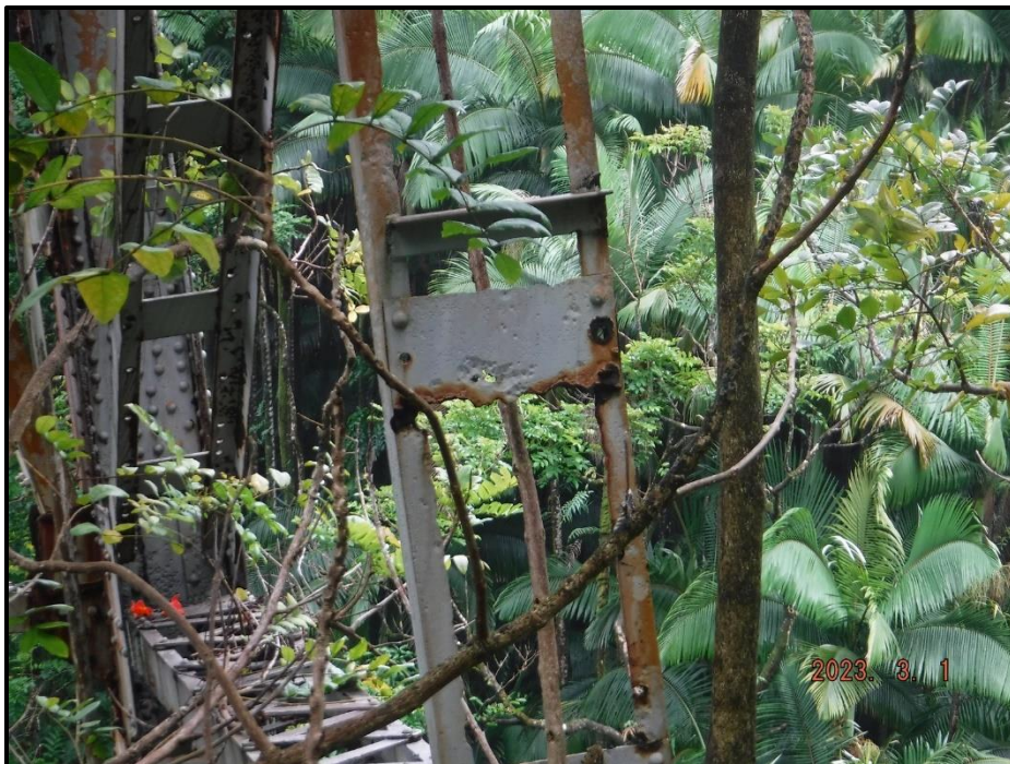
Photograph 139. Tower 4, Level 4, Column D, vertical bracing, looking north. Up to 1" H x full width area of 100% section loss across bottom edge of batten plate, CS3.
