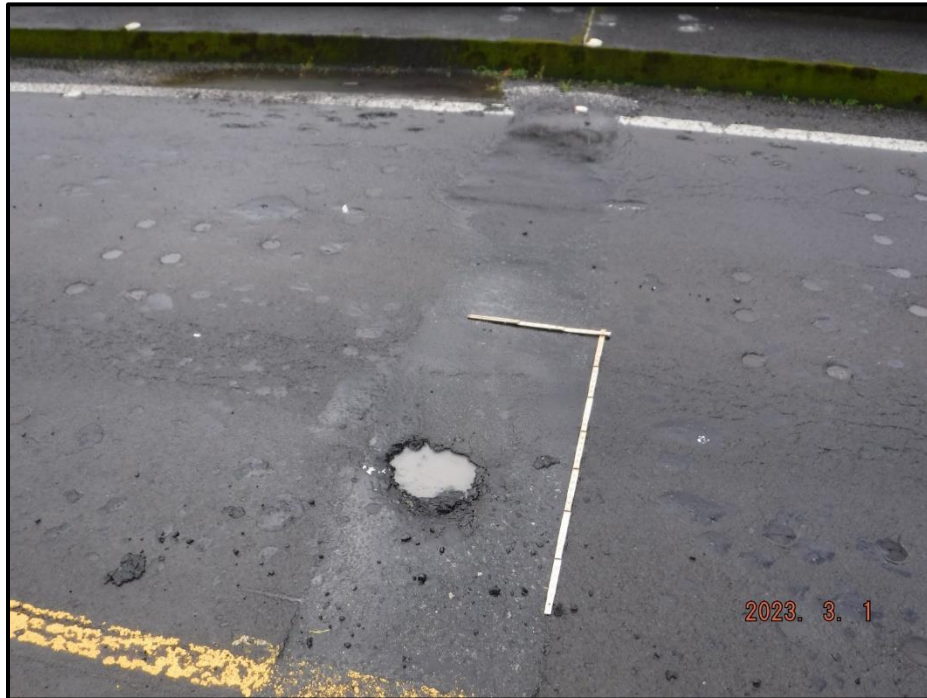
Photograph 19. Bent 5 Joint, SB lane, looking southwest. 2' L x 4' 5" W x 2" deep settled patch with a 11" L x 11" W x 1" deep spall within with exposure of deck and joint, CS3, CS4.
