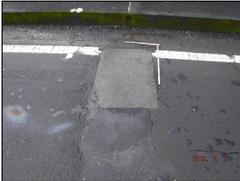
Photograph 51. Bent 7 Joint, SB lane, looking west. Previous cracked and settled patch has been re-patched.
