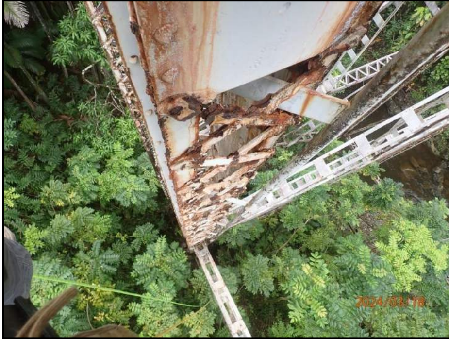
Photograph 55. Bent 4, Level 5, Column C, west face, (6) lacing bars, looking east. 100% section loss, CS3.
