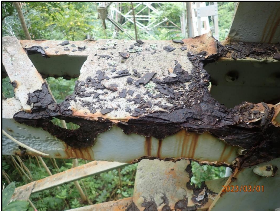
Photograph 63. Bent 2, Level 2, between Columns B and C, horizontal bracing near Column B, looking north. The bottom 1" of both angles have knife-edging to 100% section loss. There is an area of 90% section loss to the south angle, CS3.
