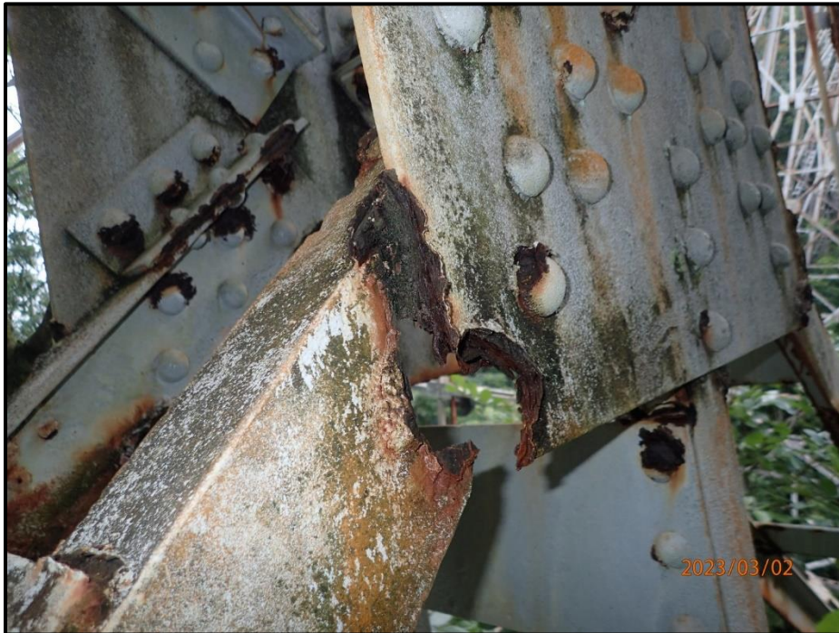
Photograph 138. Tower 4, Level 3, Column C, lower south diagonal bracing, looking east. West angle has 4" H x 2" L area of 100% section loss adjacent to the gusset plate, and the east angle has 1/4" loss in same location. Combined for 50% loss of member cross sectional area, CS4.
