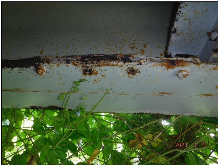
Photograph 32. Span 2, Girder 3, east face bottom flange, 5' north of Bent 1, looking west. (2) missing rivets in 1' L area of up to 1" thick pack rust, CS3.
