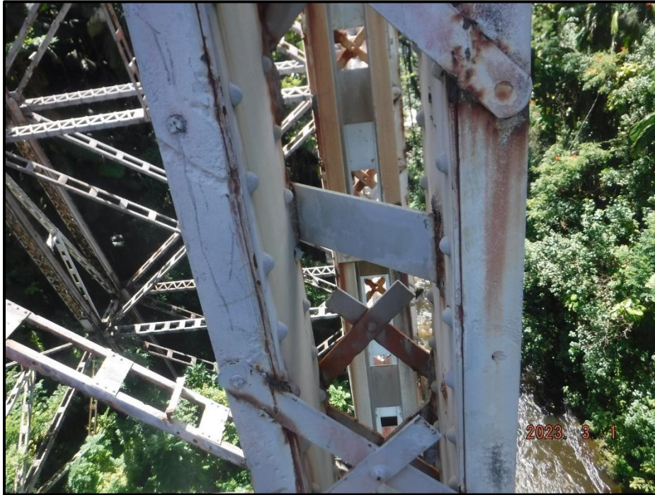
Photograph 112. Bent 5, Level 3, Column A, looking west. (9) lacing bars removed from column, CS3.
