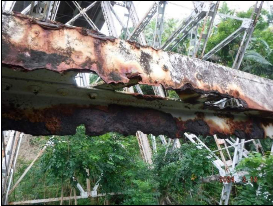
Photograph 41. Bent 3, Level 2, between Columns B and C, horizontal bracing, looking south. Knife-edging with up to 1-1/2" diameter corrosion holes on both flanges, CS3.
