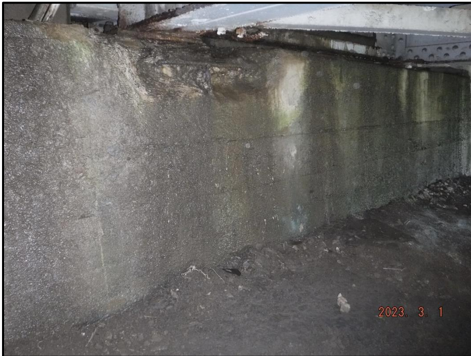
Photograph 44. North Abutment, west end of center section, looking northeast. Honeycombing, up to 2' H x 1' W x 1" deep, CS3.
