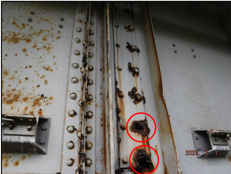
Photograph 40. Bent 3, Girder 4 web sliding plate, looking east. Heavy corrosion at the bolt slots and (2) missing bolts at the bottom, with a 2" H x 3" W area of 100% section loss, CS3.
