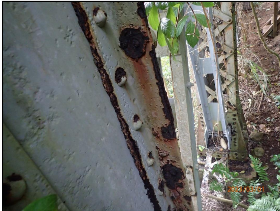
Photograph 57. Bent 1, Level 1, Column D, south face, looking east. Scattered rivets with up to 100% section loss, CS3.
