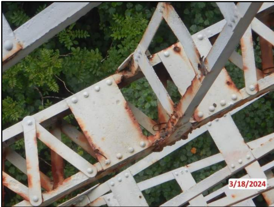
Photograph 56. Tower 3, Level 1, Column A, horizontal and vertical bracing gusset plate, looking southeast. Up to 85% section loss, full length x 2" H, CS3.
