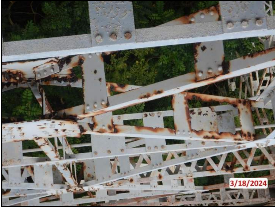
Photograph 23. Tower 2, Level 1, Column B, lower north diagonal bracing, both angle legs, looking west. Up to 1' L x 1-1/2" W isolated areas of 100% section loss along full member length, CS3.
