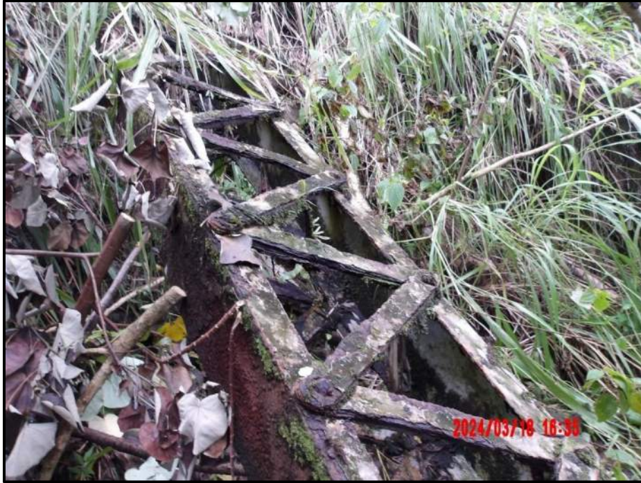
Photograph 125. Tower 5, Level 2, Column D, diagonal bracing, lacing bars, looking east. Heavy laminar corrosion (similar as Bent 8, Column D), CS3.
