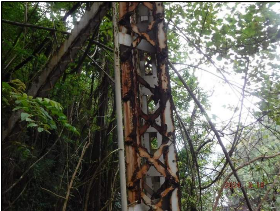
Photograph 94. Bent 6, Level 5, Column B, looking east. Almost all lacing bars on the west side of the column have 100% section loss; (6) bars remaining intact at time of inspection, CS4.
