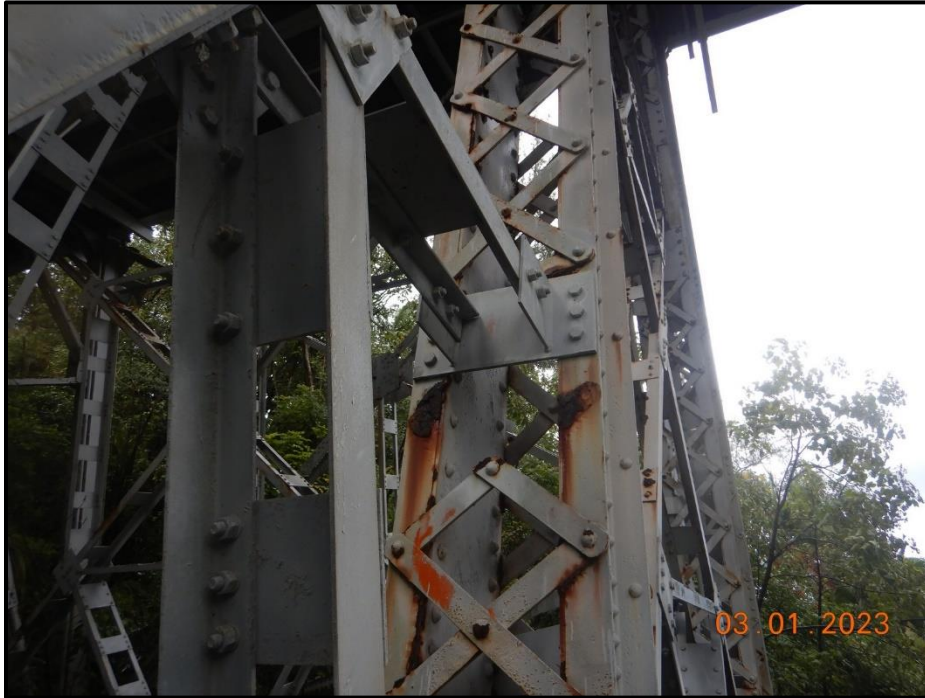
Photograph 152. Bent 8, Level 1, lower section, Column C, looking east. (2) lacing bars on west face have 100% section loss, CS3.
