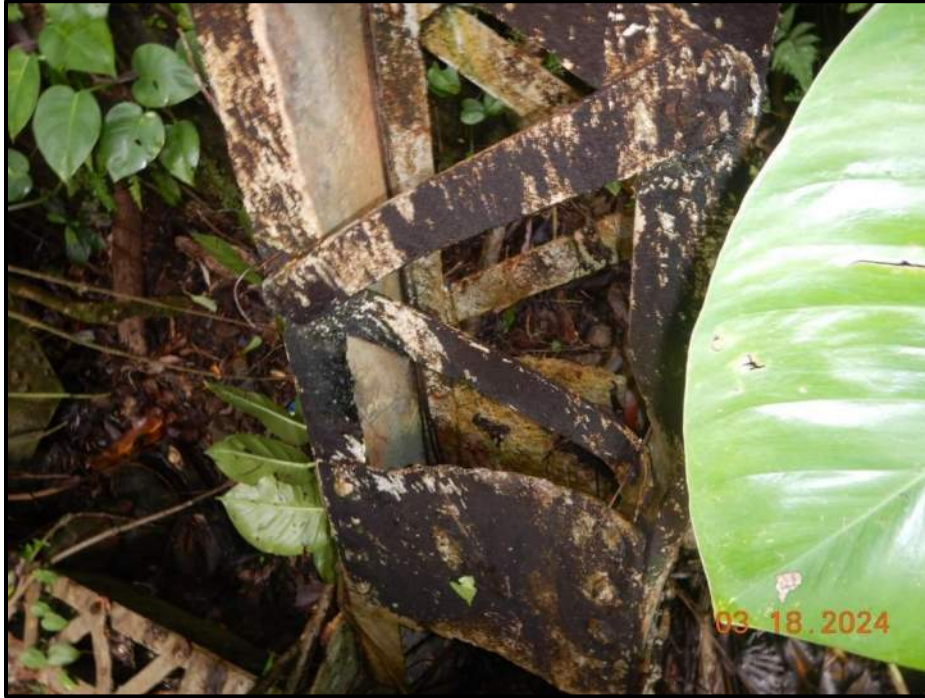
Photograph 113. Tower 4, Level 6, Column C, adjacent to Bent 6 pedestal, interior channel, looking north. 3" downward deformation over 1' 6" L, CS3.
