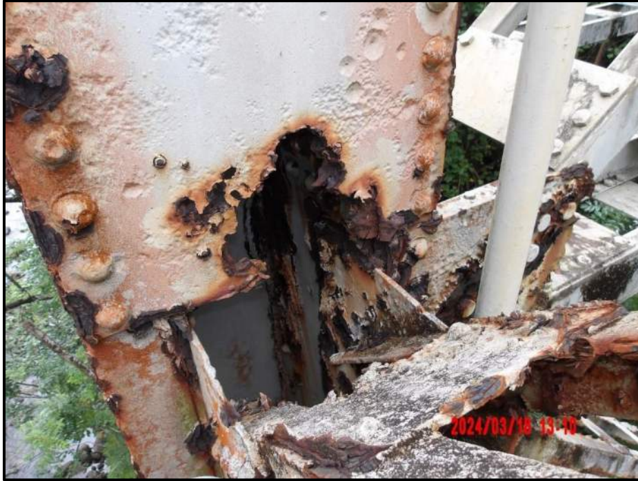
Photograph 79. Bent 5, Level 4, Column B, west cover plate, looking east. Corrosion hole, 9" diameter, CS3.
