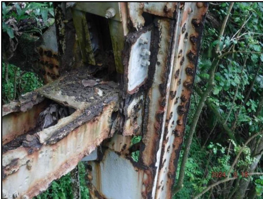
Photograph 96. Bent 6, Level 5, Column A, gusset plate at horizontal bracing, looking northeast. 75% section loss with corrosion holes, CS3.
