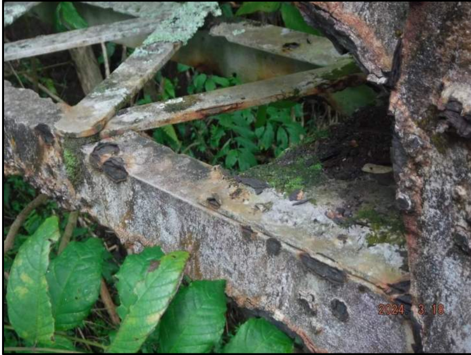
Photograph 25. Tower 2, Level 3, Column B, horizontal bracing, looking northeast. Numerous rivet heads with up to 100% section loss, CS3.
