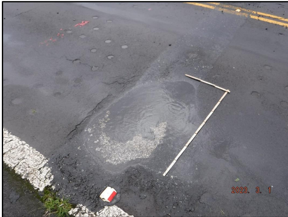
Photograph 18. Bent 5 Joint, NB lane, looking southwest. 2' 4" L x 4' W x 1/2" deep cracked and settled pothole with ponding water, CS3.
