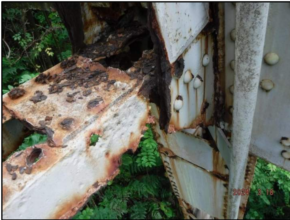
Photograph 120. Bent 7, Level 3, Column A, south horizontal bracing angle, looking northeast. 3" W x 4" H corrosion hole in vertical angle, CS3.
