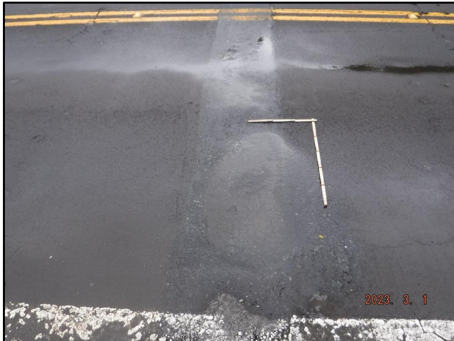
Photograph 22. Bent 9 Joint, NB right wheel line, looking west. Cracked and settled potholes with ponding water, CS3.
