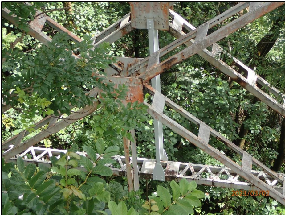
Photograph 135. Tower 4, Level 3, Column A, vertical bracing, looking east. Exterior leg with 80% section loss has been replaced.
