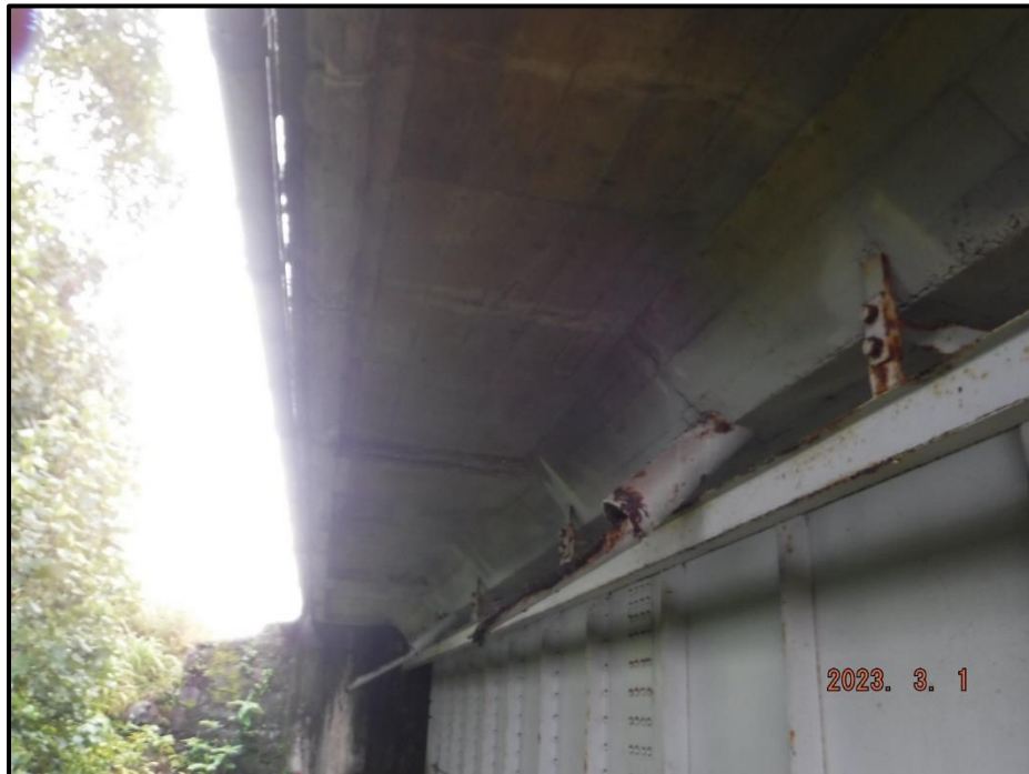
Photograph 24. Span 1, underside of deck, east overhang, 5' south of Bent 1, looking south. Transverse cracking with efflorescence throughout, typically 3'-4' apart x up to 1/8" W, CS3.
