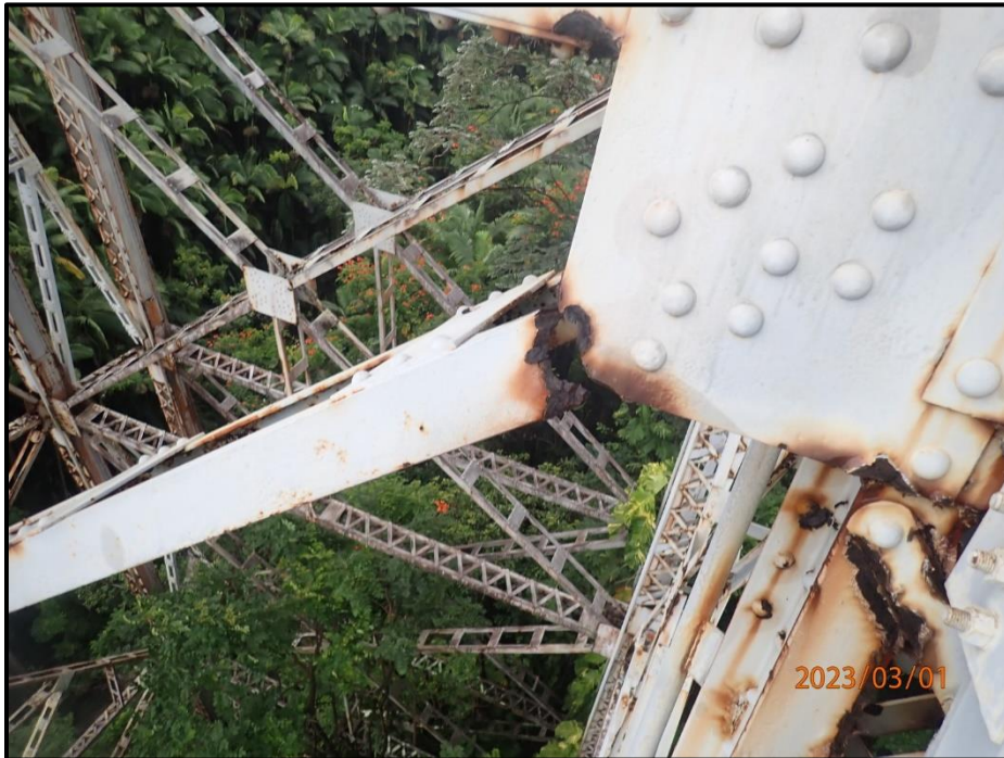
Photograph 134. Tower 4, Level 2, Column B, upper north diagonal bracing, looking west. Exterior angle of diagonal has 100% section loss to vertical leg, CS3.
