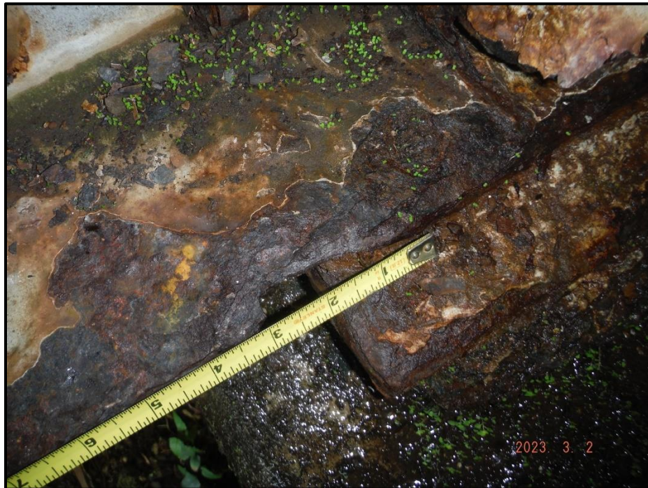
Photograph 38. Span 10, Girder 1, east face at North Abutment, looking west. 3" L x 1/2" W area of 100% section loss, CS3.
