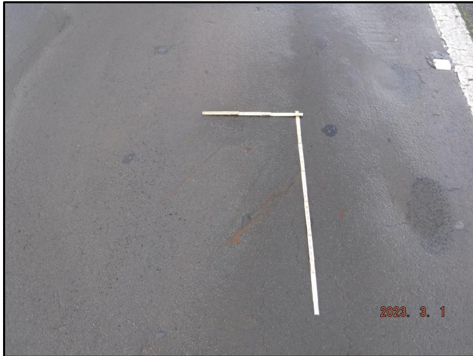
Photograph 17. Span 4, NB Lane, 20' north of Bent 3, looking north. 3' L x 3' W area of gouges (largest is 1' 1" L x 2' W x 1/2" deep), CS3.
