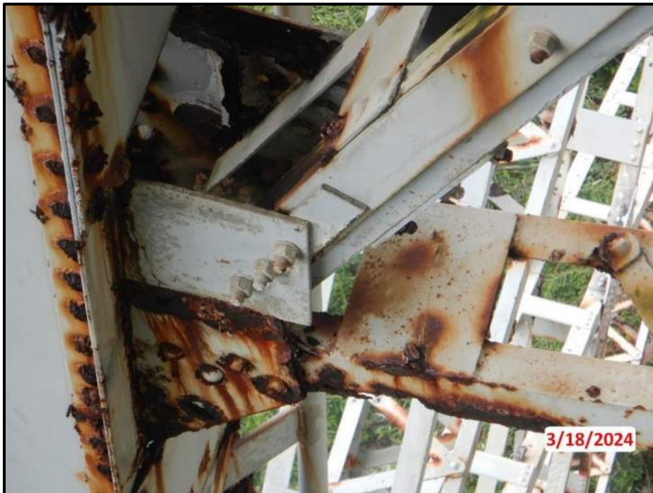
Photograph 114. Bent 7, Level 1, upper section, Column A, gusset plate, looking south. (2) corrosion holes up to 1" diameter, CS3.
