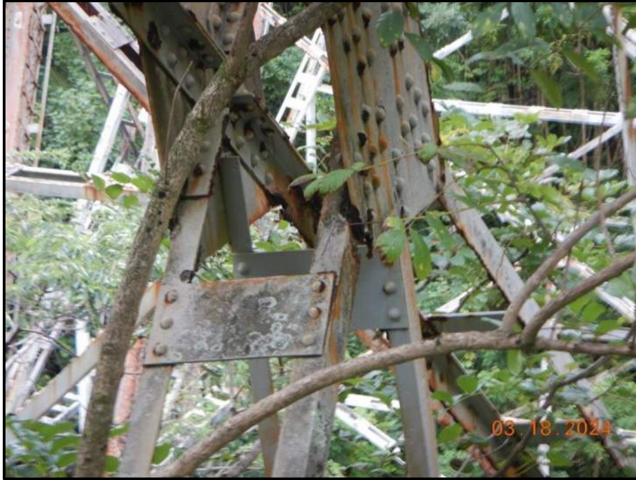
Photograph 109. Tower 4, Level 3, Column C, lower north diagonal bracing, looking southeast. West angle has 4" H x 2" L area of 100% section loss adjacent to the gusset plate, and the east angle has 1/4" loss in same location. Combined for 50% loss of member cross sectional area, CS4.
