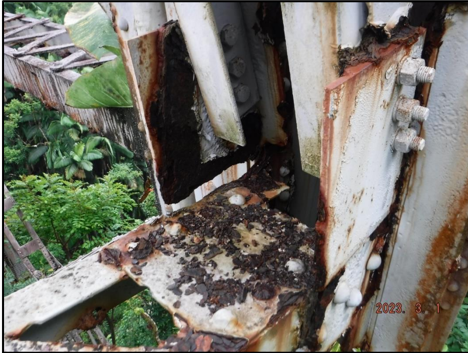
Photograph 148. Bent 7, Level 2, Column D, gusset plates, looking south. Corrosion, heavy laminar corrosion with diagonal lateral bracing corroded away and detached, CS4.
