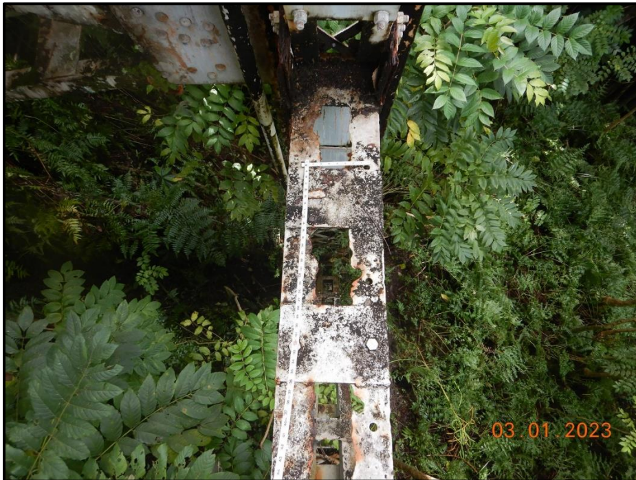
Photograph 80. Bent 3, Level 3, between Columns C and D, horizontal bracing, looking west. Knife-edging and multiple corrosion holes up to 2" diameter across full member length, CS3.
