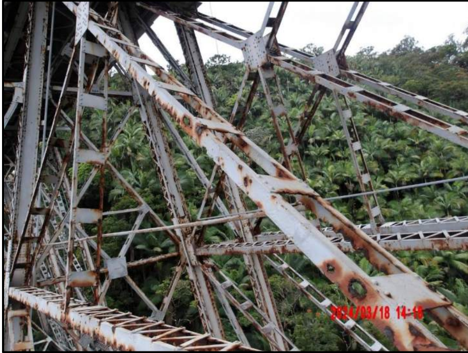
Photograph 59. Tower 3, Level 1, Column B, lower north diagonal bracing, looking southwest. Worst case is a 4" diameter corrosion hole near center gusset plate. Approximately 40% loss in cross sectional area, CS3.
