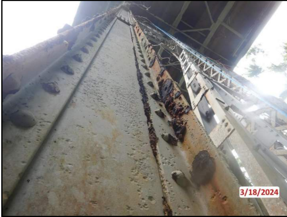
Photograph 11. Bent 1, Level 1, Column D, south face, looking north. Scattered rivets with up to 100% section loss, CS3.
