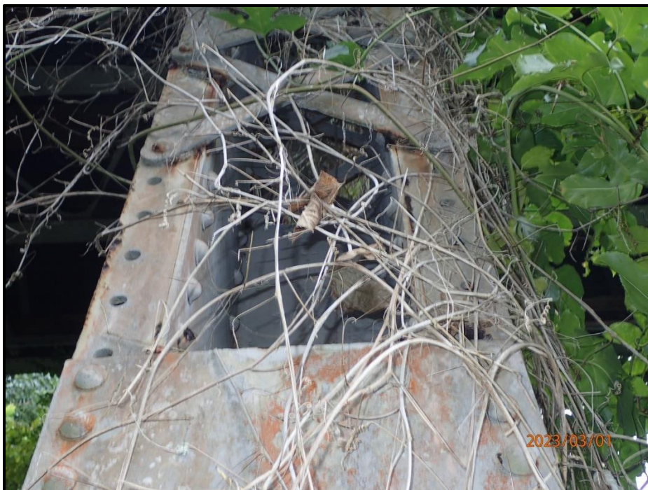
Photograph 56. Bent 1, Level 1, Column D, east face, near mid height horizontal, looking west. Missing batten plate, CS3.
