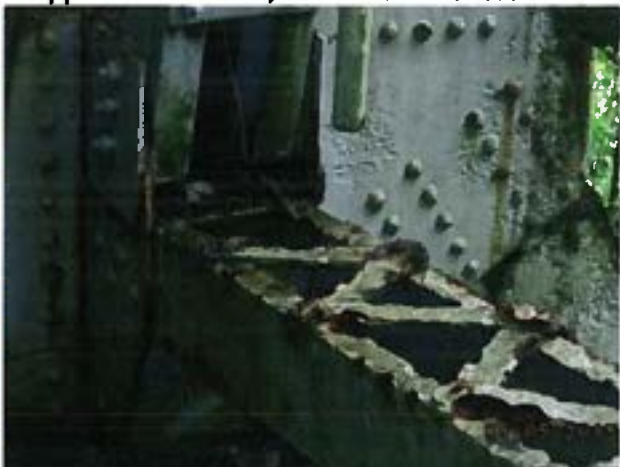
Bottom of bent 7 outlet end, column brace plates and lacings has corrossions.
