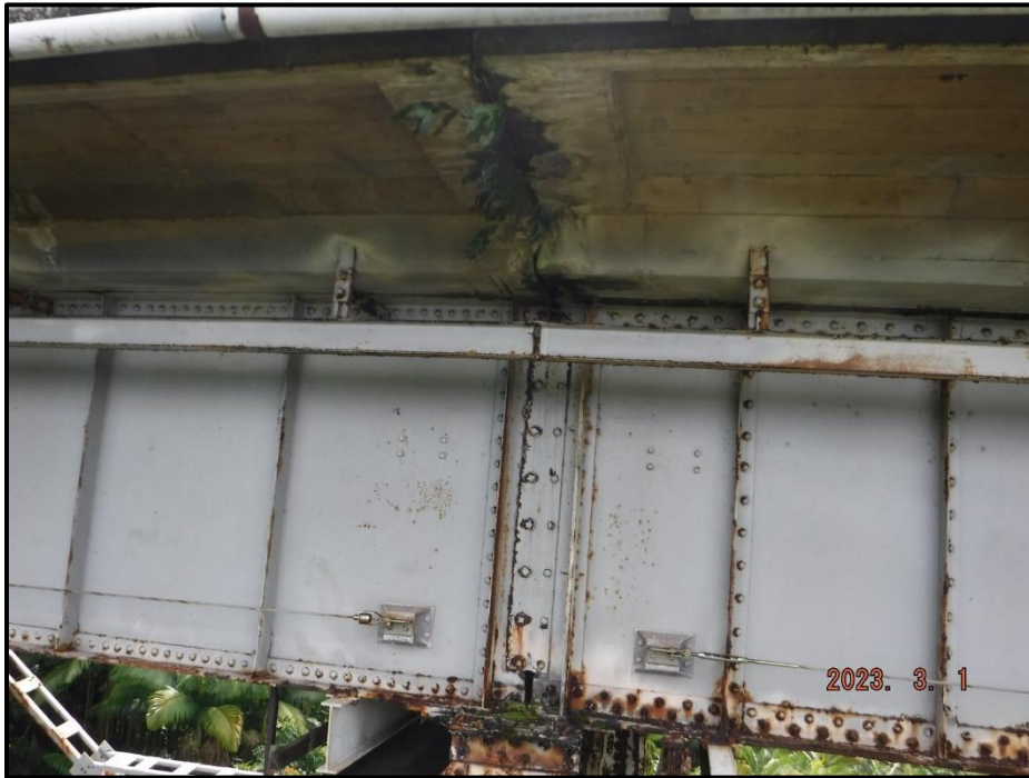
Photograph 45. Bent 3, center joint, looking west. Vegetation growth into the joint from the underdeck at the east overhang.
