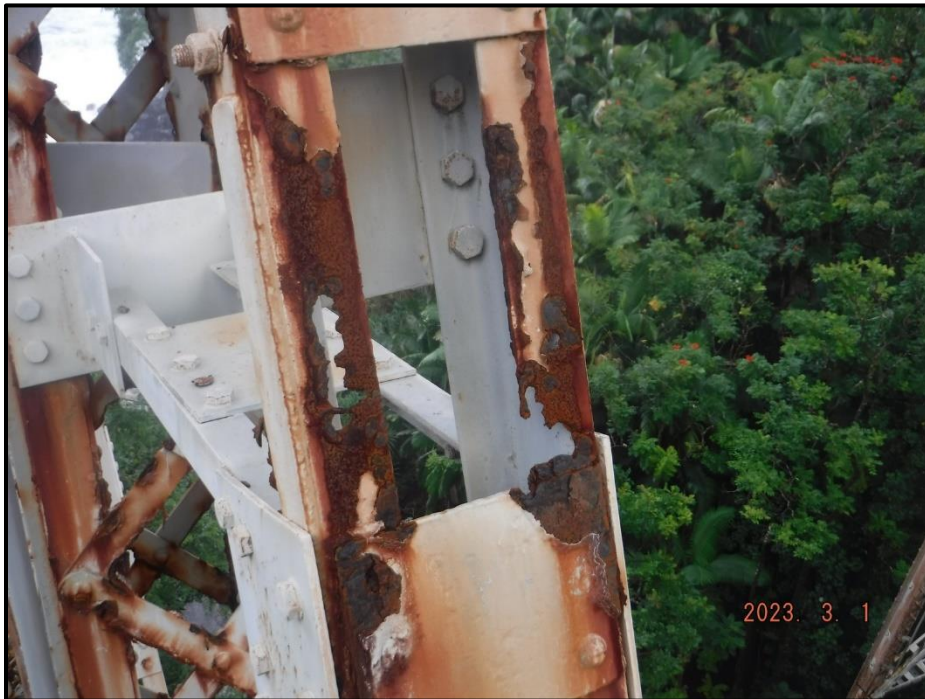
Photograph 123. Bent 6, Level 2, between Columns C and D, near mid-length of longest diagonal bracing, outer flanges, looking southeast. Up to 5" long corrosion holes, CS3.
