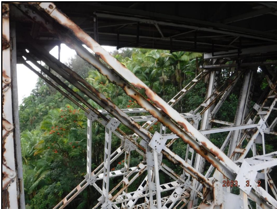
Photograph 72. Tower 2, Level 1, Column D, upper north diagonal bracing, near Bent 3, looking east. Heavy knife-edging and 6" L x 2" H corrosion holes, CS3.
