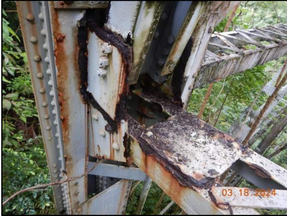
Photograph 19. Bent 2, Level 2, east of Column D, horizontal and diagonal bracing gusset plates, looking northwest. Typical heavy laminar corrosion and knife edging, CS3.
