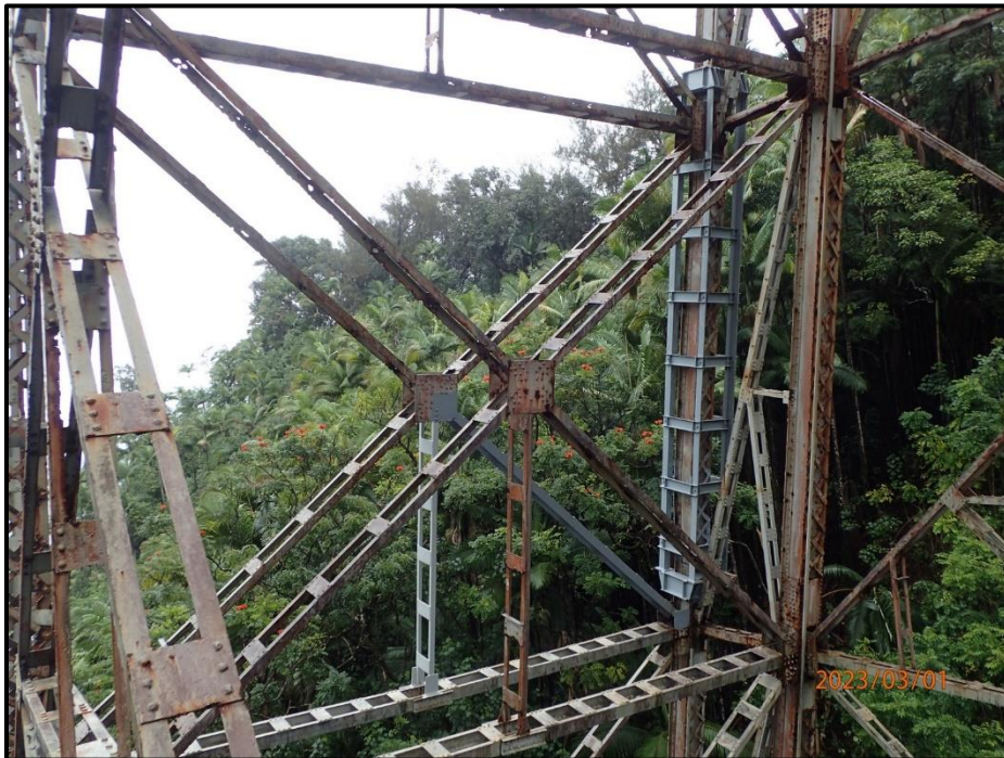
Photograph 98. Tower 3, Level 3, Column A, lower south diagonal, and vertical bracing, looking southeast. Repaired.
